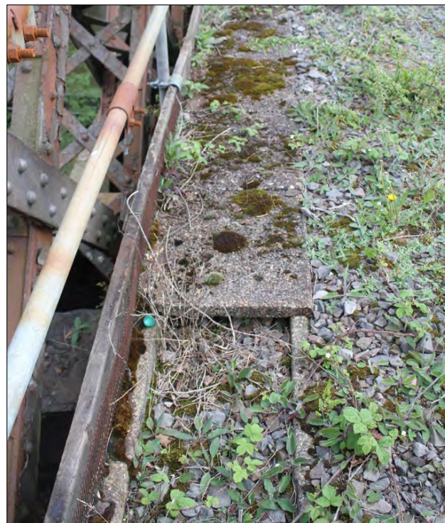
Concrete ducting for electric cabling
