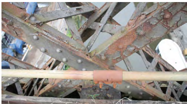
Steel fishplate with angled head showing thinner section and less corroded rivets
