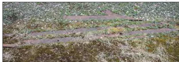
Broken fragments of lattice bars on the deck of the viaduct
