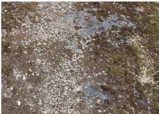
Exposed bitumen on the deck
