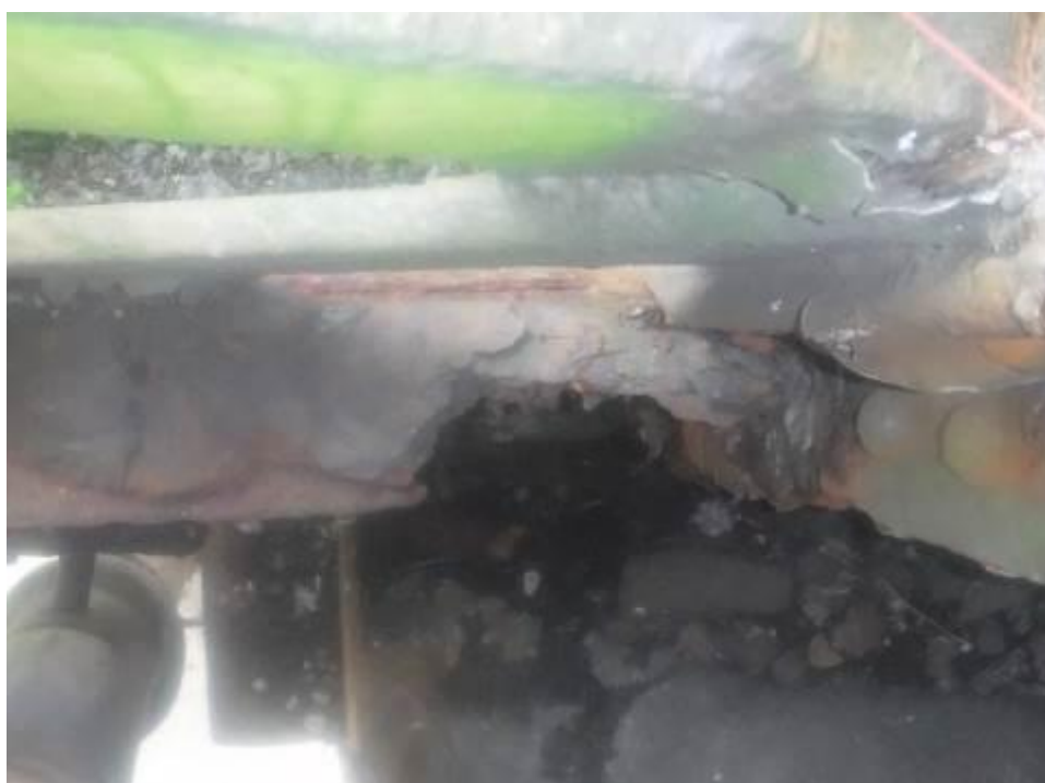
Photograph 130: Loss of thickness & section to bottom boom, top flange of south truss of span 4
