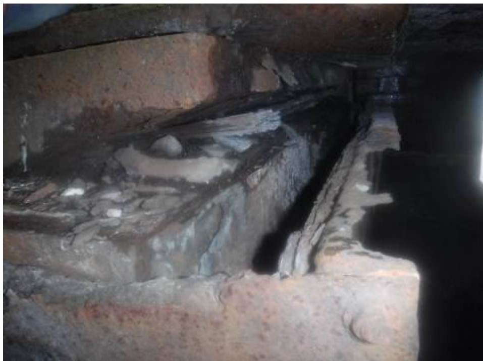
Photograph 25: Loss of thickness & loss of section to south bearing of west abutment
