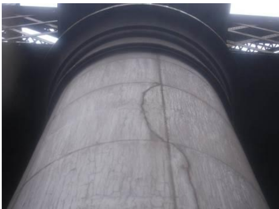
Photograph 66: Vertical & diagonal fractures to north column of pier 4
