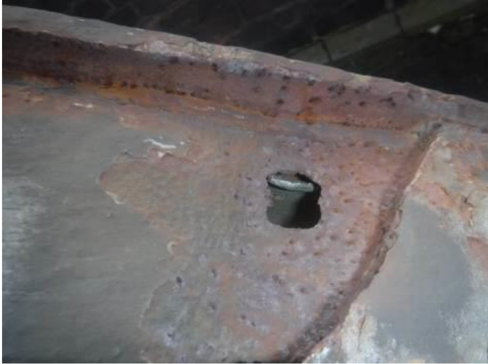
Photograph 151: Loss of section to bottom boom, bottom flange of south truss of span 6
