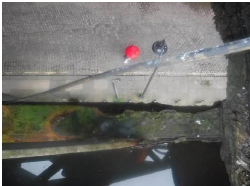
Photograph 103: Loss of section to bottom boom, top flange to north truss of span 2
