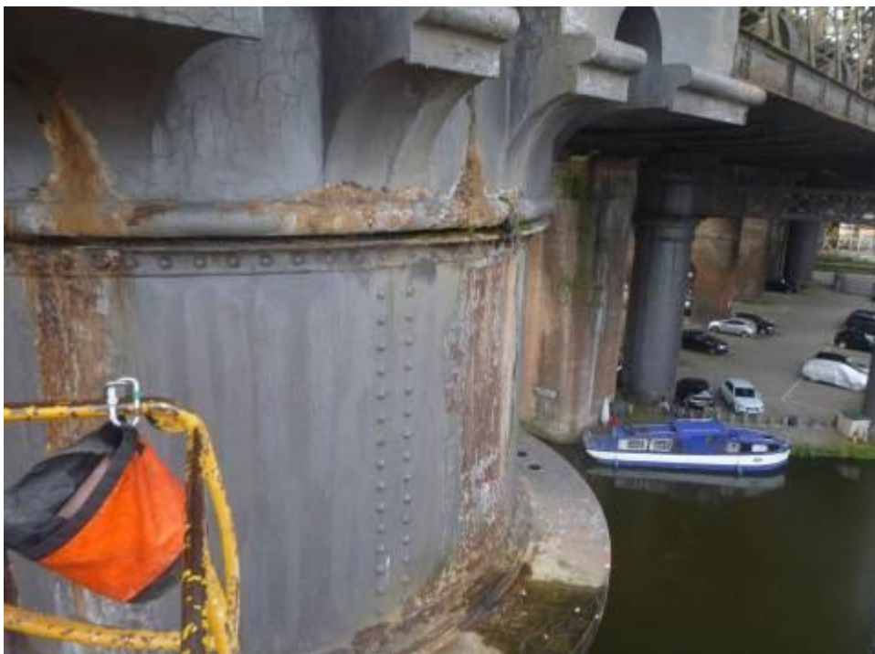
Photograph 68: Area of seepage & loss of thickness to north column of pier 4
