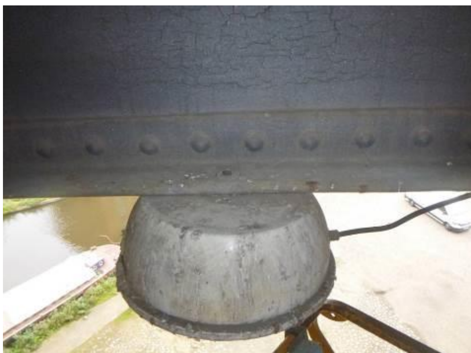
Photograph 198: Missing nut to fixing of lighting junction of soffit of span 4
