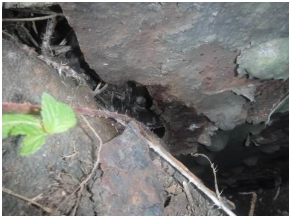
Photograph 115: Loss of section to end plate flange of north truss of span 3
