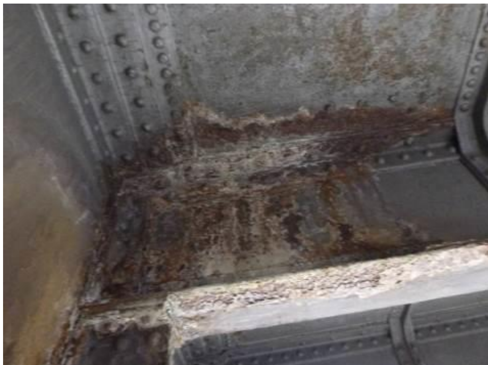
Photograph 197: Loss of thickness & pitting to MGI4 of soffit of span 4
