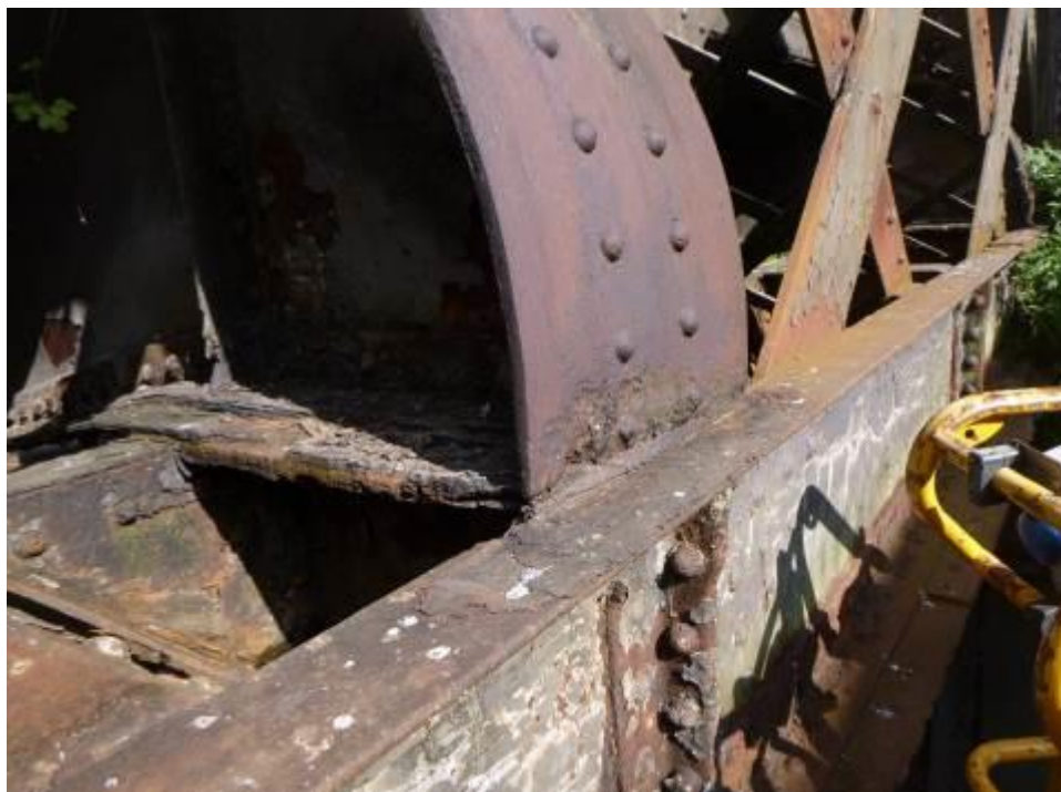
Photograph 181: Loss of thickness to T18 of soffit of span 2
