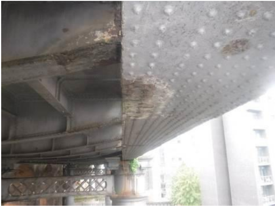
Photograph 205: Loss of thickness to MGE1 of soffit of span 5
