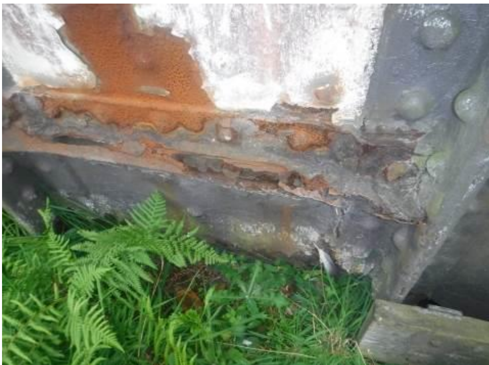
Photograph 150: Loss of section to end plate stiffener of south truss of span 6
