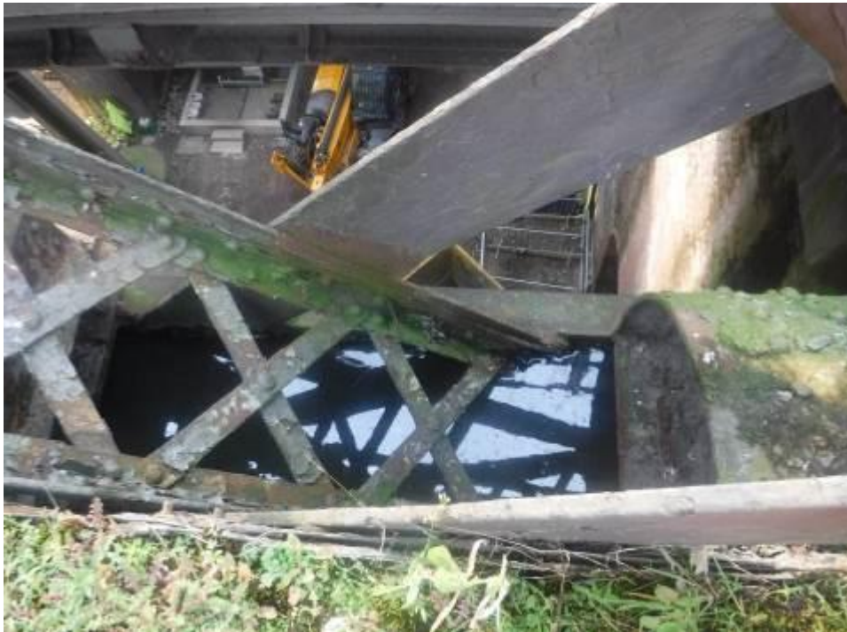
Photograph 167: Typical flooding to bottom boom of south truss of span 8
