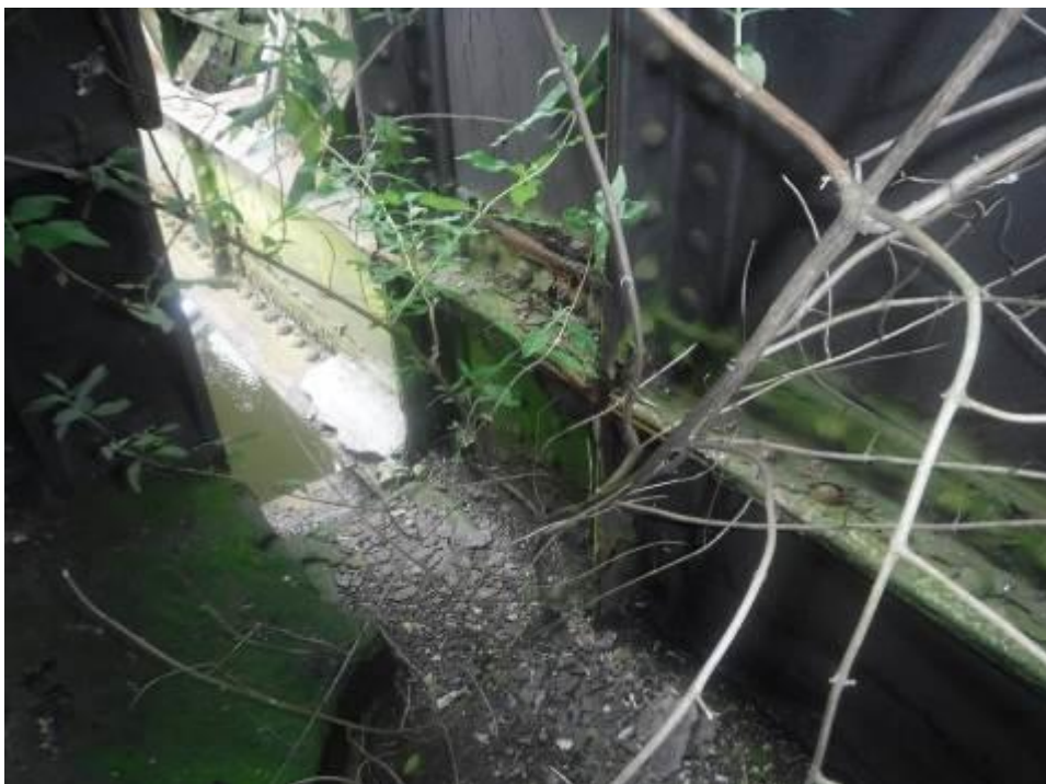
Photograph 142: Sapling growth to end beam void of south truss of span 5
