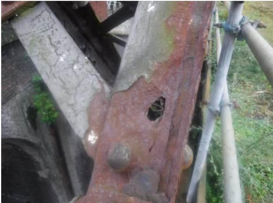
Photograph 109: Loss of section to diagonal bracing of south truss of span 2
