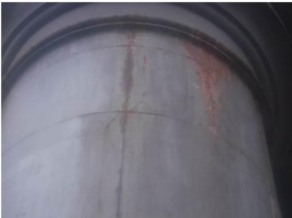
Photograph 78: Vertical fracture to north column of pier 5
