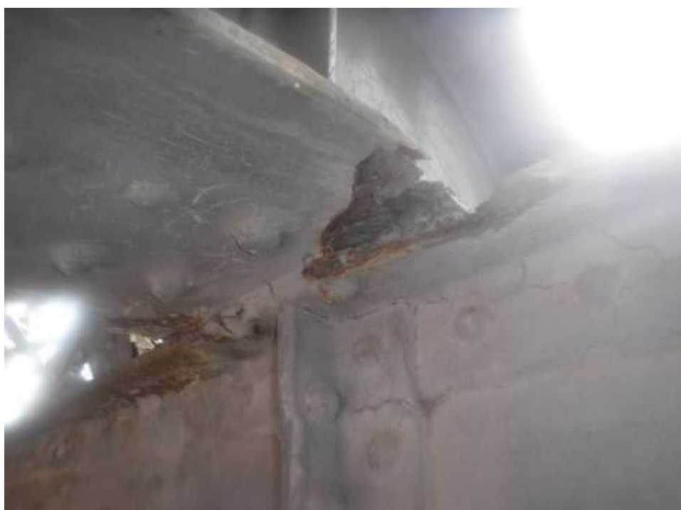
Photograph 220: Loss of section to T80 of soffit of span 8
