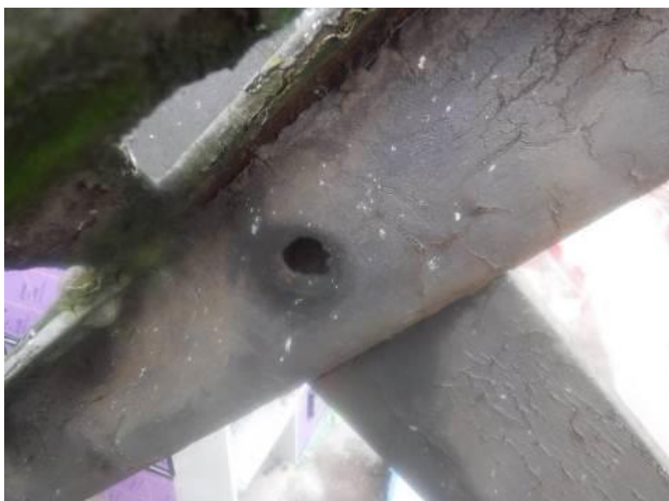
Photograph 164: Missing rivet to diagonal bracing of north truss of span 8
