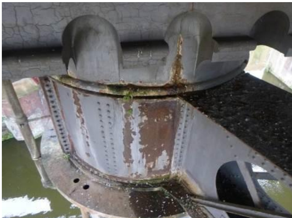
Photograph 70: Area of seepage & loss of thickness to south column of pier 4
