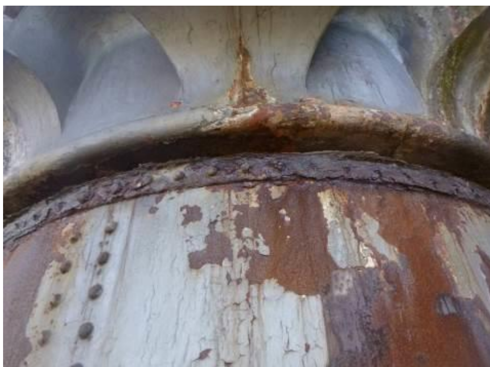
Photograph 40: Area of loss of section to north column of pier 1
