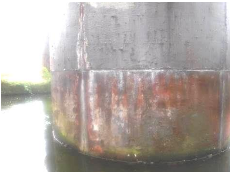
Photograph 60: Area of loss of thickness to south column of pier 3
