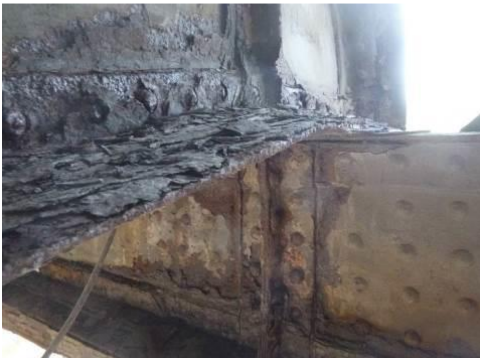
Photograph 188: Loss of thickness & pitting to T31 of soffit of span 3
