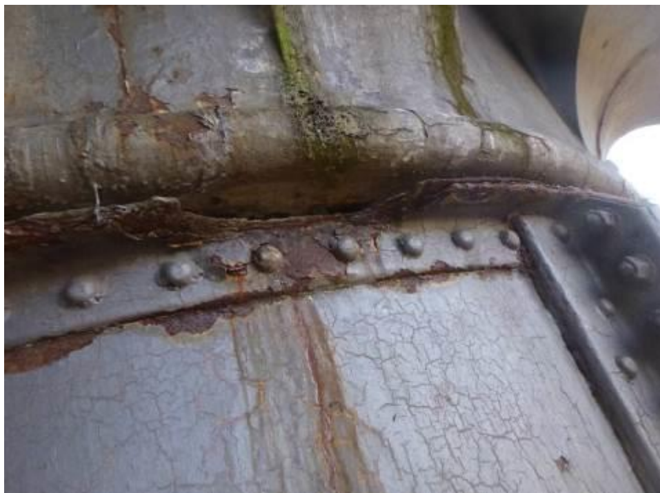
Photograph 49: Area of loss of section to upper angle of north column of pier 2
