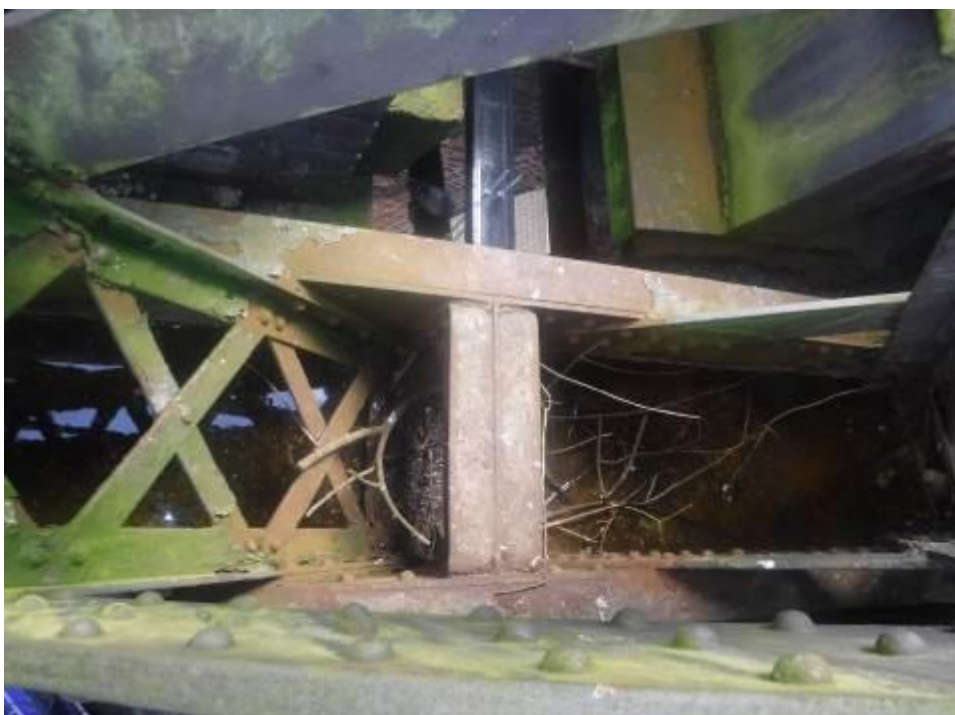
Photograph 140: Typical pooling & debris to bottom boom of south truss of span 5
