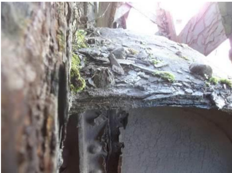
Photograph 214: Loss of thickness to T64 of soffit of span 7
