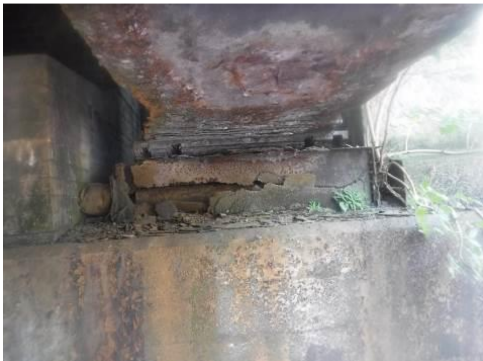
Photograph 21: Loss of thickness & loss of section to north bearing of west abutment
