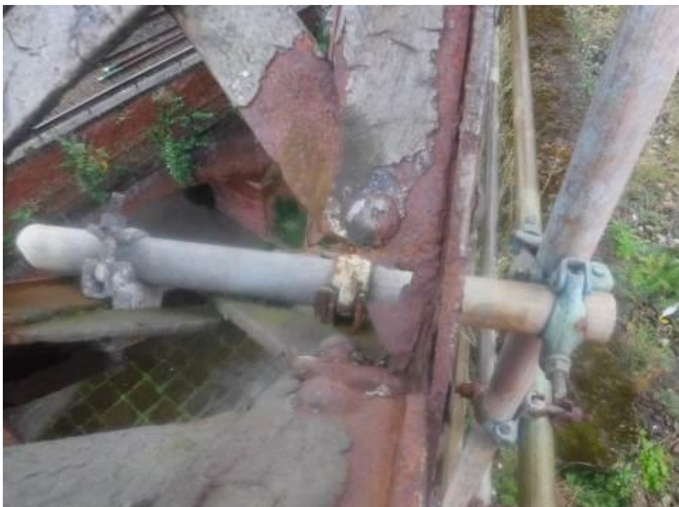
Photograph 100: Loss of section to diagonal member of north truss of span 2
