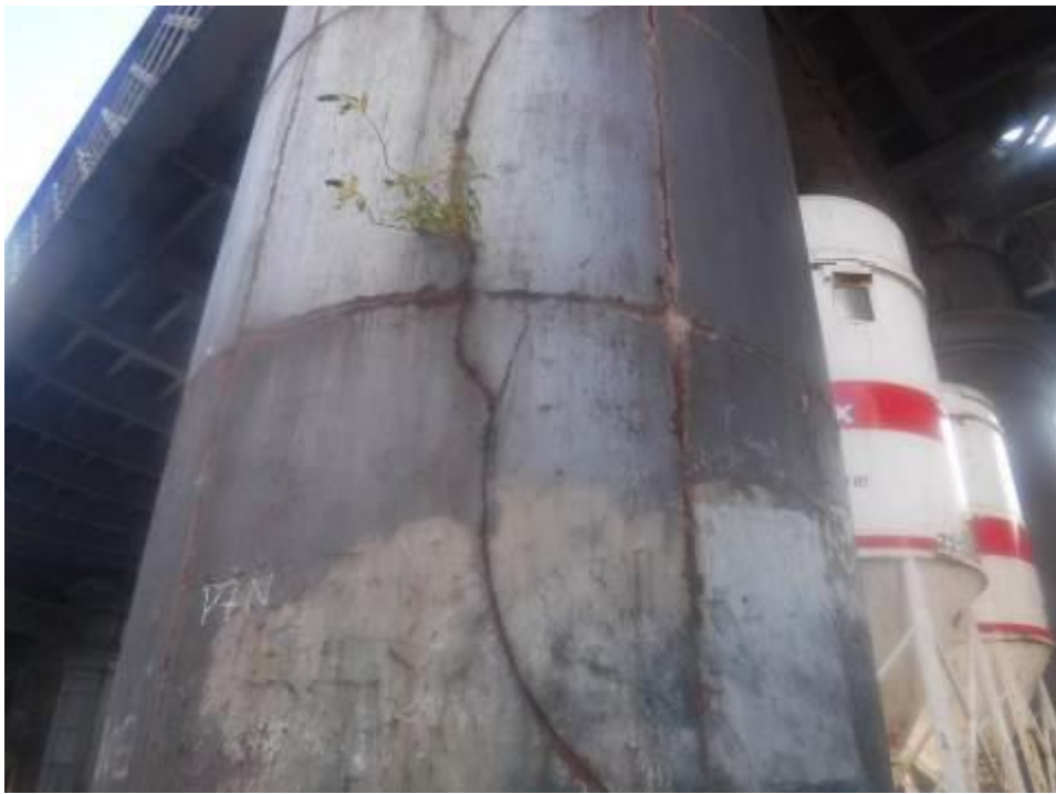
Photograph 85: Vertical branched fracture & buddleia growth to north column of pier 7
