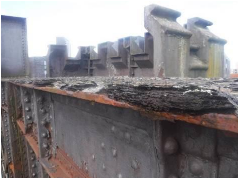
Photograph 137: Loss of thickness to top boom, top flange of north truss of span 5
