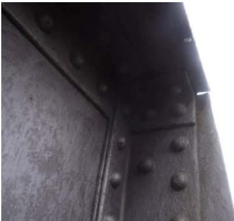
Photograph 178: Loss of section to upper transverse steelwork T27
