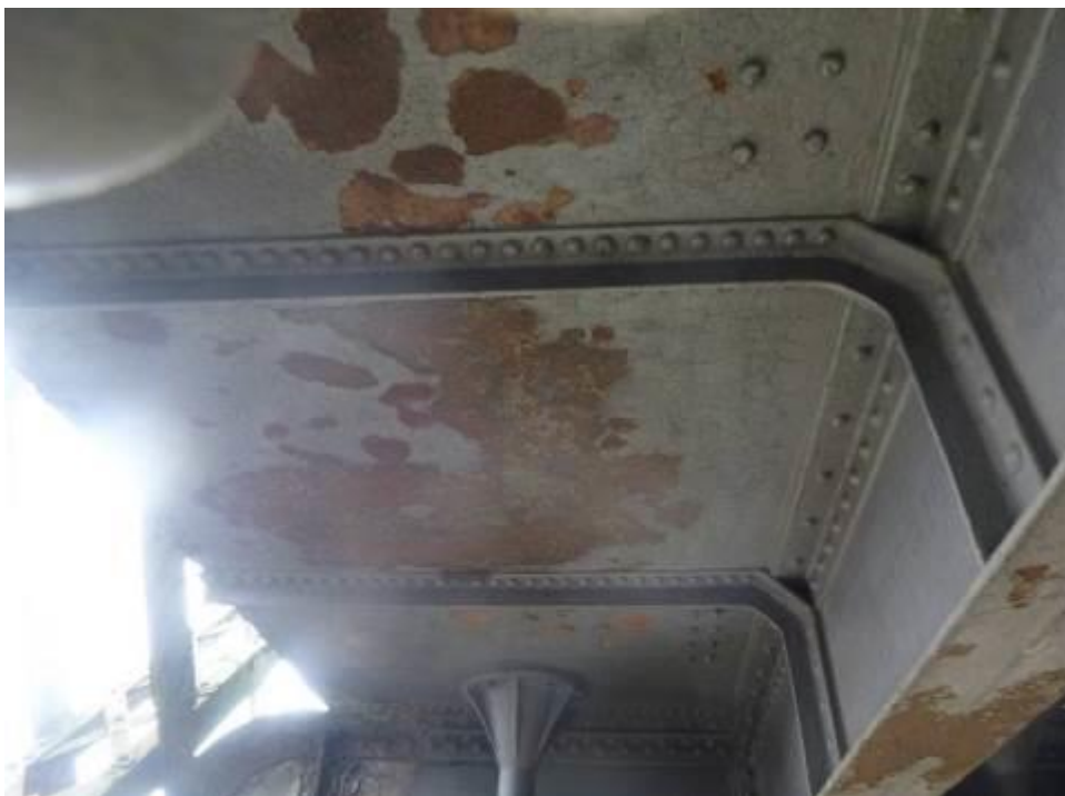
Photograph 196: Spot corrosion to deck of soffit of span 4
