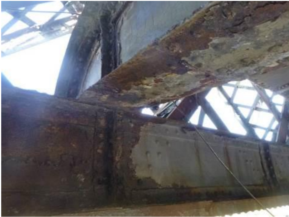
Photograph 187: Loss of thickness & section to T26 of soffit of span 3
