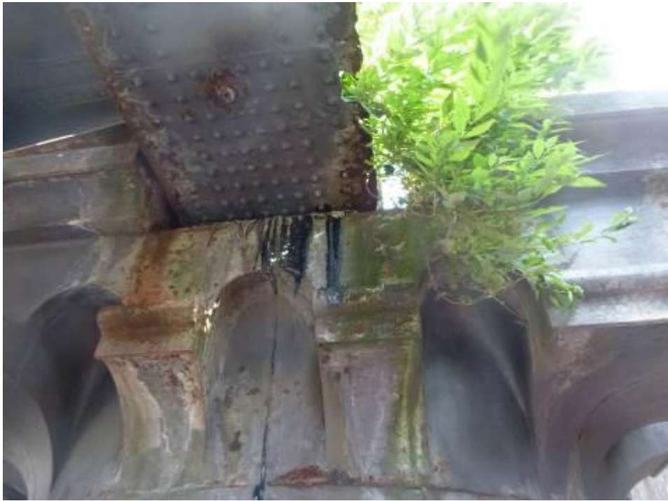
Photograph 41: Area of vegetation growth to south column of pier 1
