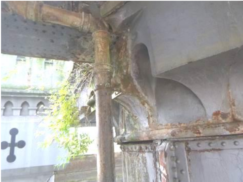
Photograph 59: Area of seepage, vegetation growth & loss of thickness to south column of pier 3
