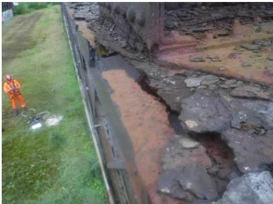
Photograph 111: Loss of section to top boom, top flange of south truss of span 2
