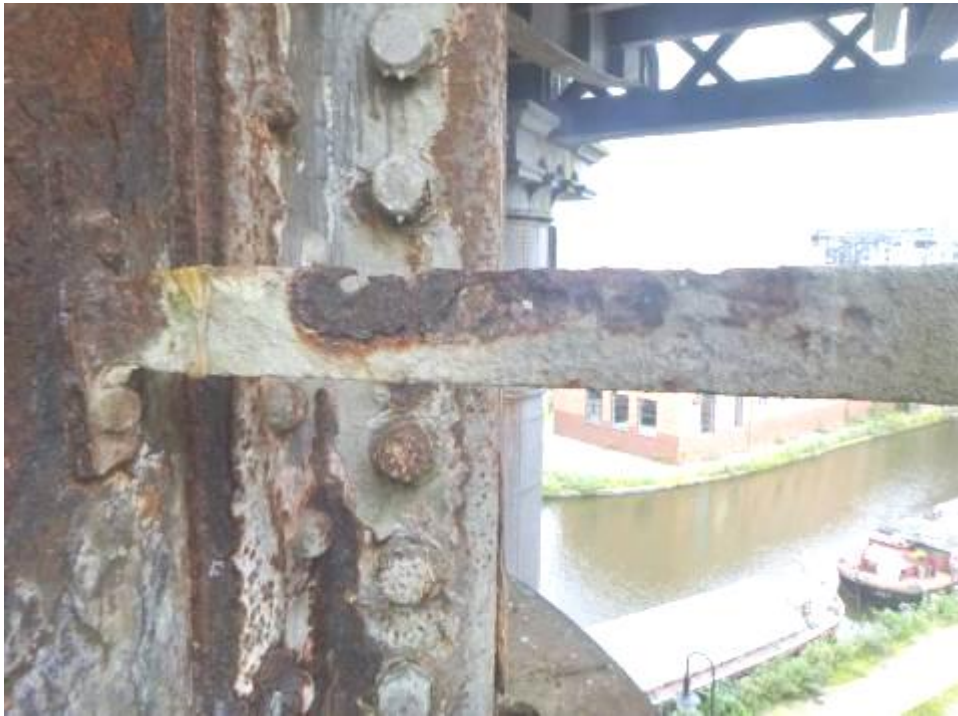
Photograph 75: Area of loss of thickness to drainpipe bracket of south column of pier 4
