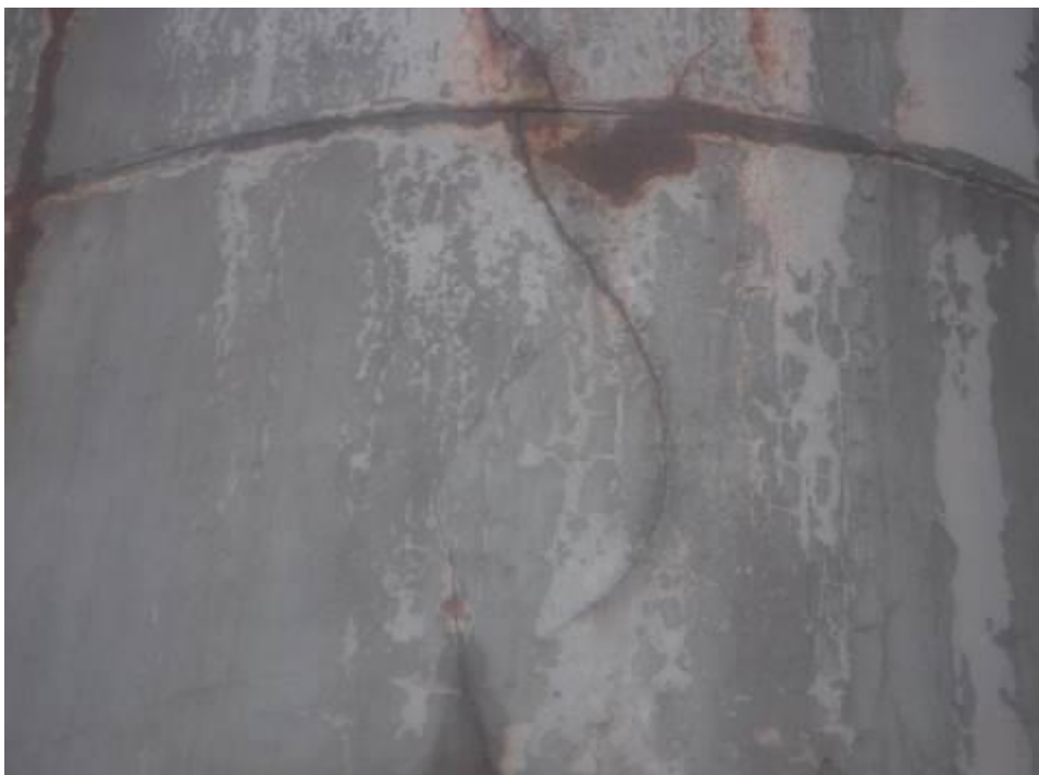
Photograph 46: Diagonal fractures to north column of pier 2
