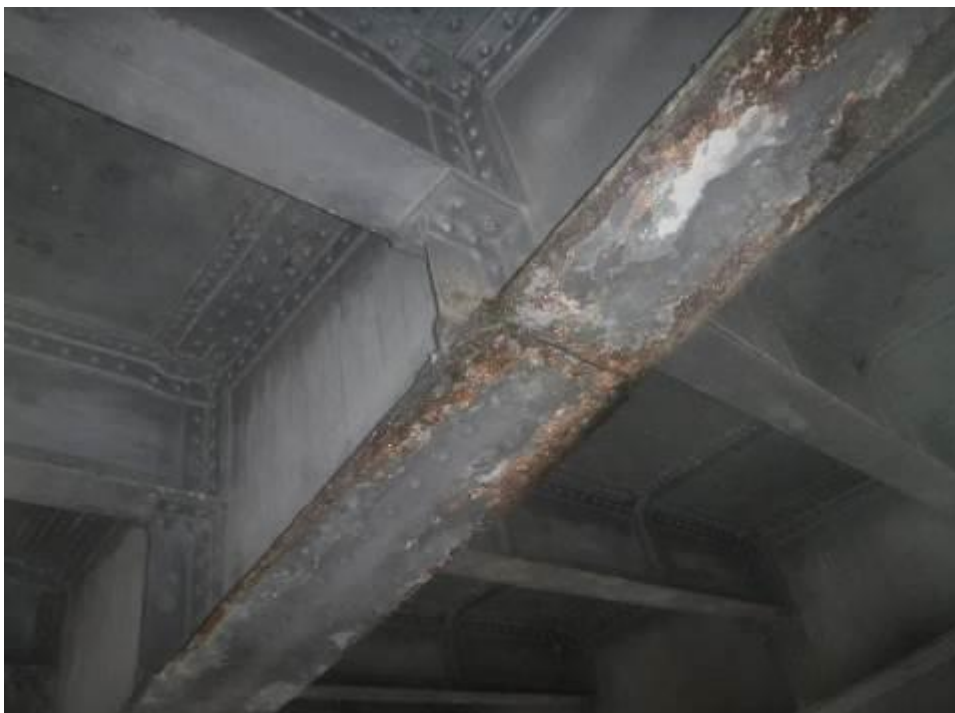
Photograph 210: Corrosion to T57 of soffit of span 6
