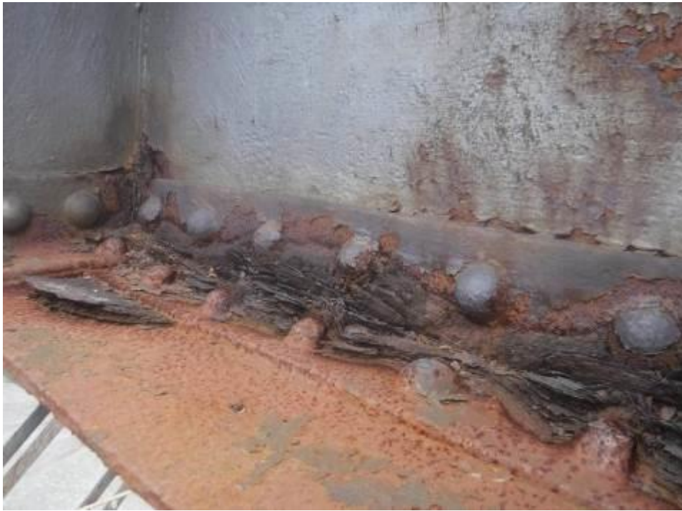
Photograph 175: Typical loss of thickness to west bottom angles of upper transverse steelworks
