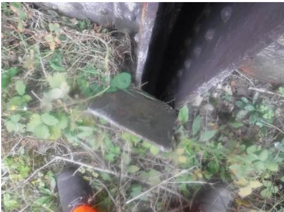
Photograph 166: Deformed & detached ballast plate to north truss of span 8
