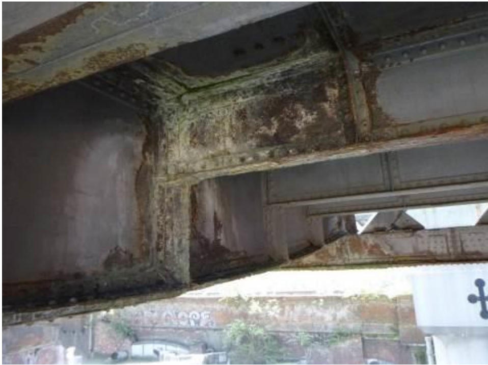
Photograph 189: Surface corrosion & loss of thickness to MG14 of soffit of span 3
