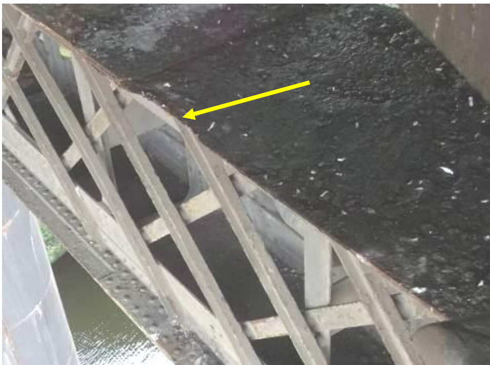
Photograph 56: Area of loss of section to interconnecting truss of pier 3
