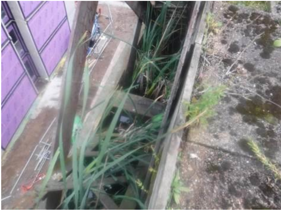
Photograph 165: Vegetation growth to bottom boom of north truss of span 8
