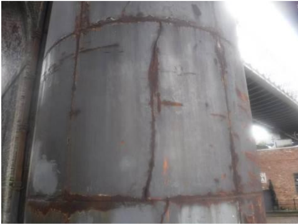
Photograph 51: Vertical fracture to south column of pier 2
