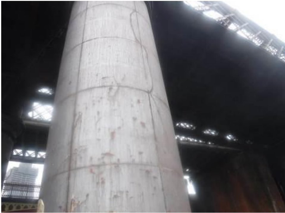
Photograph 67: Vertical fractures to north column of pier 4
