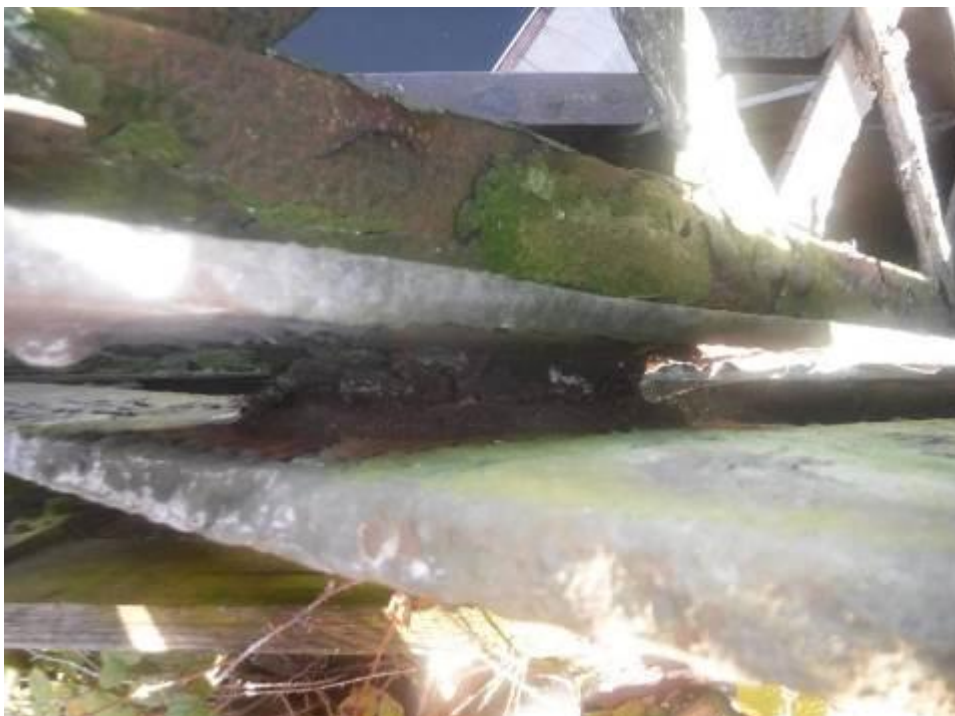
Photograph 136: Rust jacking to diagonal member of north truss of span 5
