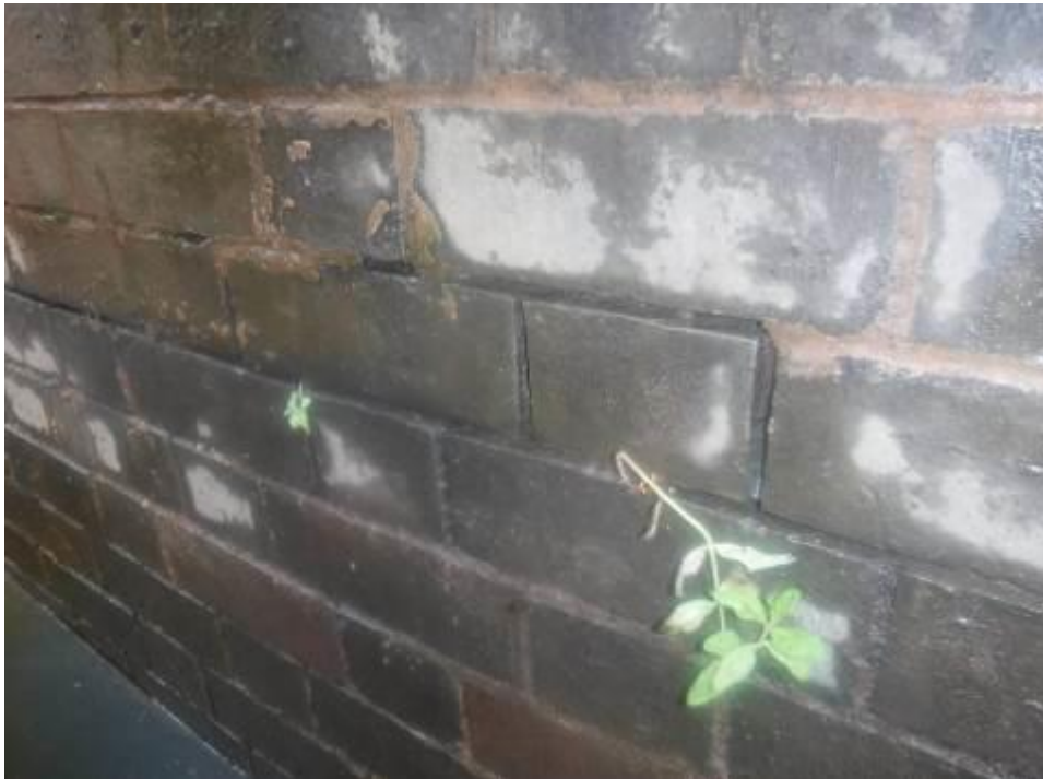
Photograph 29: Area of mortar loss with spot vegetation growth to west abutment
