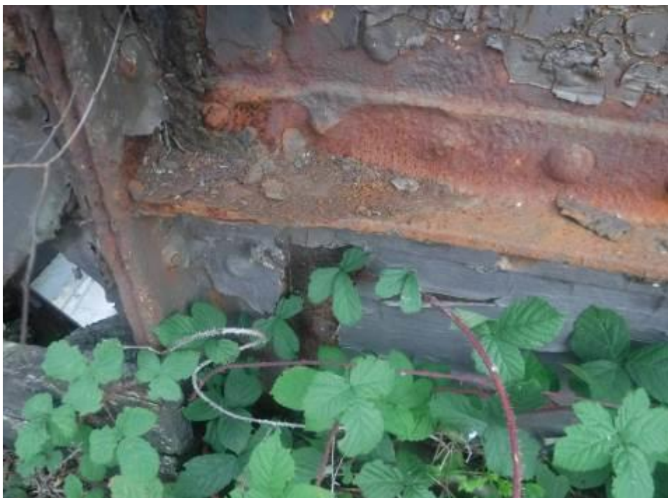
Photograph 152: Loss of thickness to end section, lower horizontal stiffener of north truss of span 7
