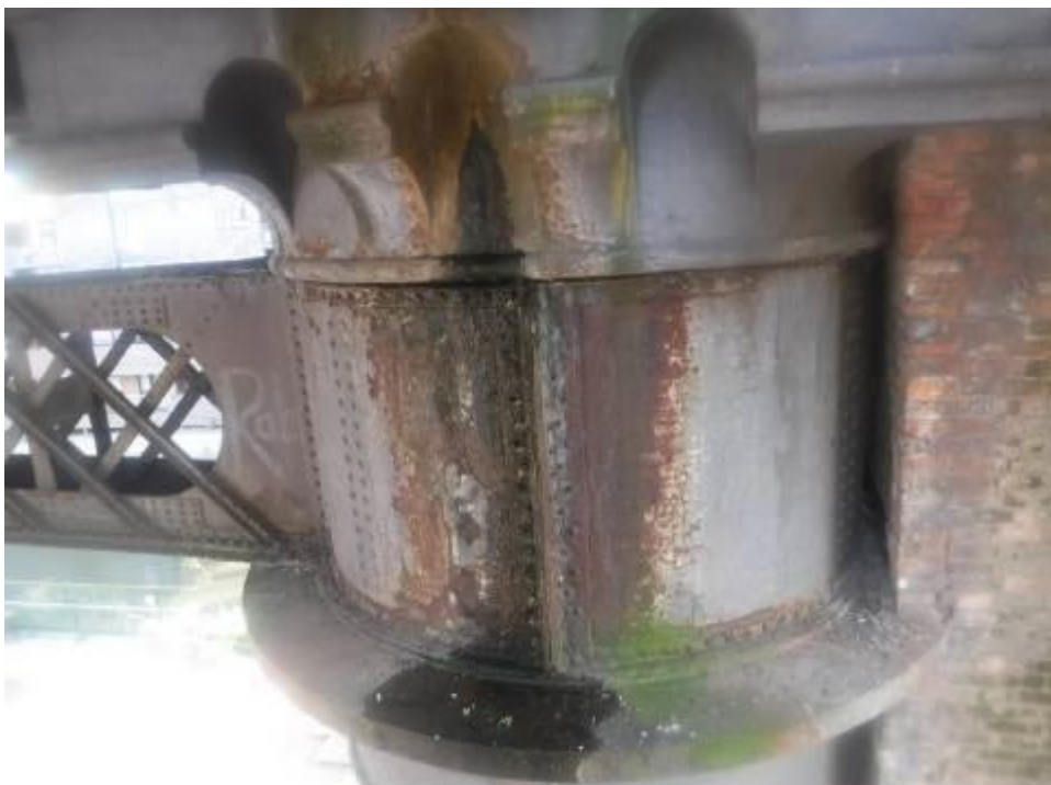
Photograph 88: Area of seepage to south column of pier 7
