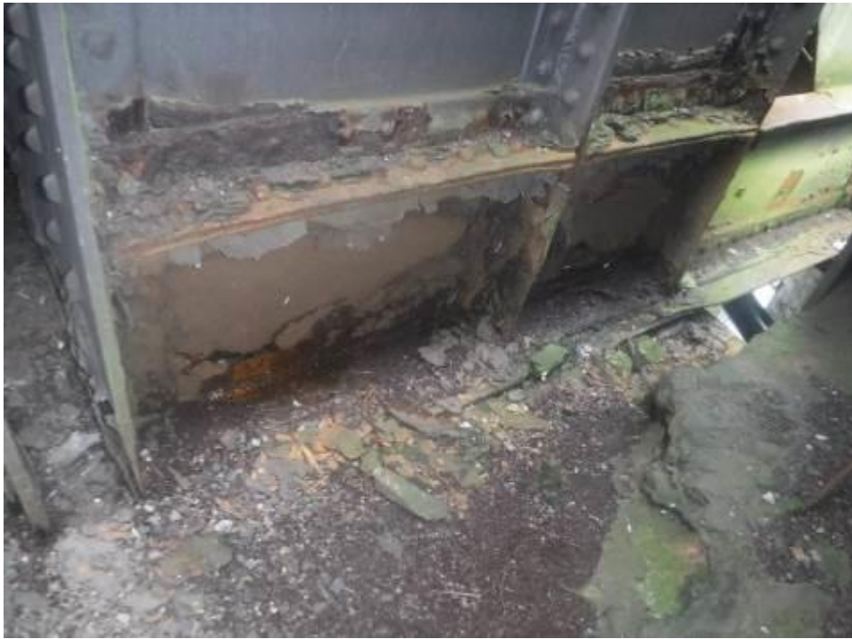
Photograph 145: Loss of thickness to end beam stiffeners of south truss of span 5
