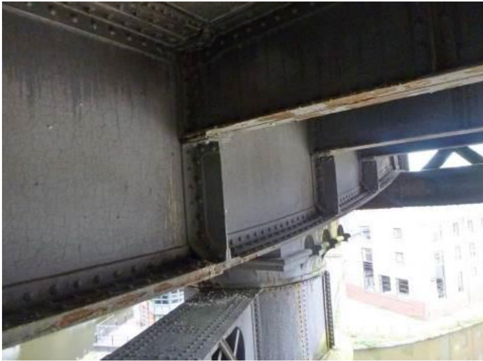
Photograph 193: Typical spot paint loss & surface corrosion to soffit of span 4
