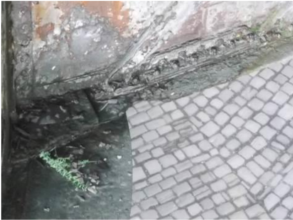
Photograph 37: Area of loss of section to interconnecting truss of pier 1
