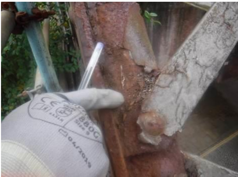
Photograph 120: Loss of thickness to diagonal member of south truss of span 3
