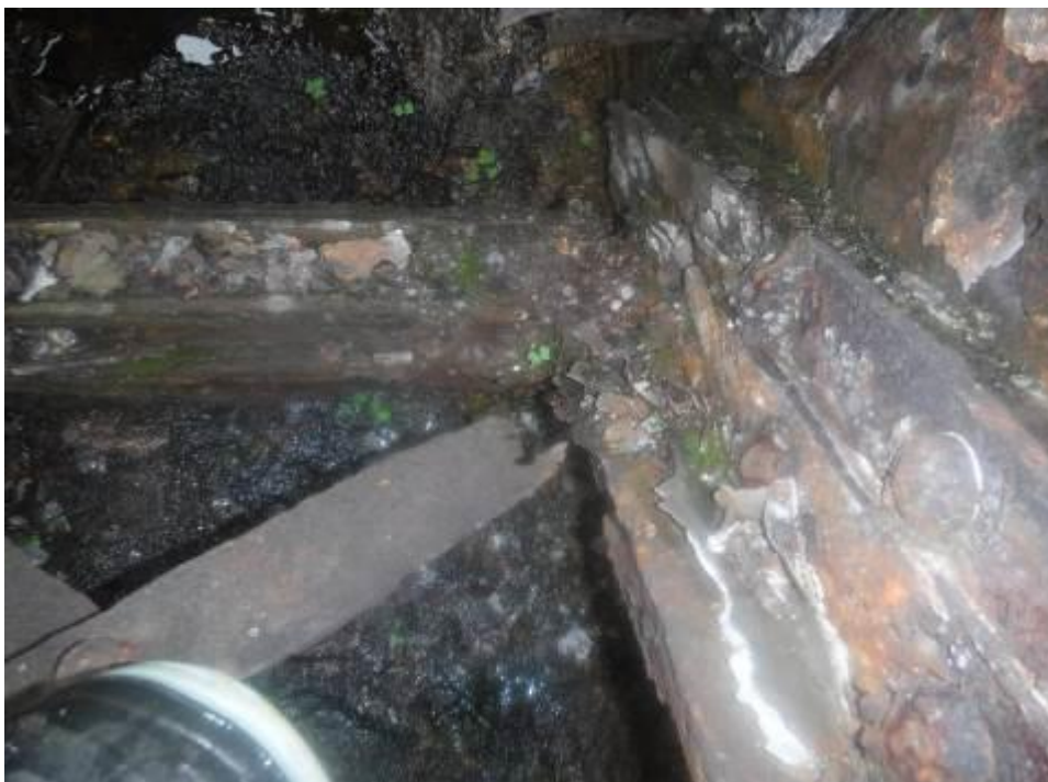
Photograph 122: Loss of section to diagonal bracing of south truss of span 3
