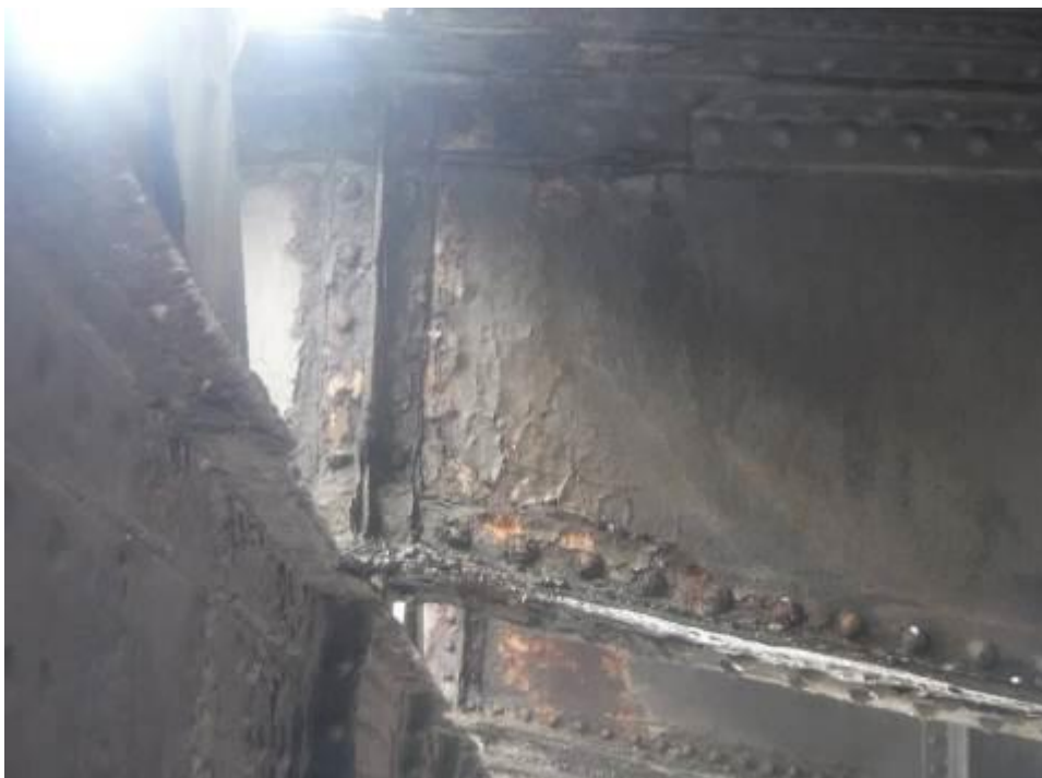
Photograph 208: Typical corrosion & pitting below vertical braces to T57 – T62 of soffit of span 6
