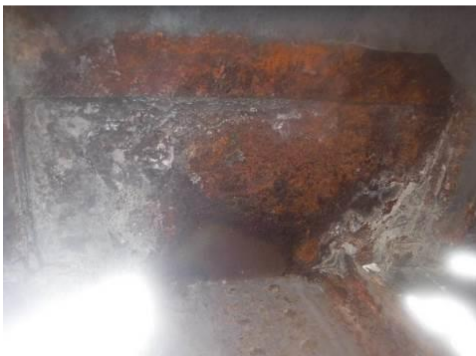
Photograph 224: Surface corrosion & loss of thickness to MGI2 of soffit of span 8
