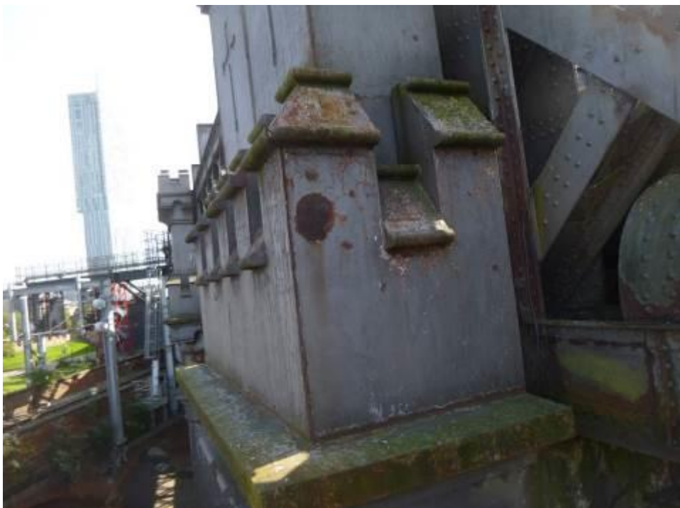
Photograph 90: Typical paint loss & surface corrosion to castle façades of piers
