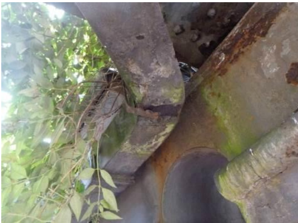
Photograph 184: Loss of section to brackets of old guttering between T19 & T20 of soffit of span 2
