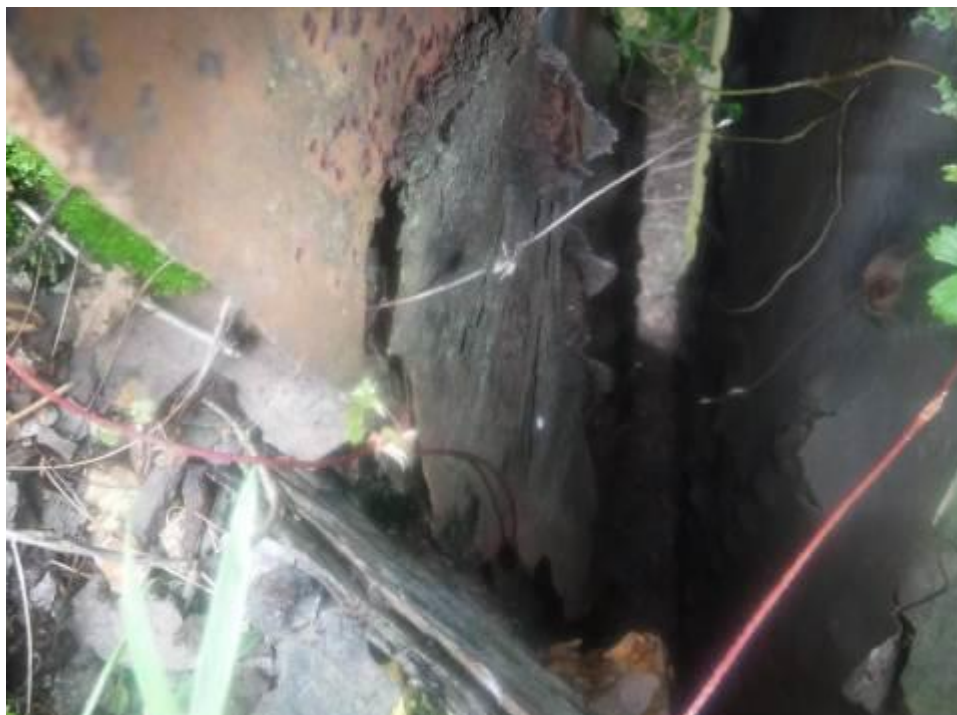
Photograph 129: Loss of section to end plate of south truss of span 4
