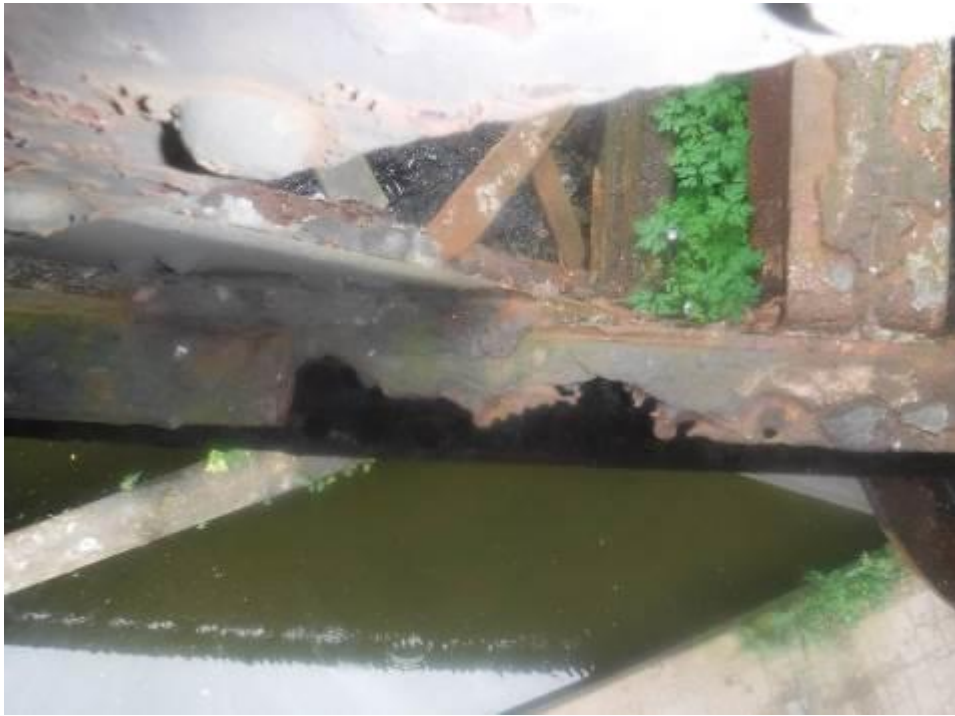
Photograph 121: Loss of section to bottom boom, top flange of south truss of span 3
