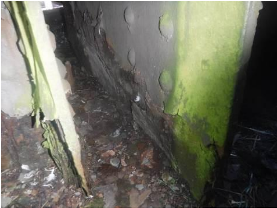
Photograph 133: Loss of thickness to end beam of north truss of span 5
