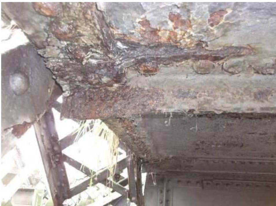
Photograph 206: Loss of thickness & section to MGE2 of soffit of span 5
