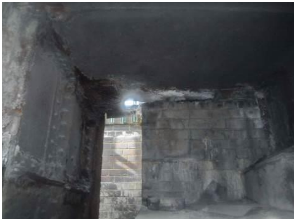
Photograph 223: Loss of section to deck of soffit of span 8
