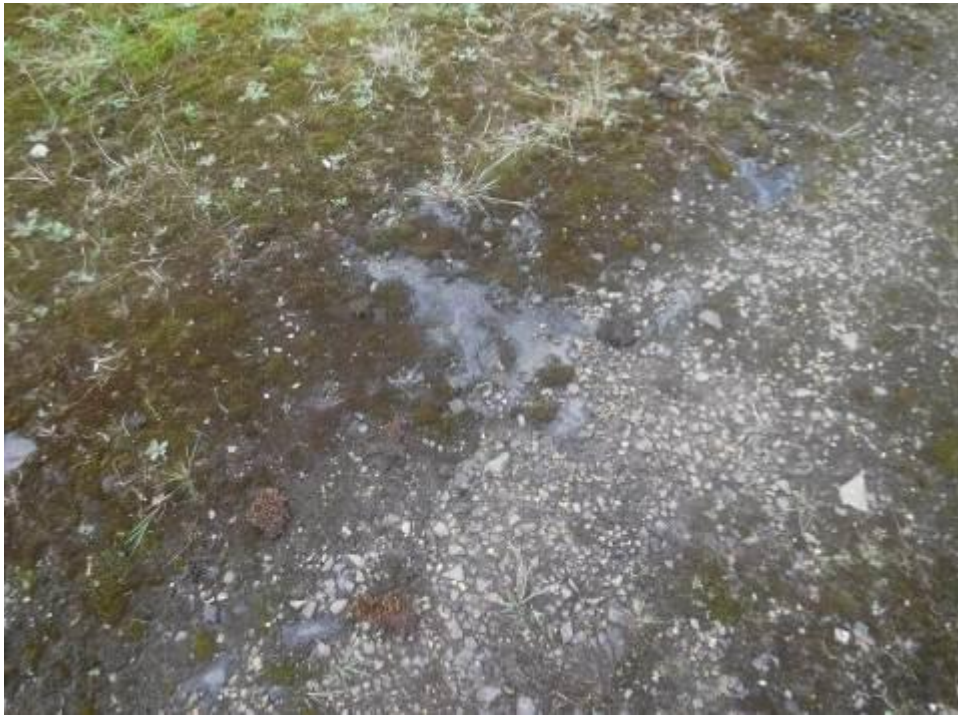
Photograph 235: Typical condition of exposed deck plates to top of deck
