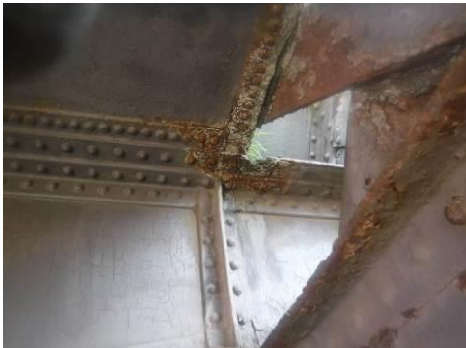
Photograph 219: Loss of thickness & section to T74 of soffit of span 8
