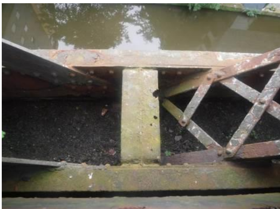
Photograph 148: Loss of section to bottom boom internal stiffener of north truss of span 6
