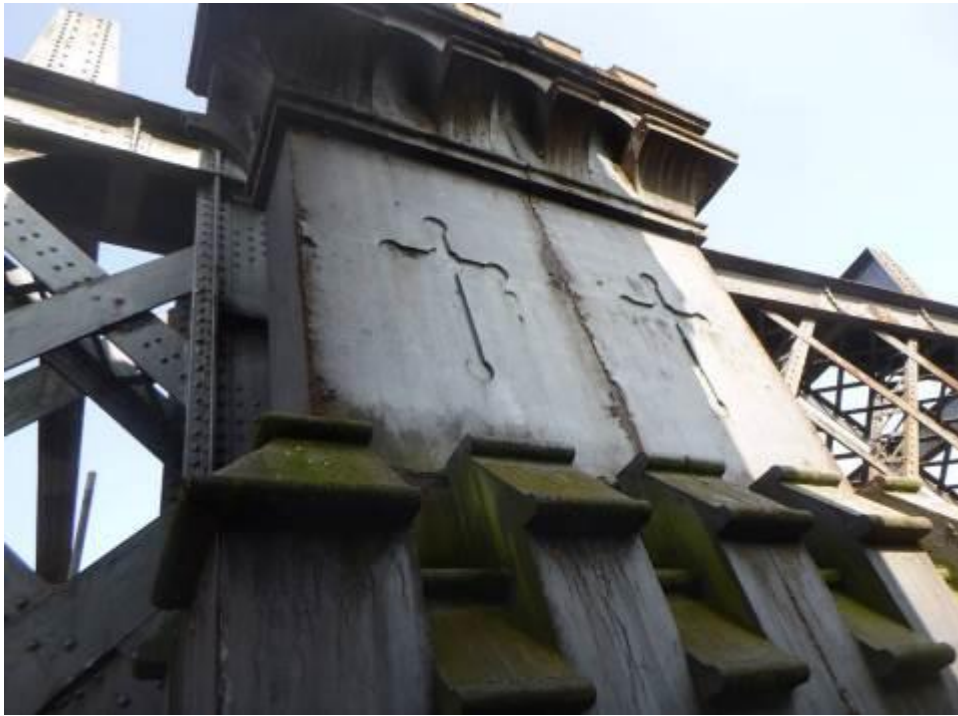
Photograph 89: Typical condition of castle façades to piers
