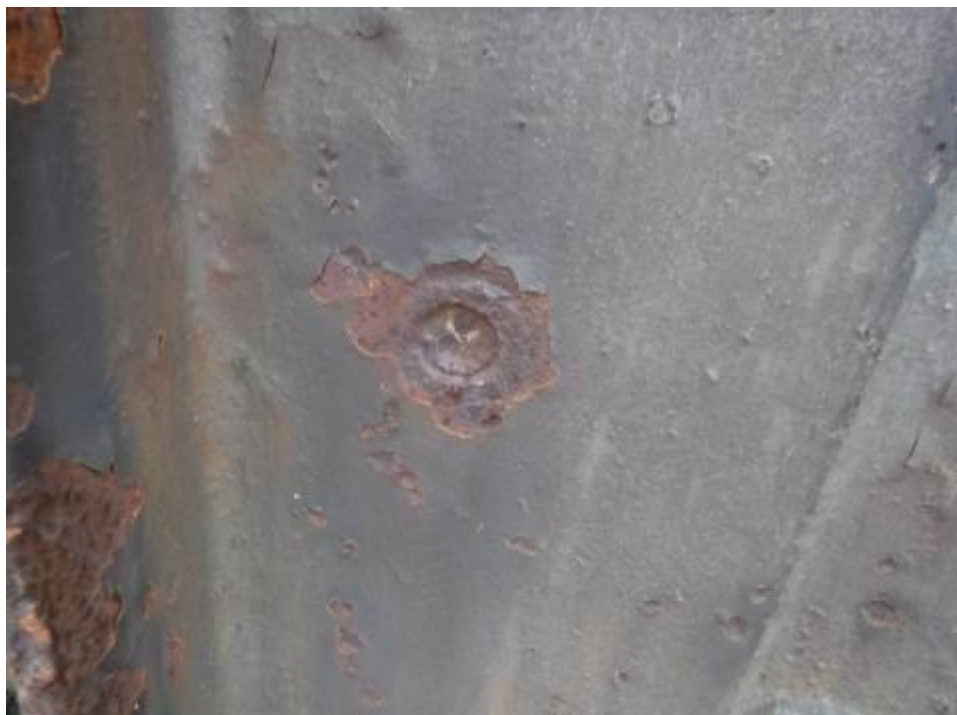
Photograph 169: Missing rivet to end plate of south truss of span 8
