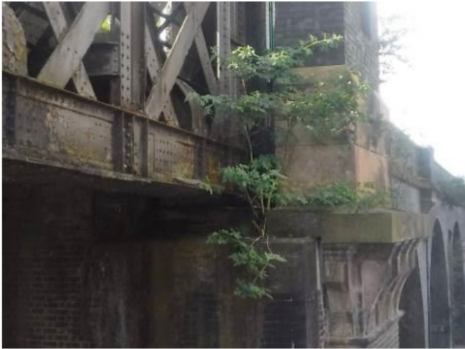
Photograph 33: Sapling growth to bearing shelf of west abutment
