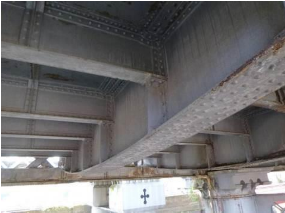
Photograph 185: Typical spot paint loss & surface corrosion to soffit of span 3
