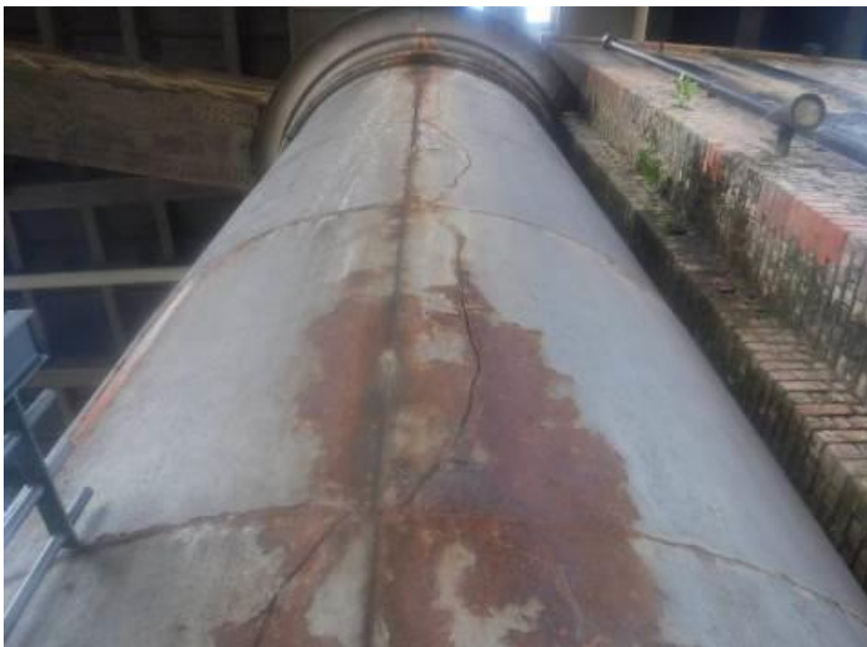
Photograph 82: Vertical fracture & area of loss of thickness to south column of pier 6
