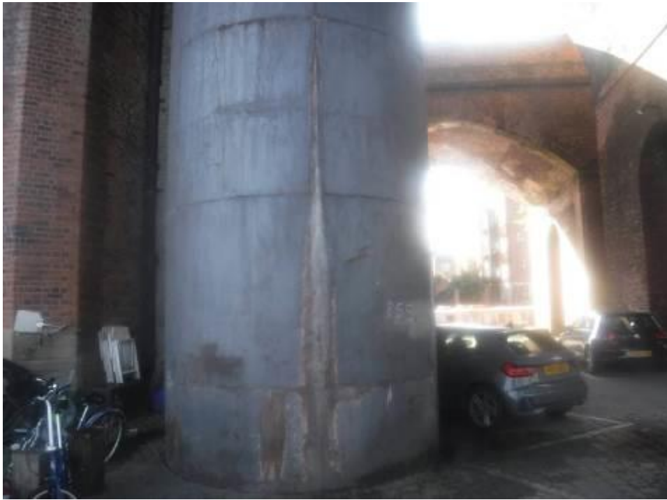
Photograph 79: Area of loss of thickness to south column of pier 5
