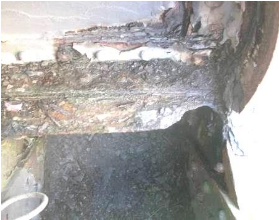
Photograph 81: Area of loss of thickness to interconnecting truss of pier 6
