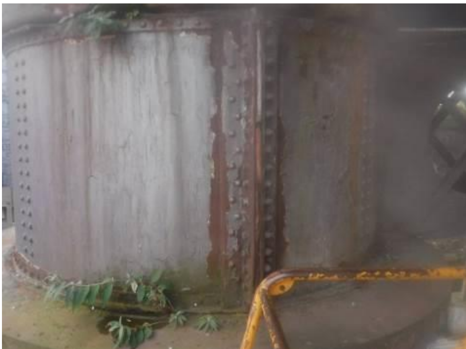
Photograph 86: Vegetation growth & loose / missing / rotten packing timber to north column of pier 7
