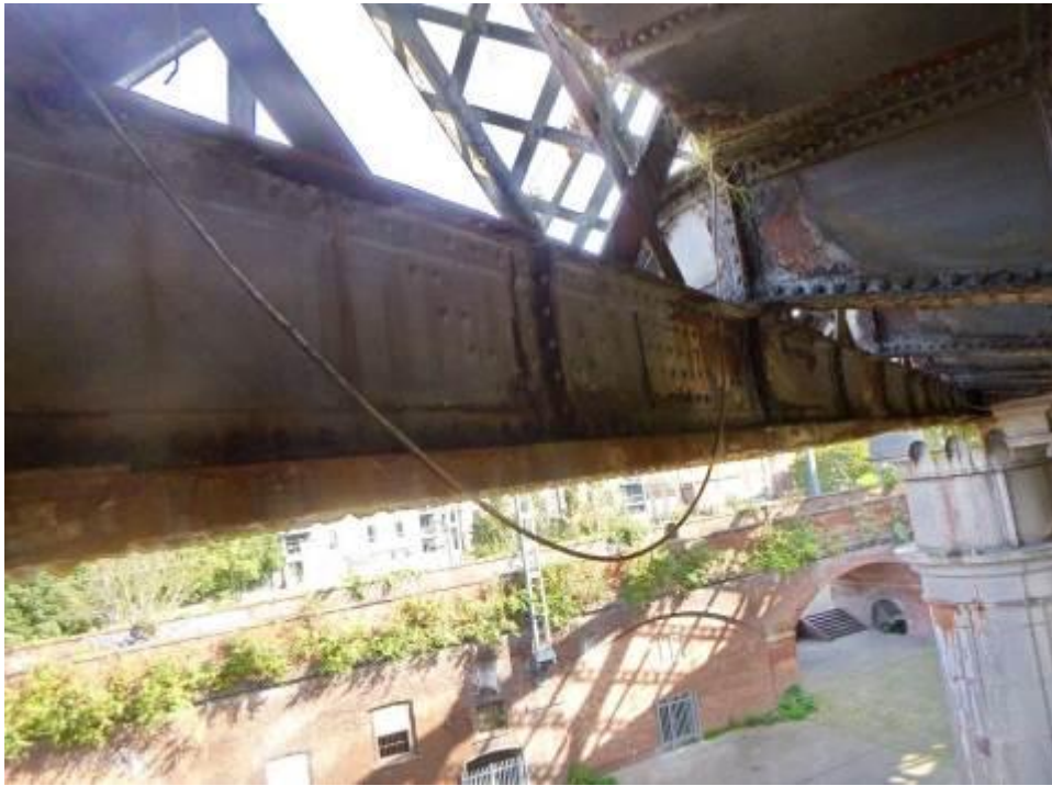
Photograph 191: Lighting cable hanging down by MGE2 of soffit of span 3
