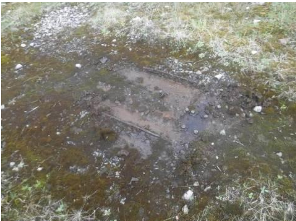
Photograph 236: Typical condition of exposed deck plates to top of deck
