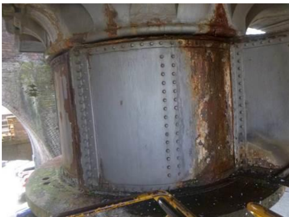
Photograph 50: Area of seepage & loss of thickness to south column of pier 2
