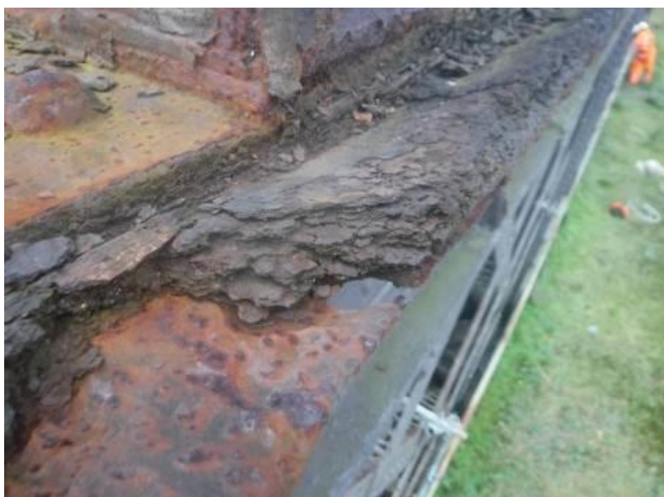
Photograph 112: Loss of section to top boom, top flange of south truss of span 2
