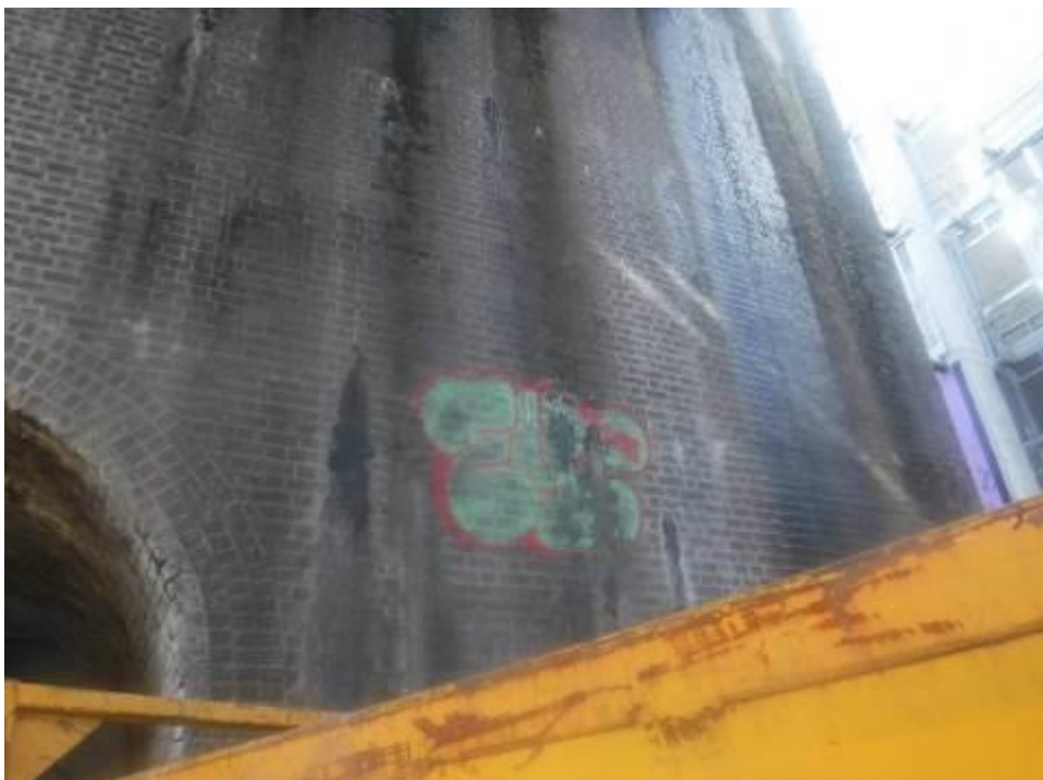
Photograph 28: Typical graffiti & seepage to west abutment
