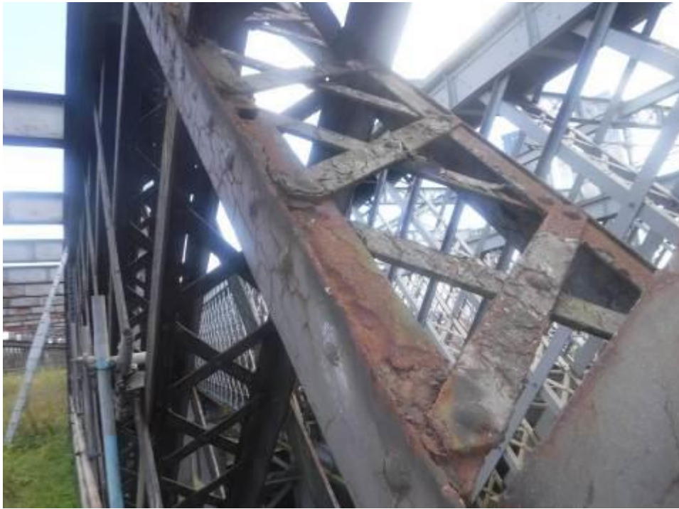
Photograph 141: Loss of thickness & section to diagonal bracing of south truss of span 5
