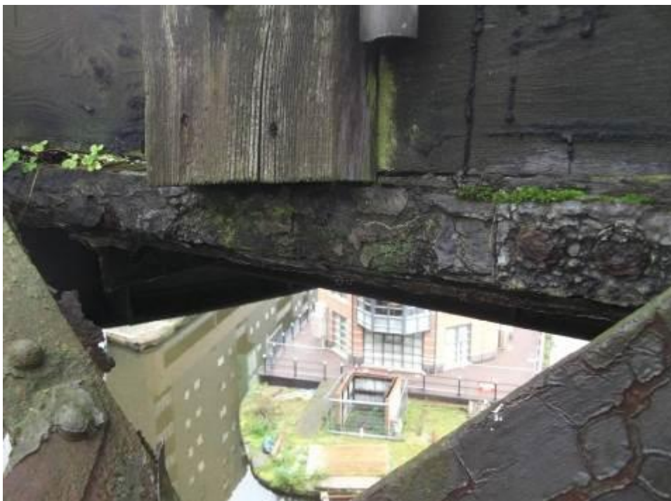
Photograph 202: Typical loss of thickness to deck edge / angle / riser of soffit of span 5
