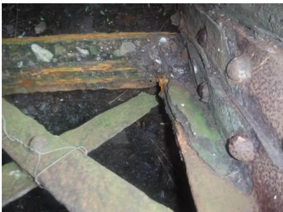
Photograph 118: Loss of section to diagonal bracing of north truss of span 3
