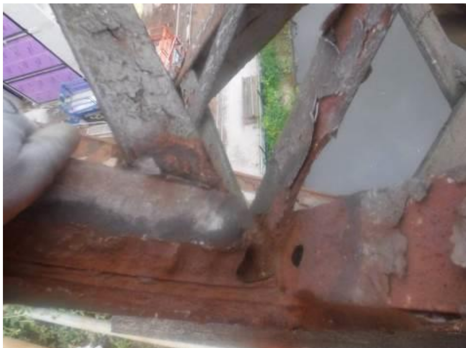
Photograph 155: Loss of thickness & section to diagonal member of north truss of span 7
