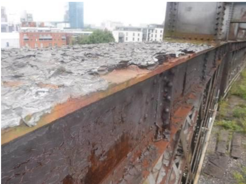
Photograph 124: Loss of thickness to top boom, top flange of north truss of span 4
