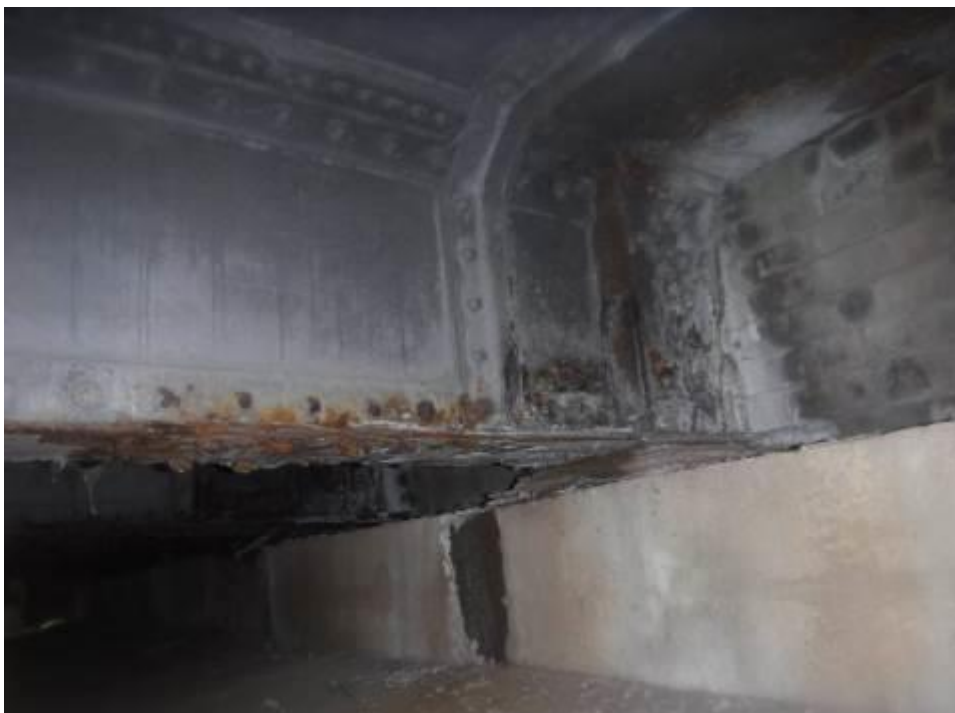
Photograph 218: Typical loss of thickness & section to MGIs at bearing points of soffit of span 8
