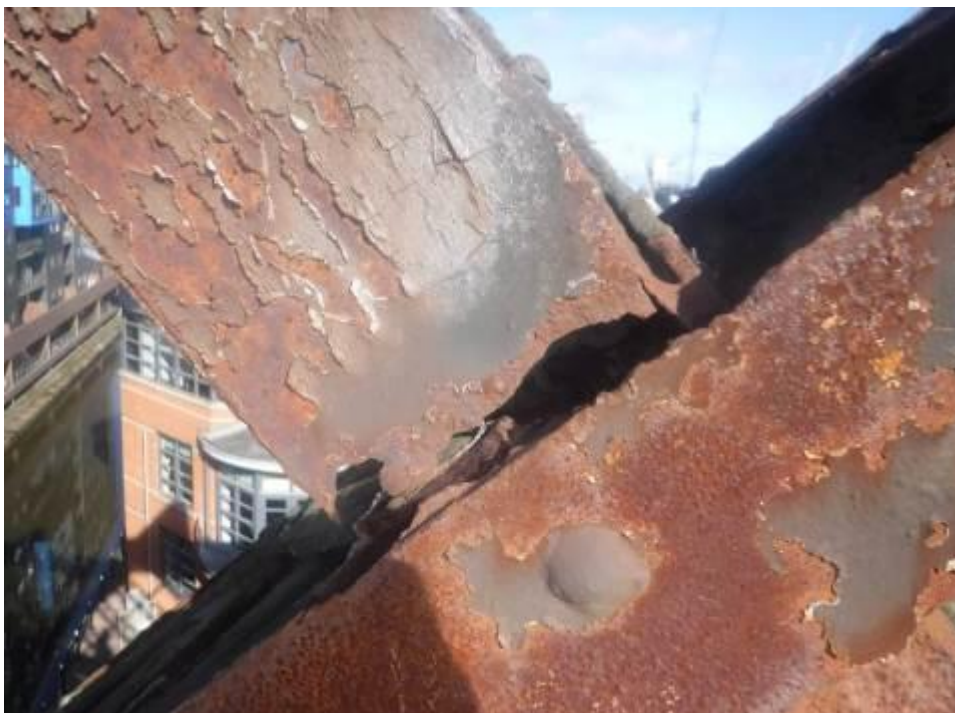
Photograph 134: Loss of section to diagonal member of north truss of span 5
