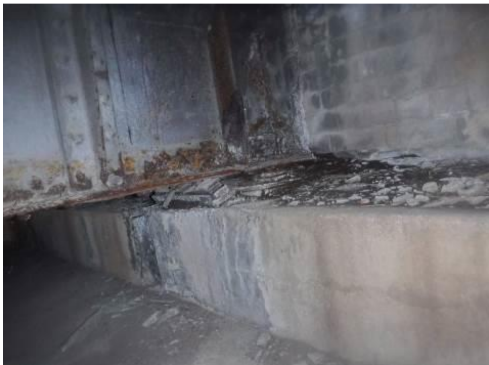
Photograph 31: Rust debris to bearing plinth of west abutment
