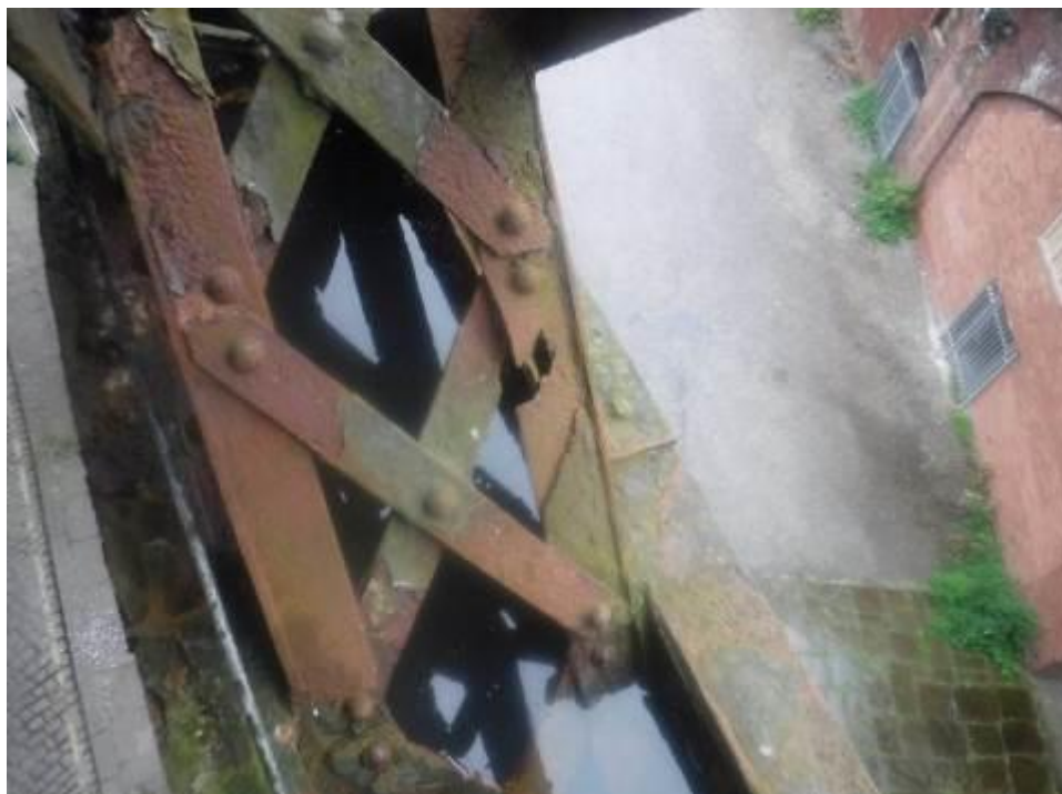
Photograph 105: Loss of section to diagonal bracing of north truss of span 2
