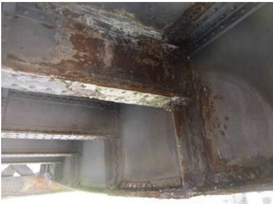
Photograph 192: Loss of thickness to MGI2, deck & T21 of soffit of span 3
