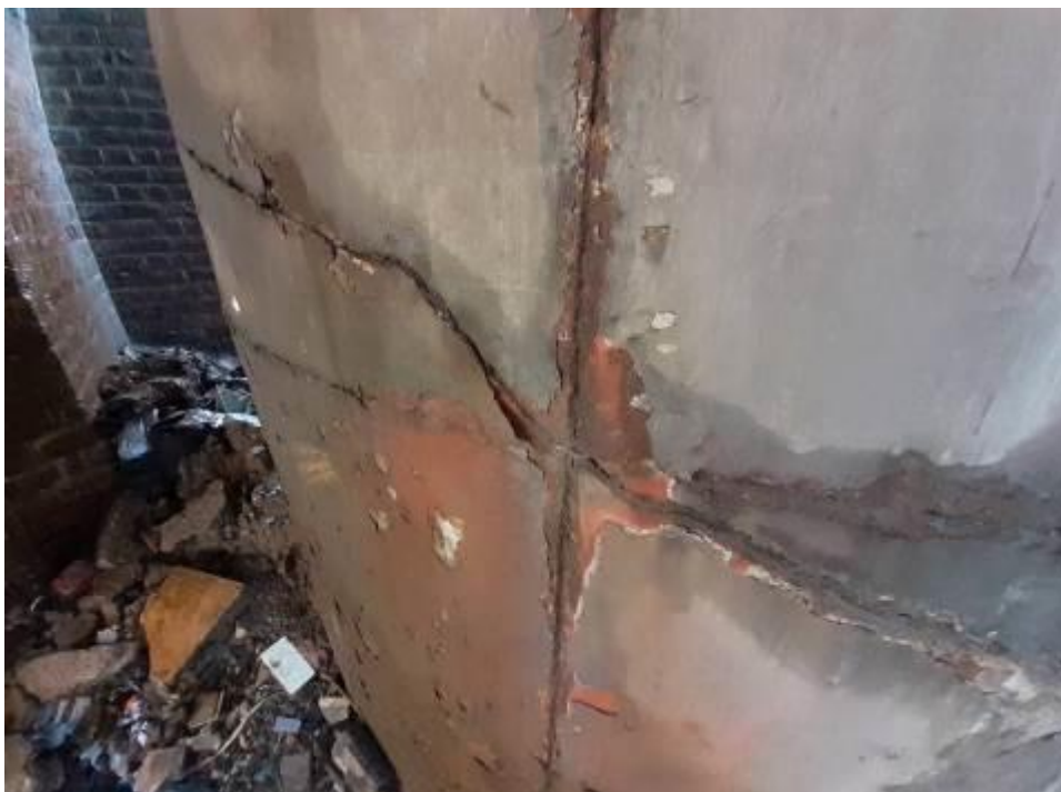
Photograph 42: Horizontal fracture to extra column of pier 1
