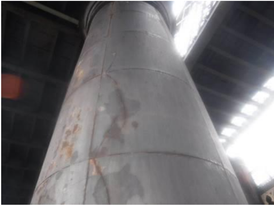
Photograph 71: Vertical fractures to south column of pier 4
