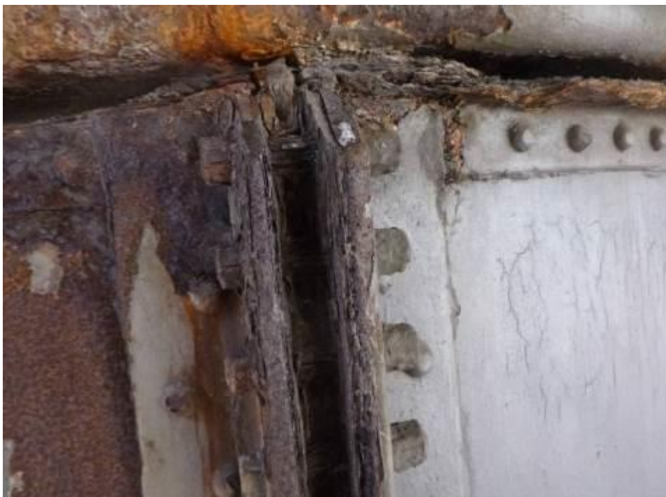
Photograph 52: Missing packing timber & loss of thickness to south column of pier 2
