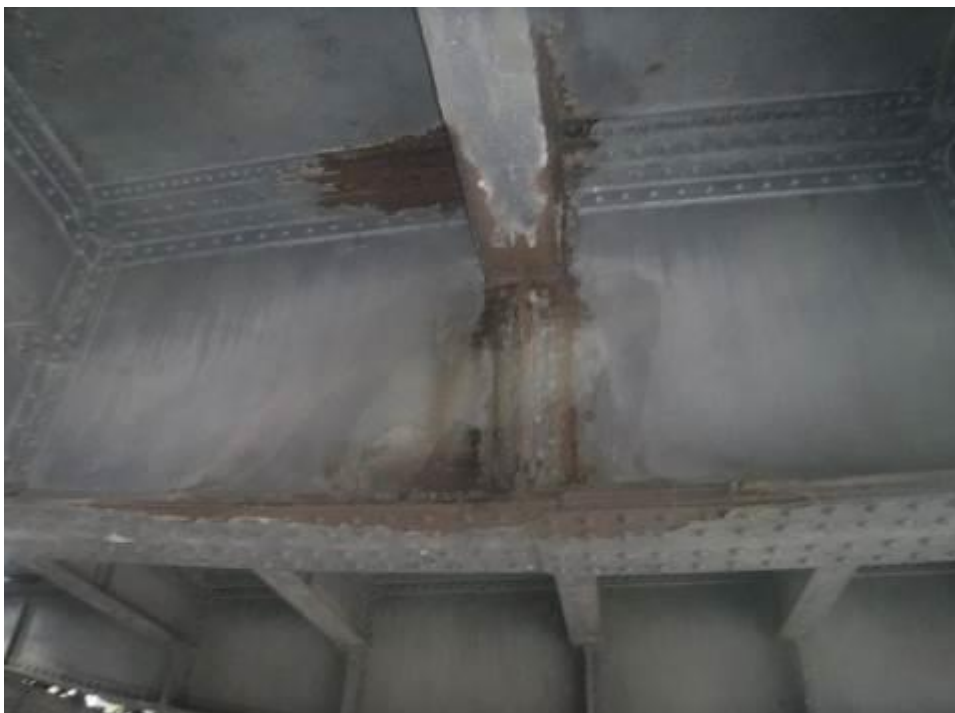
Photograph 204: Paint loss & surface corrosion to MGE1 & T47 connection to soffit of span 5
