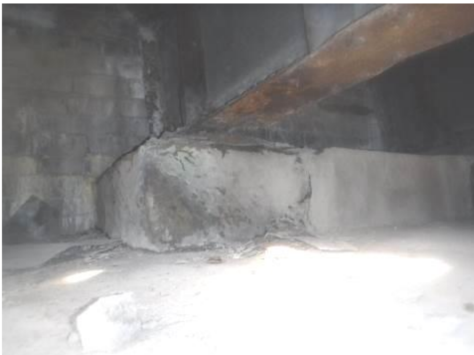
Photograph 30: Area of spalled concrete to bearing plinth of west abutment
