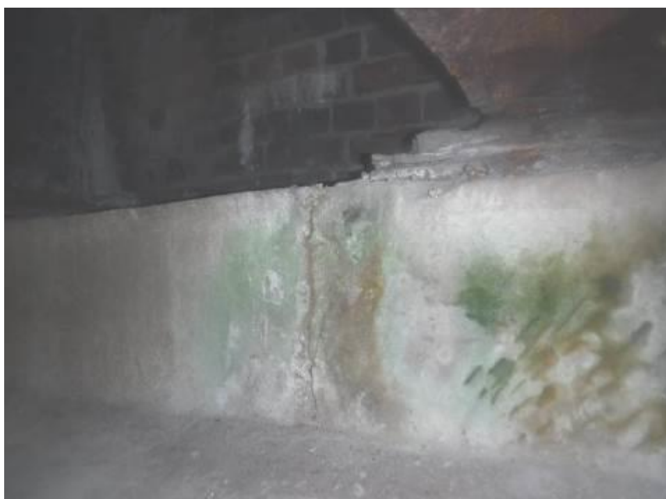
Photograph 32: Vertical fracture to bearing plinth of west abutment
