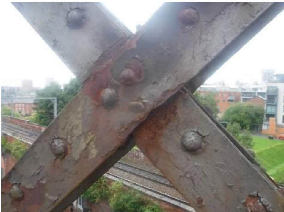
Photograph 96: Typical loss of thickness to truss section diagonal member joints
