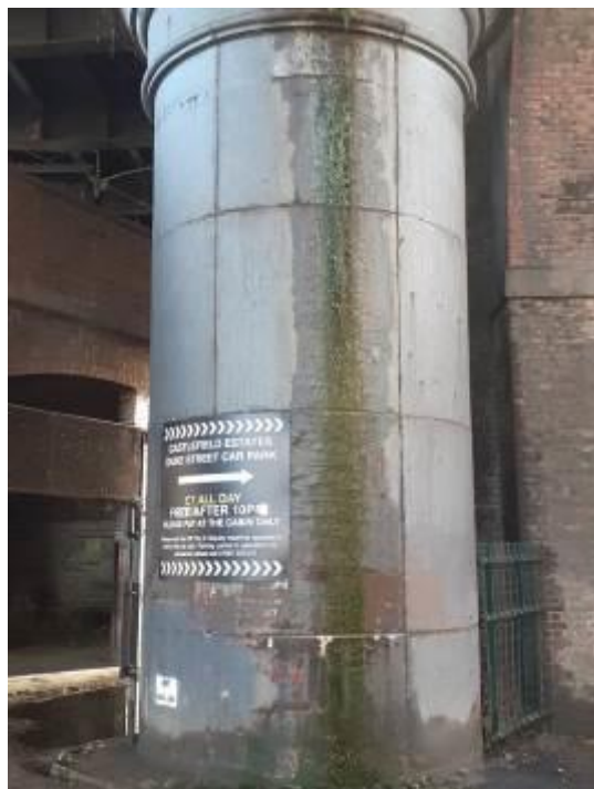
Photograph 44: Area of seepage & algae growth to extra column of pier 1
