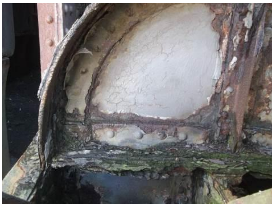
Photograph 216: Loss of thickness & section T63 at MGE1 connection of soffit of span 7
