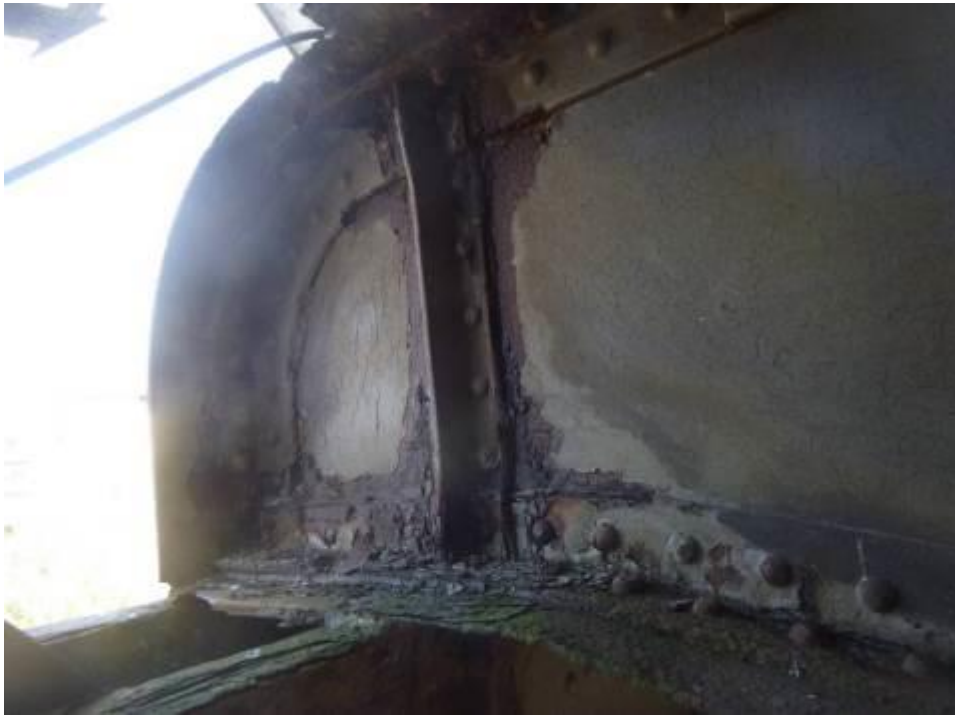
Photograph 179: Typical loss of thickness to transverse girders of soffit of span 2 at MGE connections
