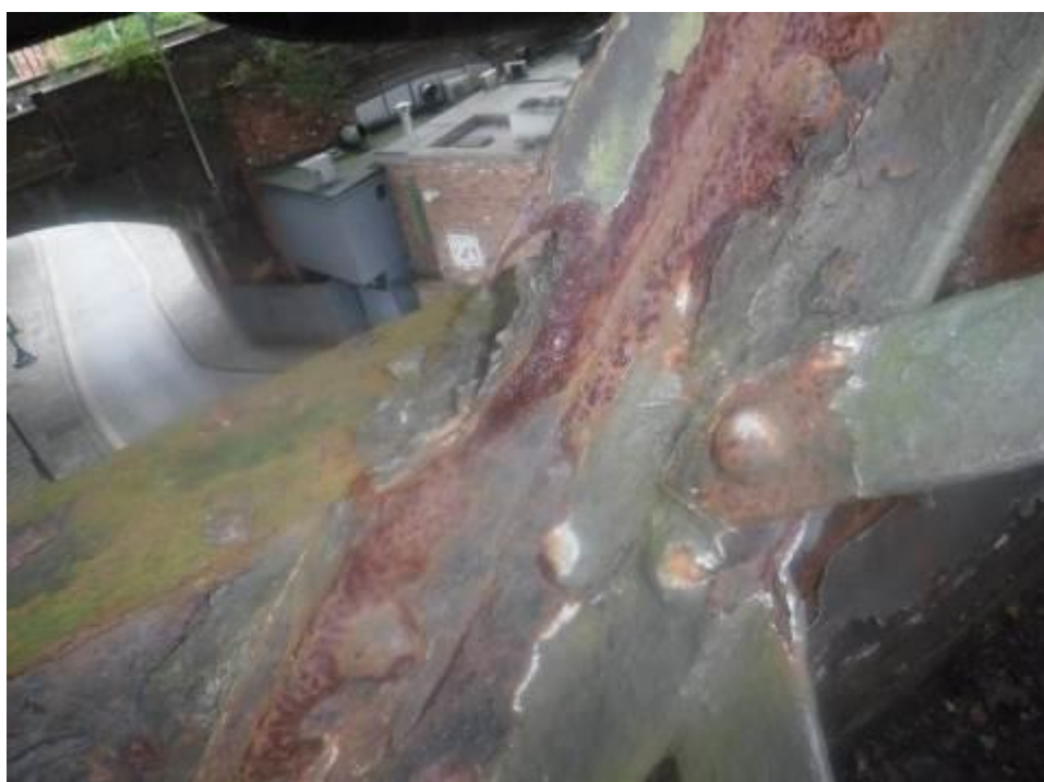
Photograph 116: Loss of section to diagonal member of north truss of span 3
