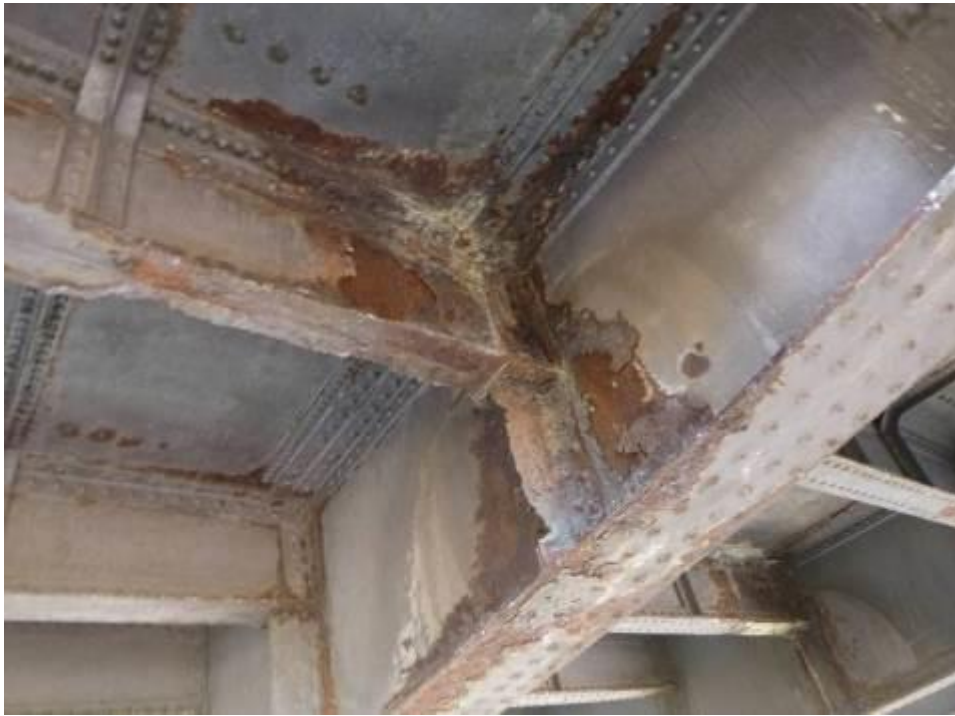
Photograph 183: Loss of thickness & section to T20 & MGI2 of soffit of span 2
