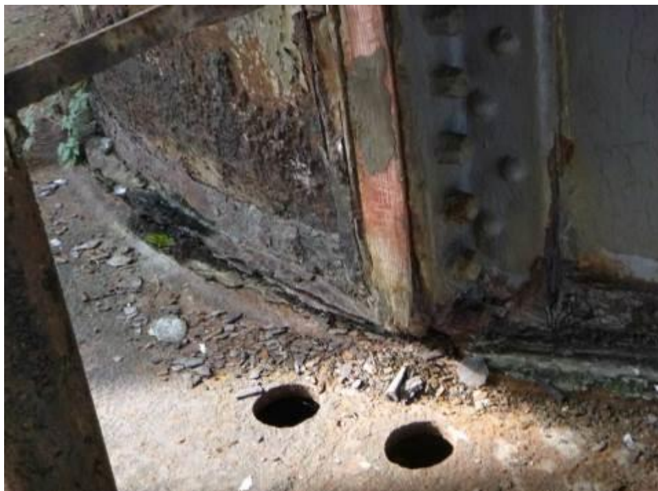
Photograph 61: Area of loss of section to south column of pier 3
