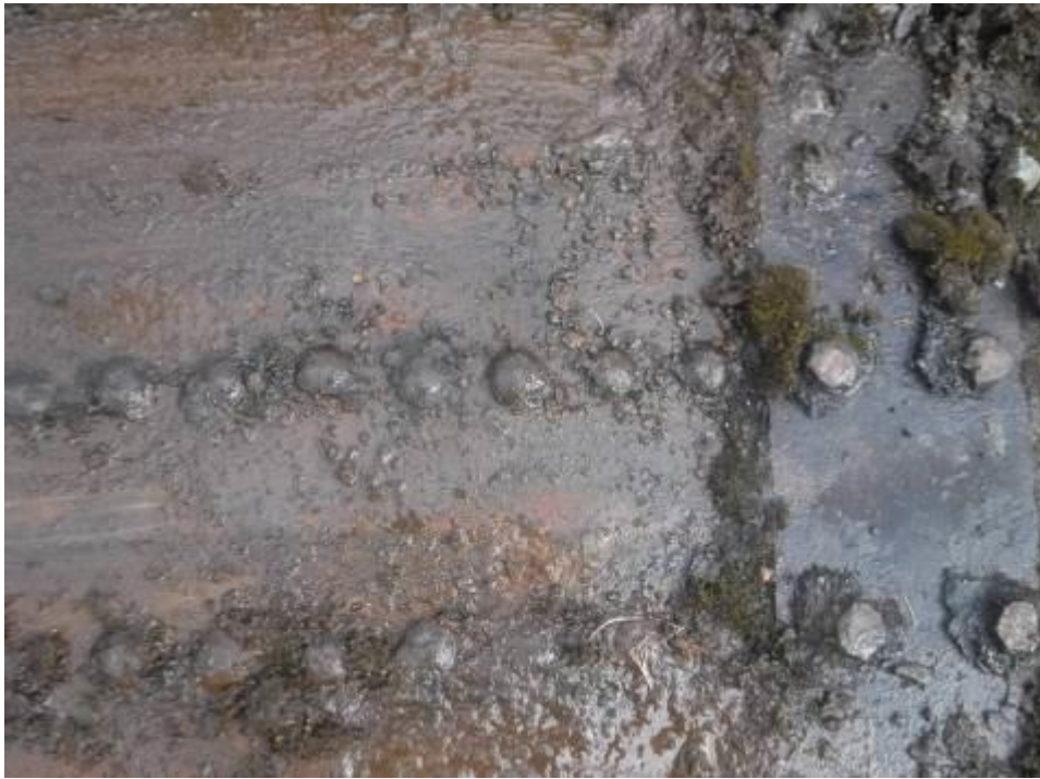
Photograph 237: Typical condition of exposed deck plates to top of deck
