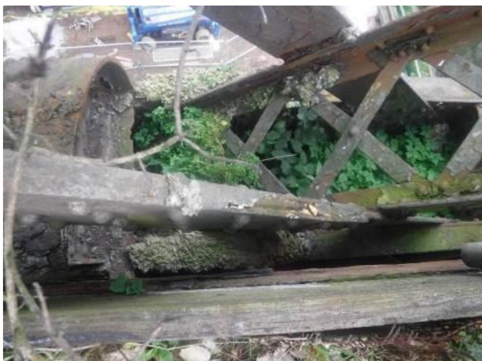
Photograph 156: Concrete & vegetation growth to bottom boom of north truss of span 7
