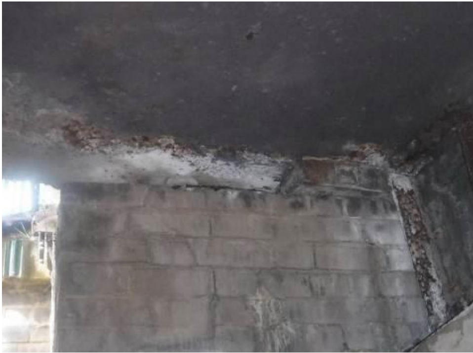
Photograph 27: Area of missing & displaced brickwork to ballast wall of west abutment
