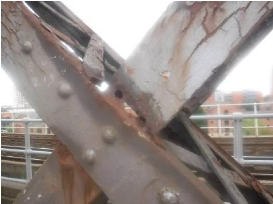
Photograph 159: Loss of thickness & section to diagonal member of south truss of span 7
