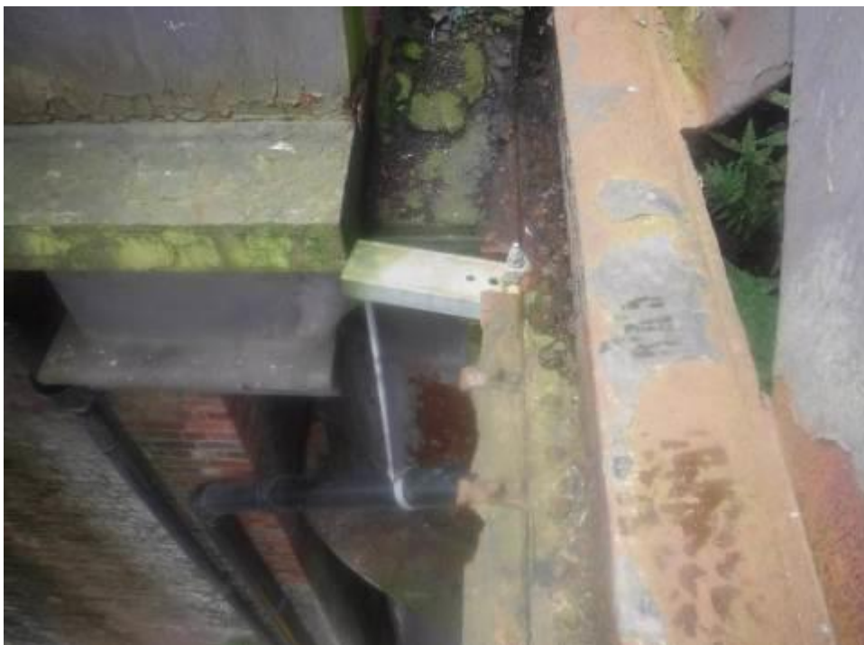
Photograph 160: Loss of section to bottom boom, bottom flange of south truss of span 7
