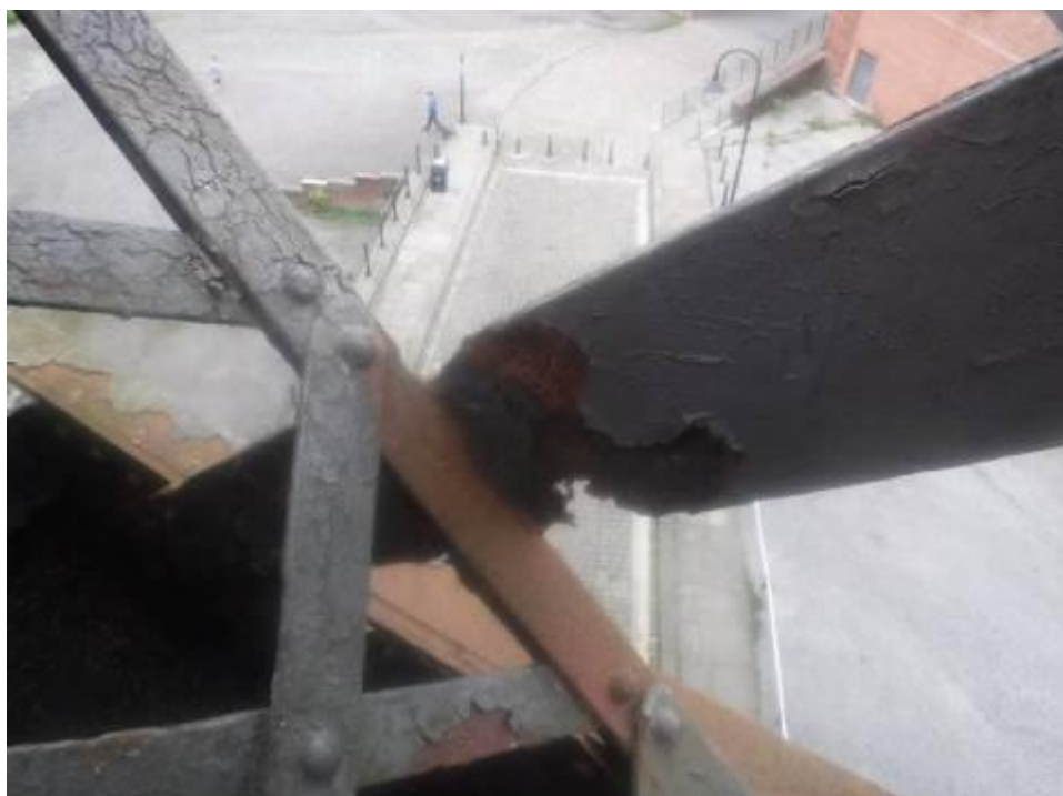
Photograph 117: Loss of section to diagonal bracing of north truss of span 3
