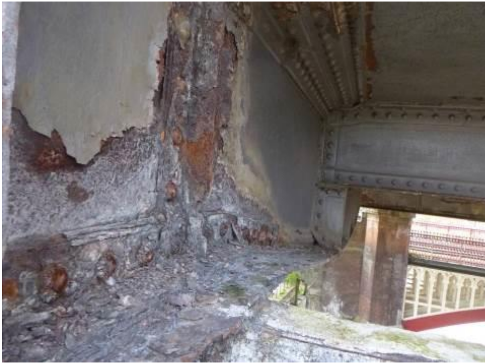
Photograph 195: Loss of thickness to vertical stiffener of T36 to soffit of span 4
