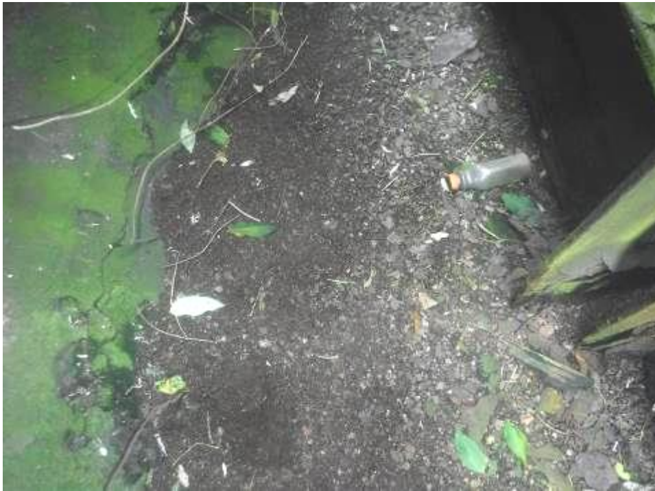
Photograph 95: Typical debris to tops of piers within castle façades
