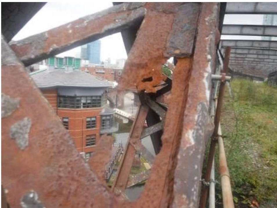
Photograph 146: Loss of thickness & section to diagonal member of north truss of span 6
