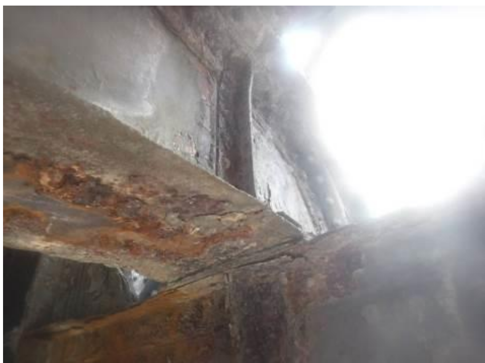
Photograph 222: Loss of thickness to T84 of soffit of span 8
