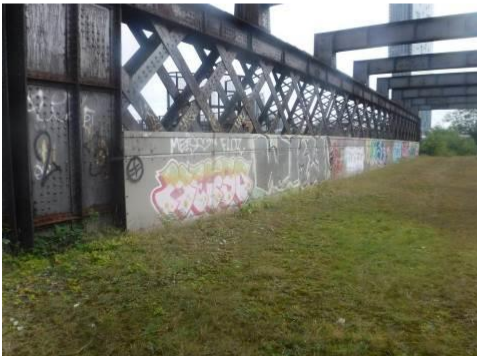
Photograph 234: Graffiti to barrier fence to east end of north truss
