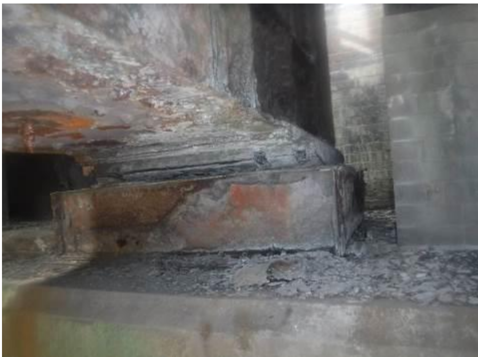
Photograph 24: Loss of thickness & loss of section to south bearing of west abutment
