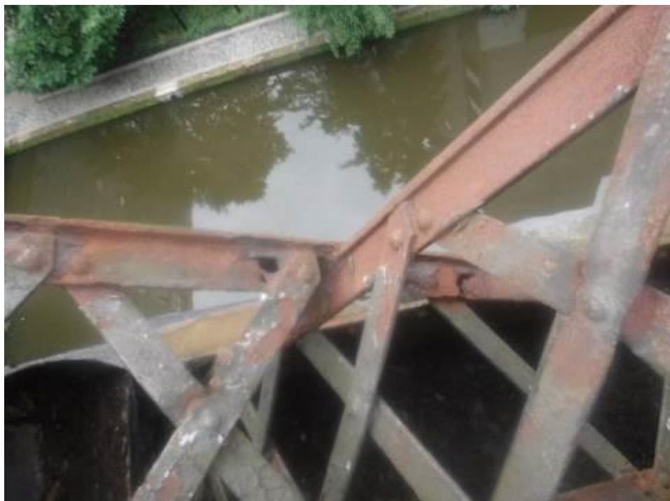
Photograph 147: Loss of thickness & section to diagonal member of north truss of span 6
