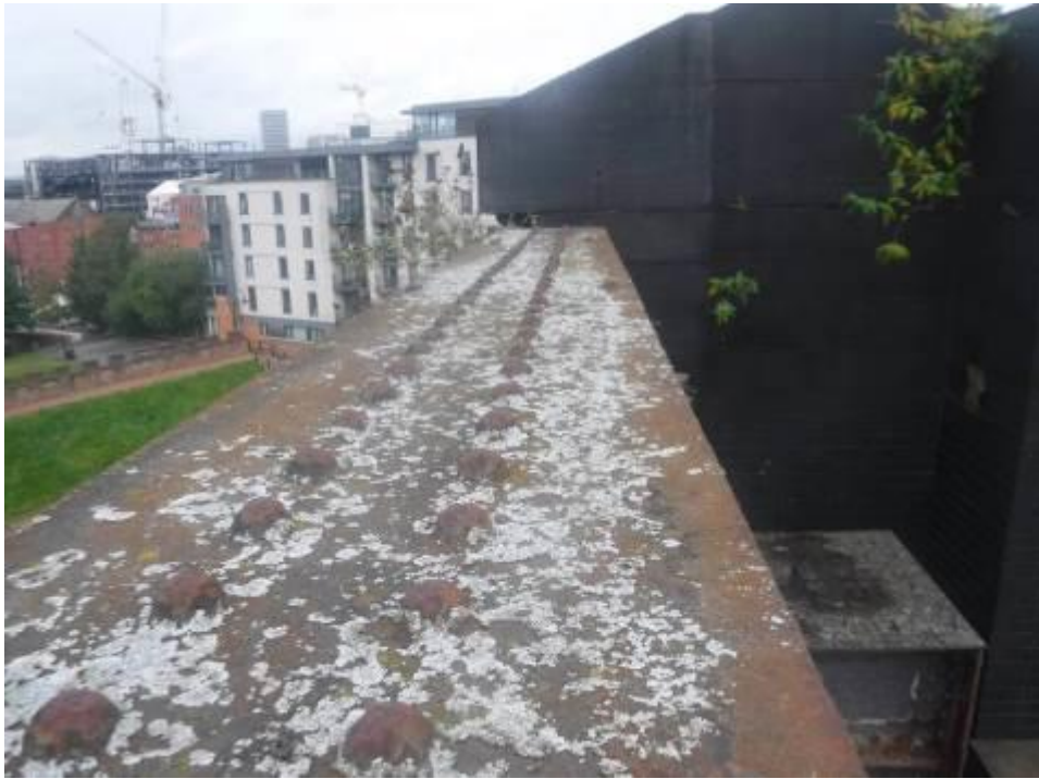
Photograph 173: Typical paint loss, surface corrosion & pitting to tops of upper transverse steelworks
