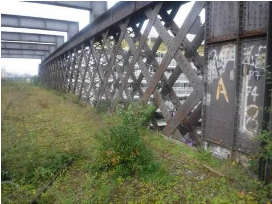
Photograph 233: No ballast boards to span 8 top of deck
