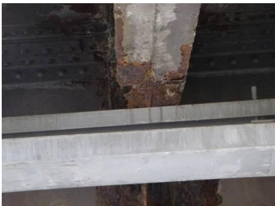
Photograph 182: Corrosion, pitting & loss of section to MG14 of soffit of span 2
