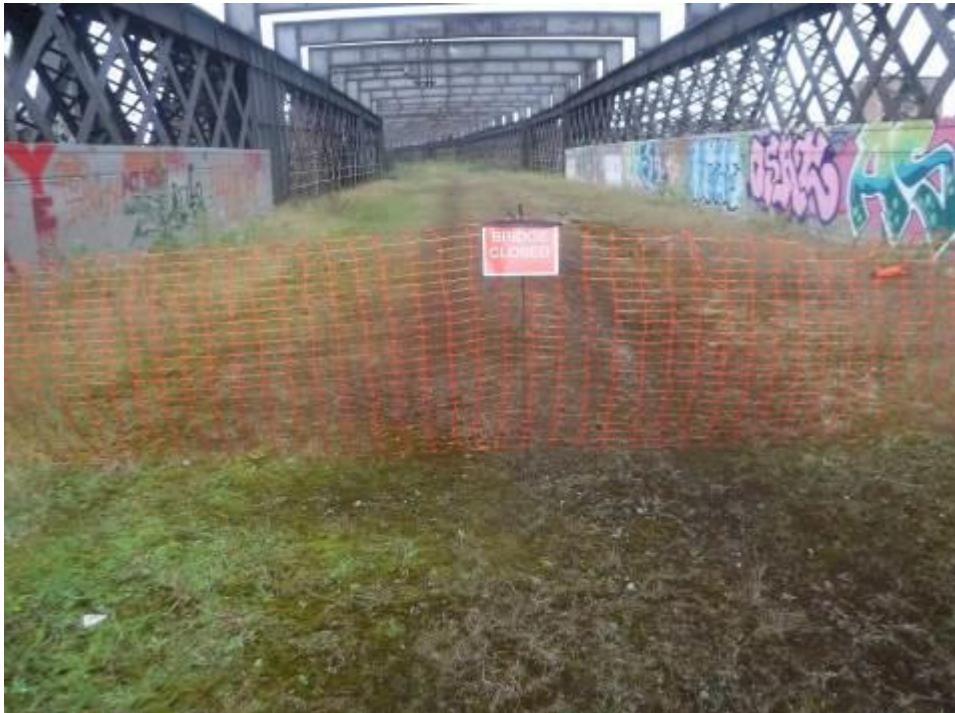
Photograph 13: Bridge closed sign employed during examination
