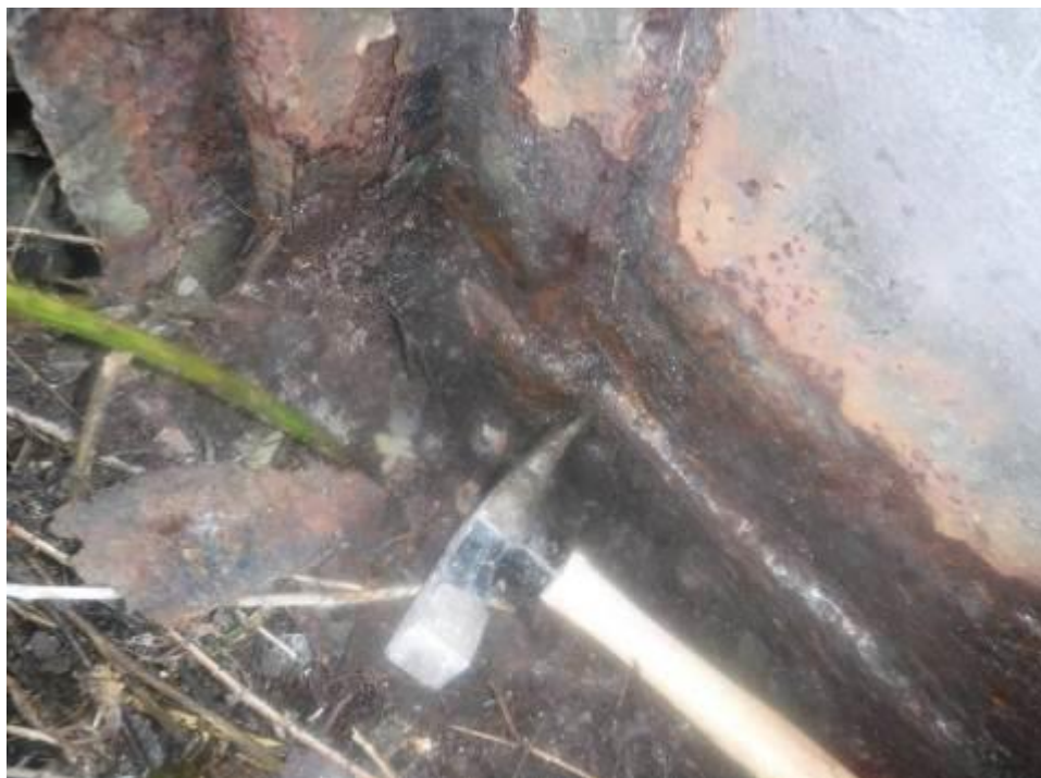
Photograph 101: Loss of thickness / delamination to base of end plate of north truss of span 2
