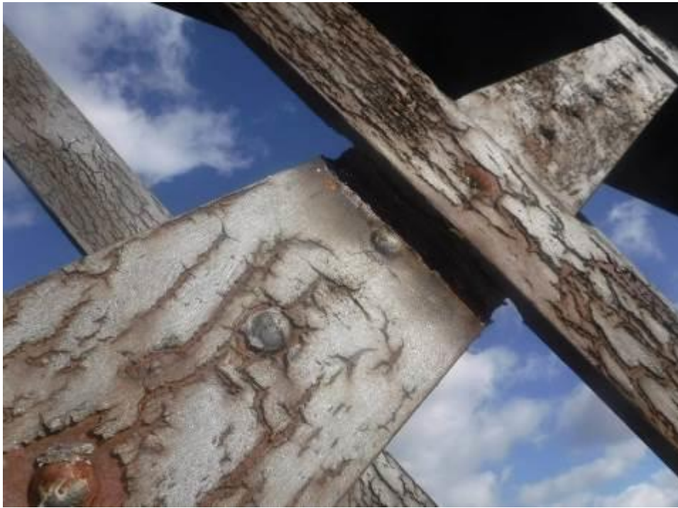
Photograph 135: Loss of thickness to diagonal bracing of north truss of span 5
