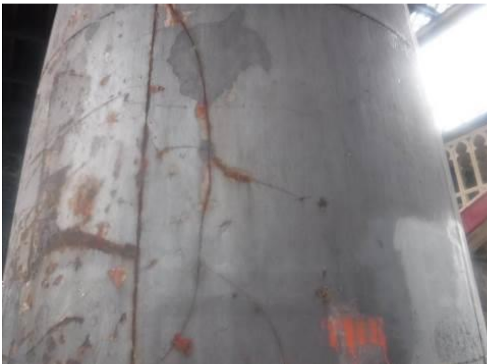
Photograph 72: Vertical branched fracture to south column of pier 4
