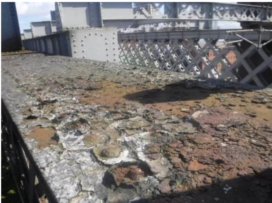
Photograph 98: Typical pitting & missing / pointed rivet heads to top flanges of top booms
