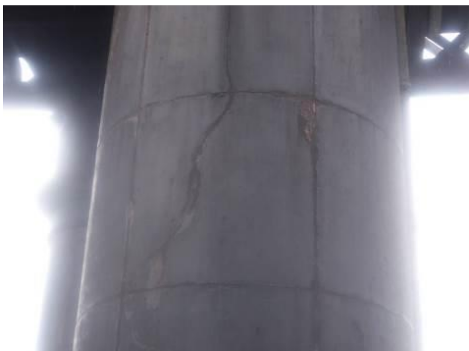
Photograph 62: Vertical & diagonal fractures to south column of pier 3
