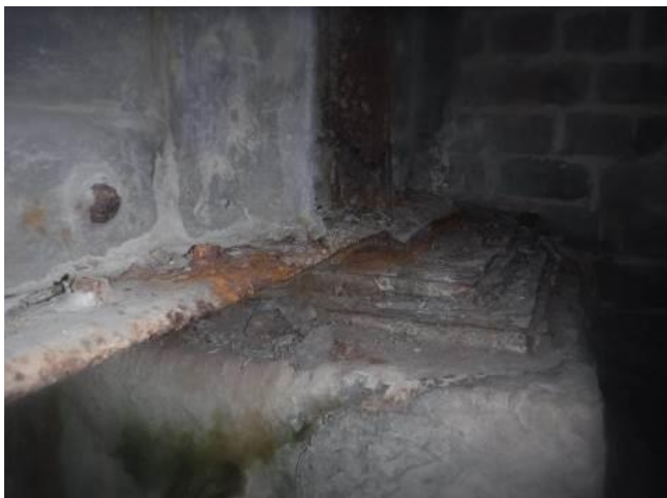
Photograph 26: Typical loss of thickness to MGI bearings of west abutment
