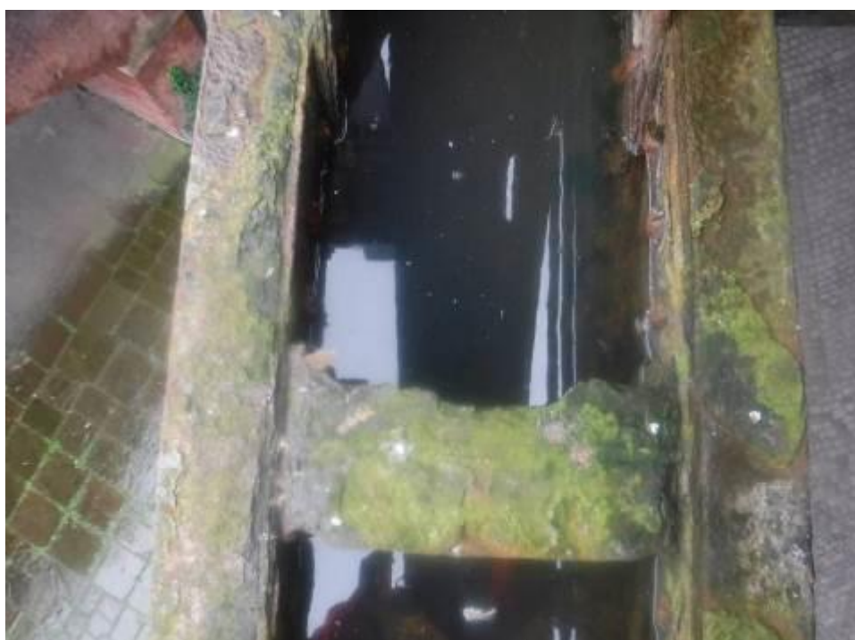
Photograph 104: Loss of section to bottom boom internal stiffener of north truss of span 2
