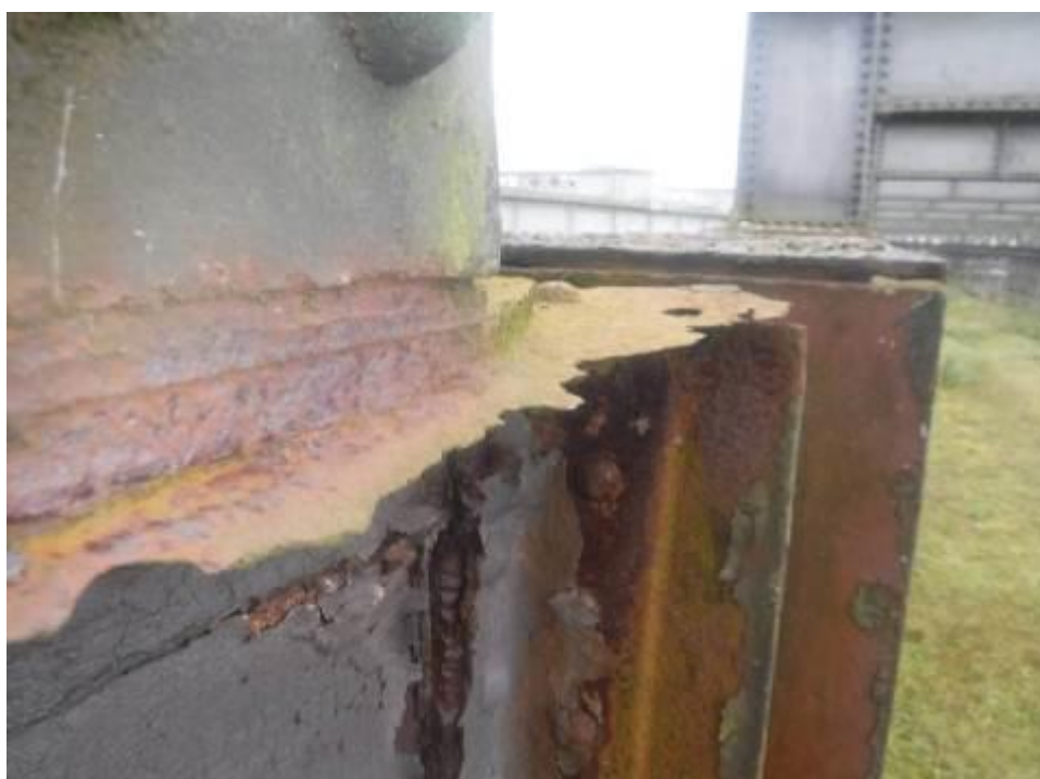
Photograph 128: Loss of section to top boom of south truss of span 4
