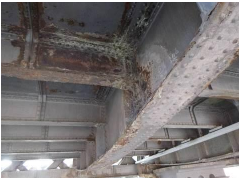
Photograph 190: Loss of thickness & pitting to MG12 & T31 of soffit of span 3
