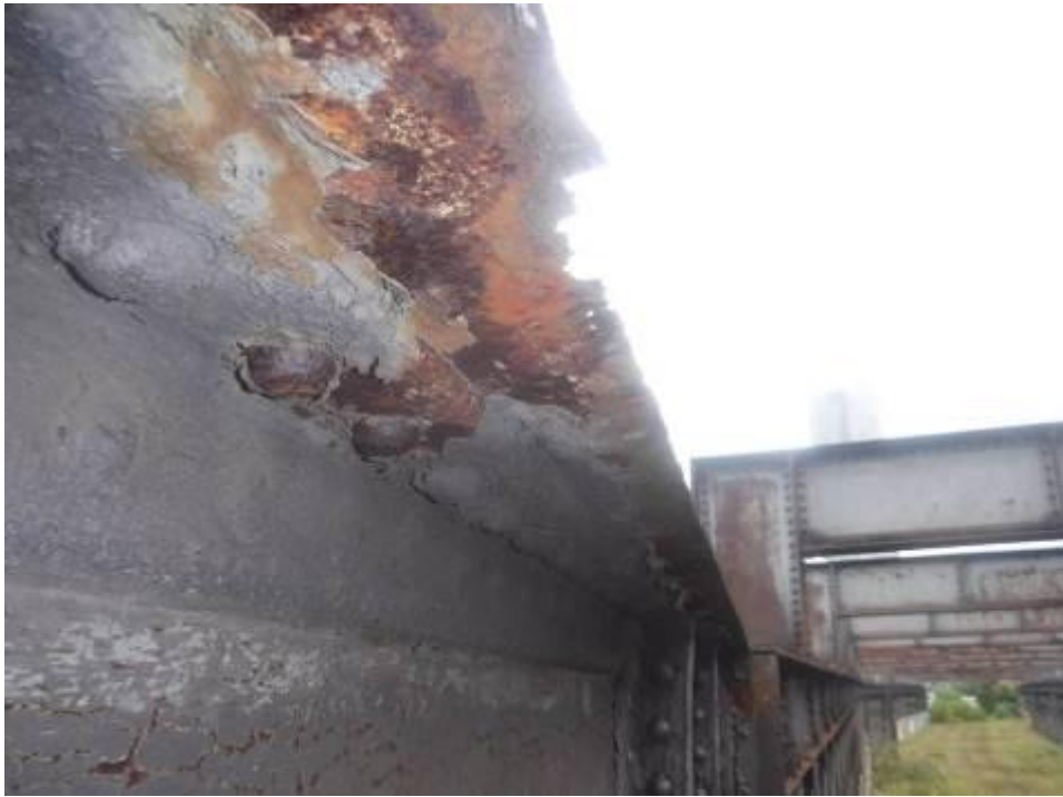
Photograph 123: Loss of section to top boom, top flange of north truss of span 4
