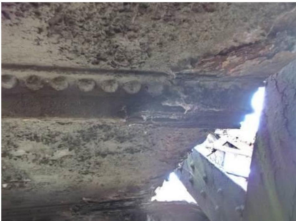
Photograph 212: Typical loss of thickness to deck stiffeners to edges of soffit of span 7
