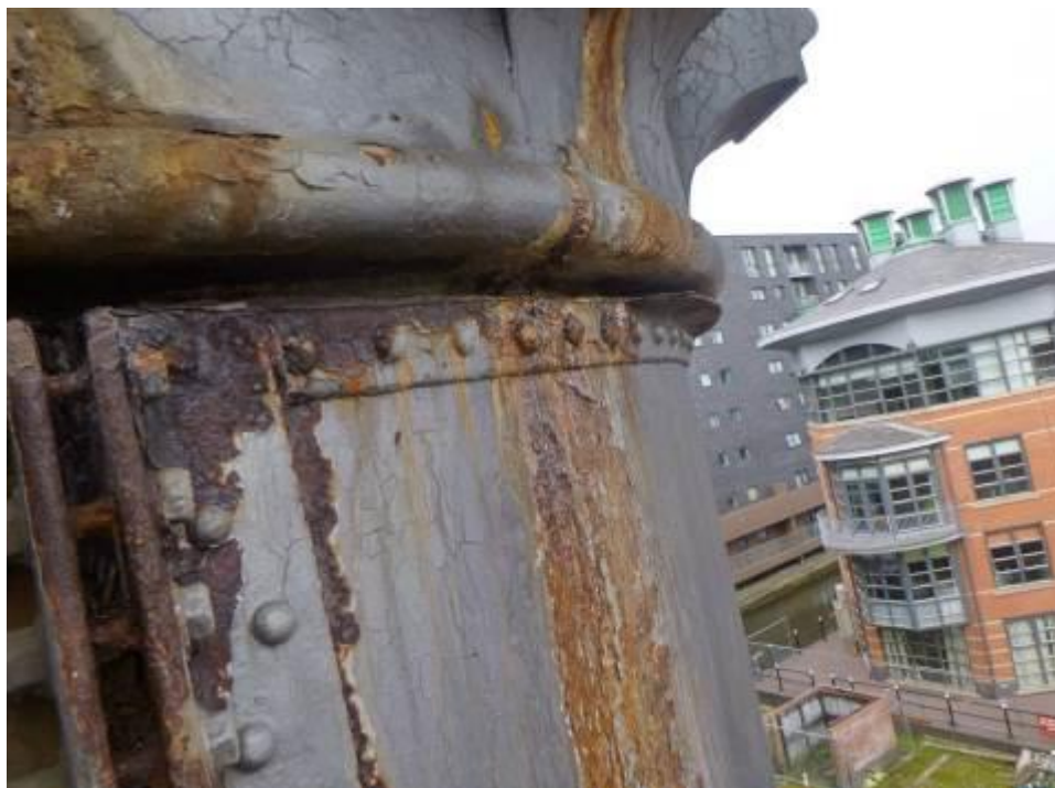
Photograph 65: Area of loss of section to upper angle of north column of pier 4
