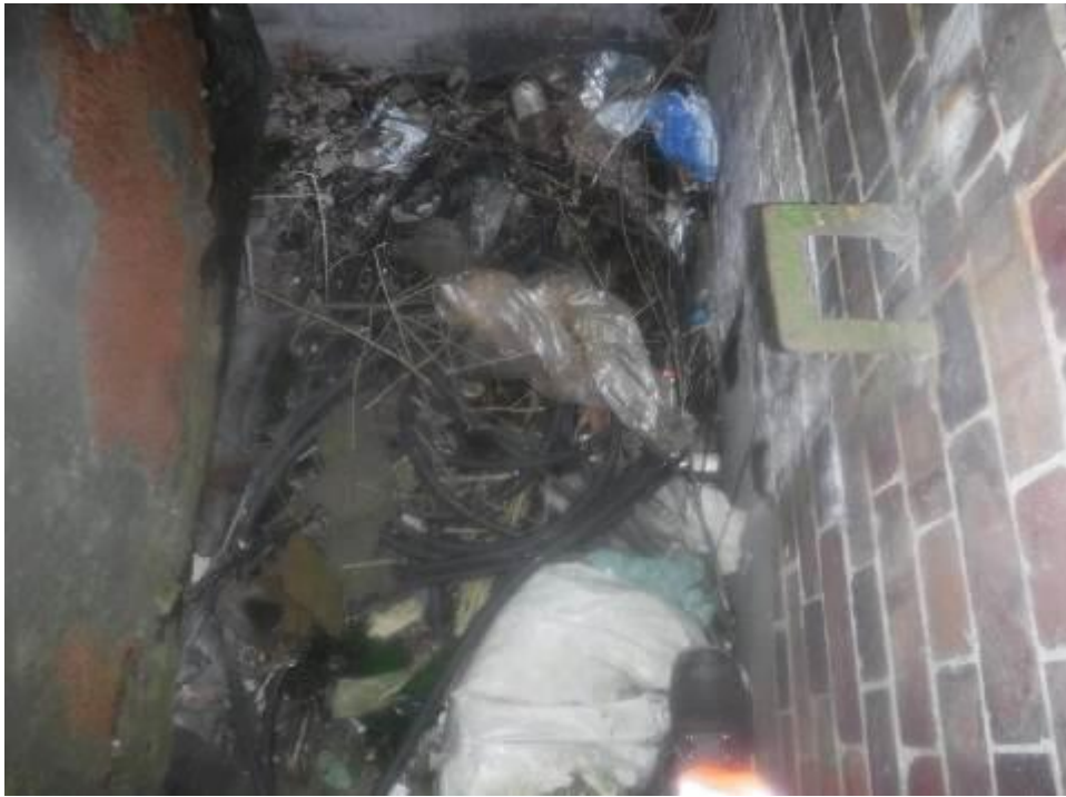
Photograph 23: Debris to bearing shelf adjacent to north bearing of west abutment
