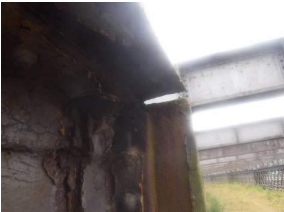
Photograph 110: Split to end plate corner of south truss of span 2
