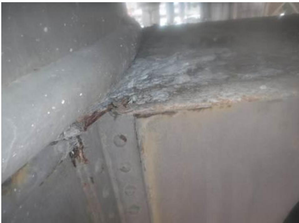
Photograph 84: Area of loss of section to interconnecting truss of pier 7
