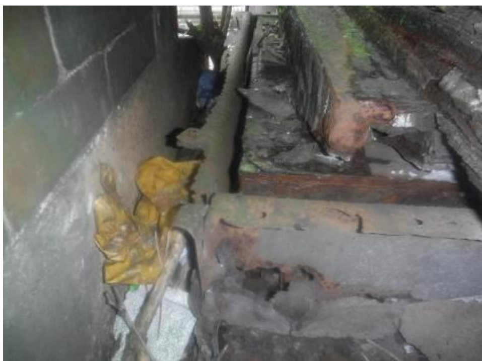
Photograph 22: Loss of thickness & loss of section to north bearing of west abutment
