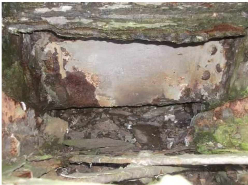
Photograph 215: Typical loss of section to MGE1 internal braces between T63 & T64 of soffit of span 7
