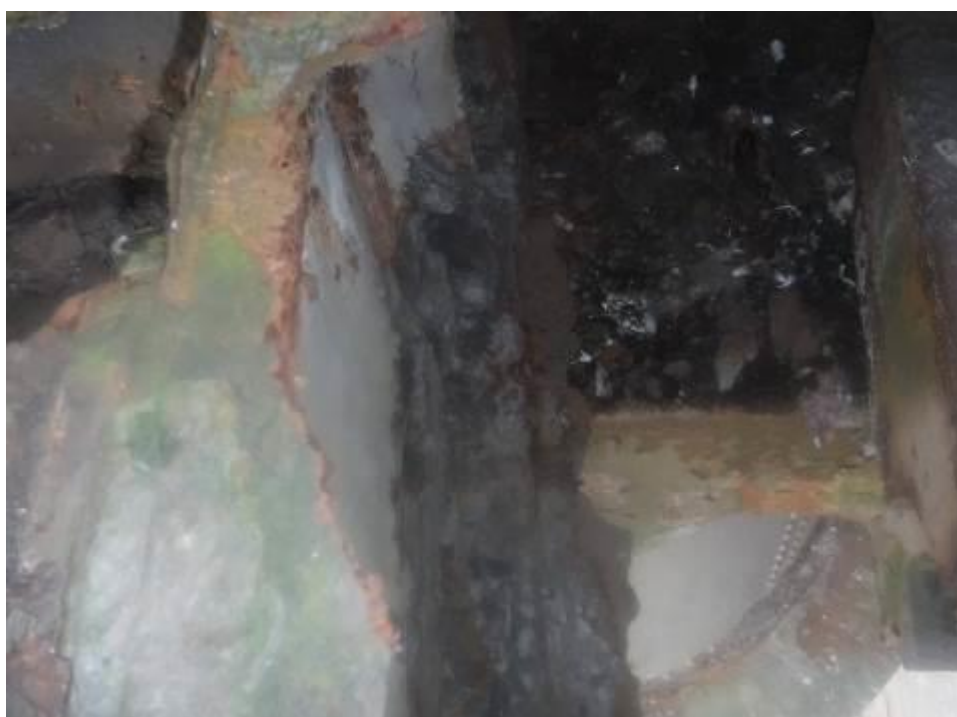
Photograph 154: Loss of section to bottom boom, top & bottom flanges of north truss of span 7
