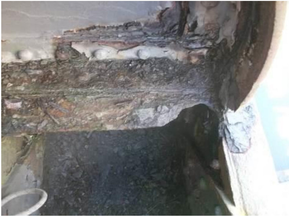
Photograph 213: Loss of section to T66 of soffit of span 7
