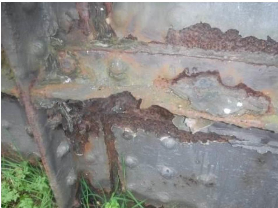
Photograph 114: Loss of section to vertical section above pier of south truss of span 2
