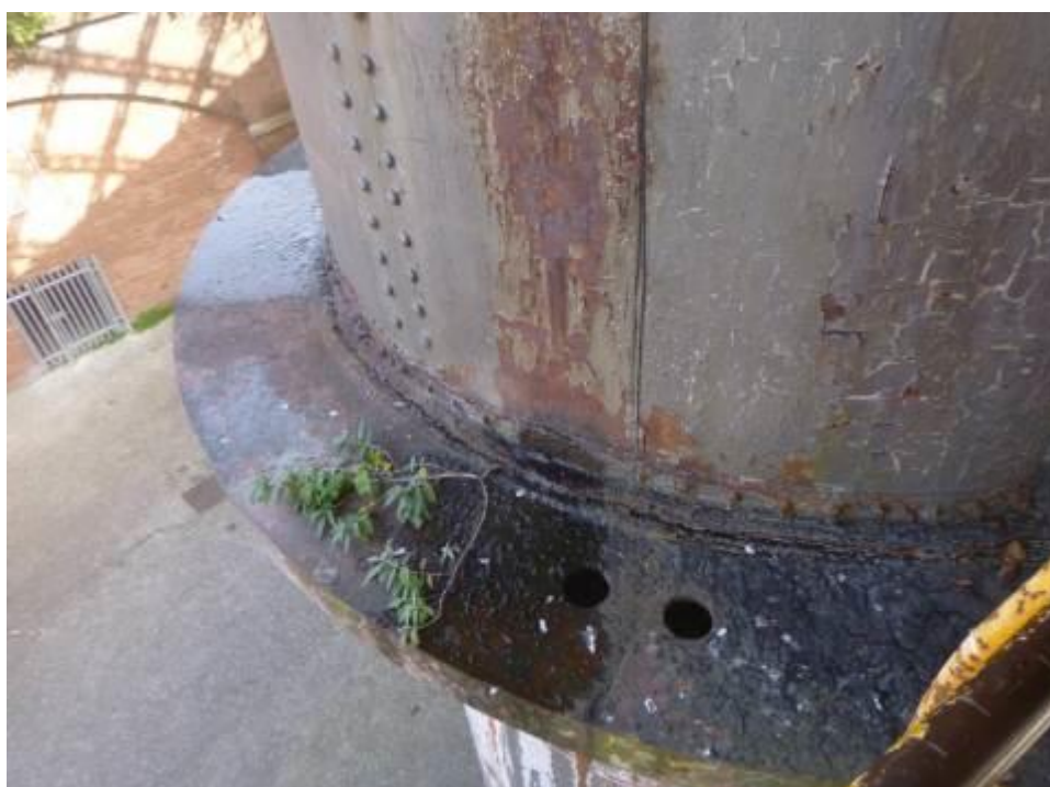
Photograph 48: Area of loss of section to lower angle of north column of pier 2
