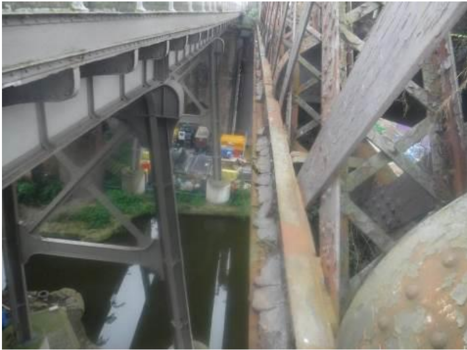
Photograph 97: Typical cracked / loose / missing mortar to bottom flanges of bottom booms
