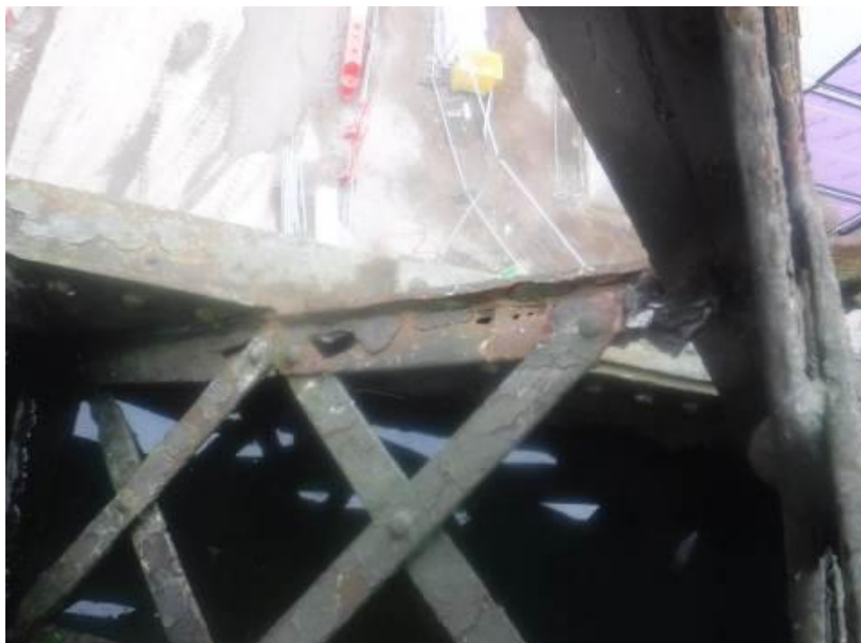
Photograph 163: Loss of section to diagonal bracing of north truss of span 8
