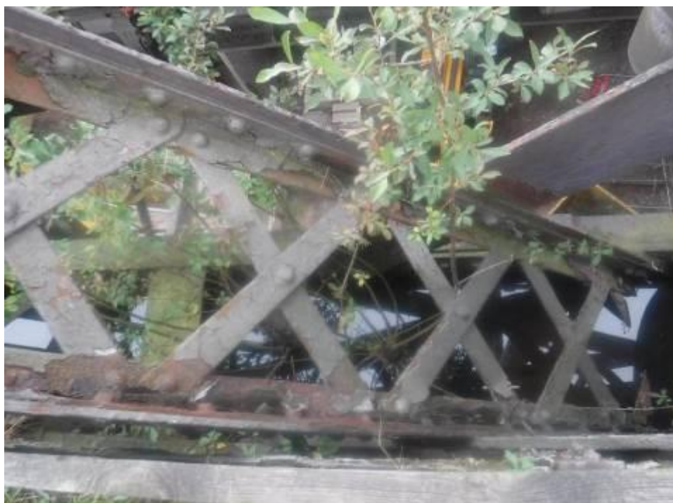
Photograph 170: Sapling growth to bottom boom of south truss of span 8
