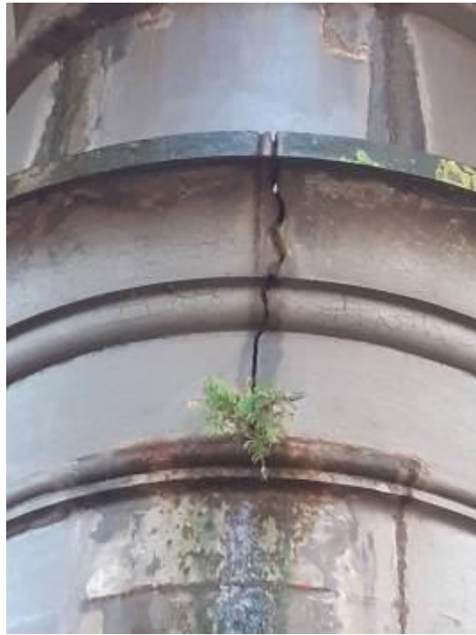
Photograph 43: Vertical fracture & vegetation growth to extra column of pier 1
