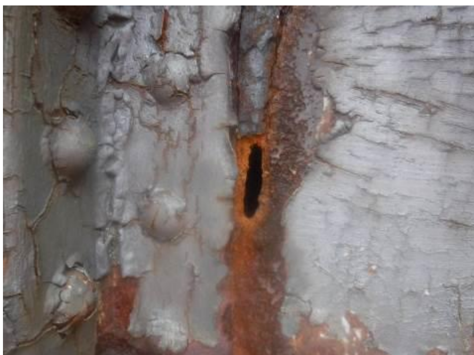
Photograph 106: Loss of section to vertical section plate of north truss of span 2
