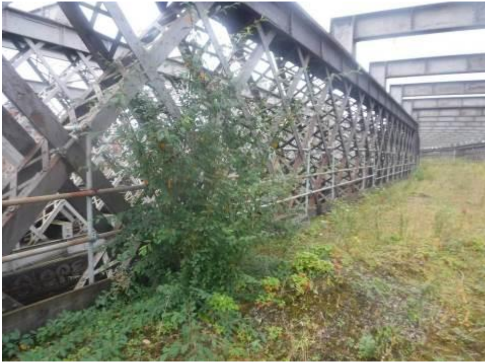
Photograph 229: Typical vegetation growth to top of deck
