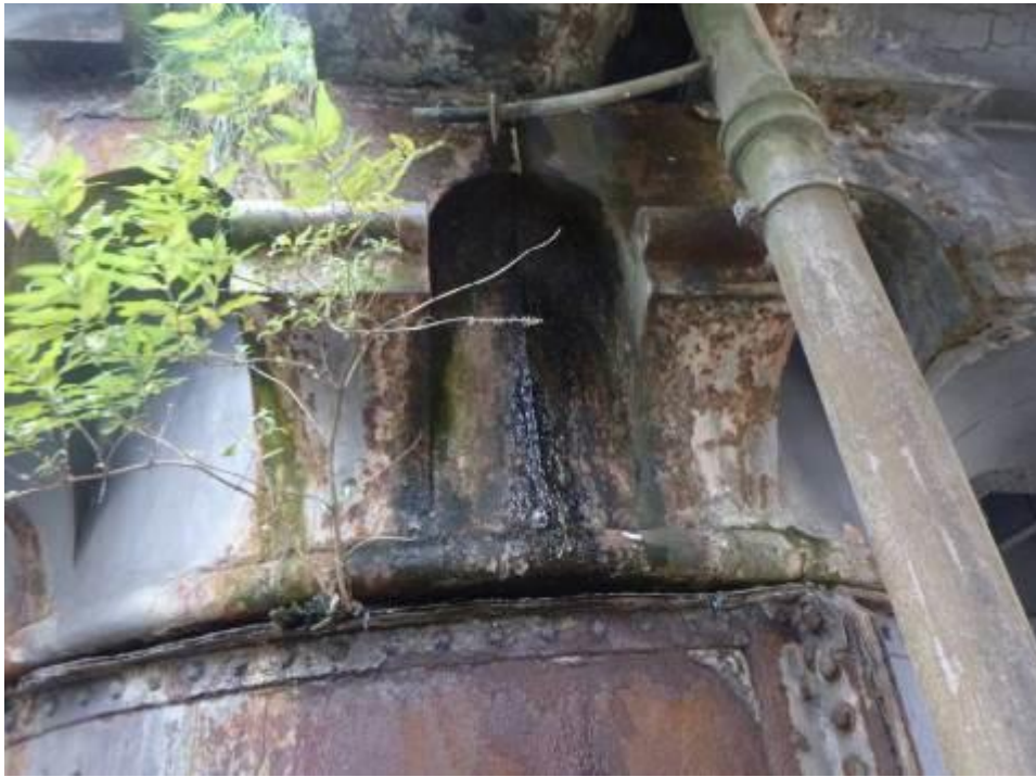
Photograph 73: Area of seepage & vegetation growth to south column of pier 4
