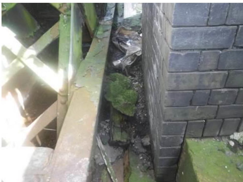
Photograph 144: Debris build-up between south truss of span 5 & adjacent structure
