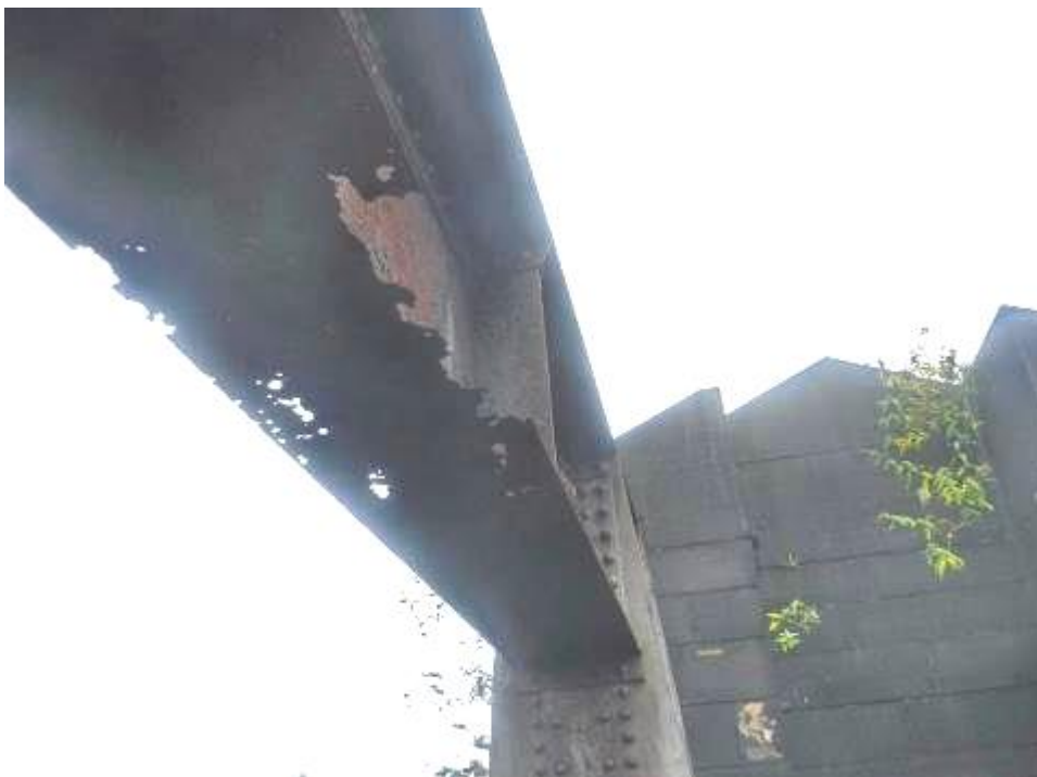
Photograph 176: Loss of section to upper transverse steelwork T1
