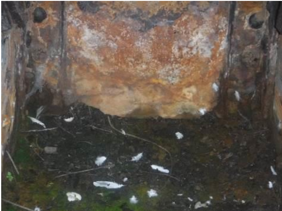
Photograph 119: Loss of thickness & section to end plate of north truss of span 3
