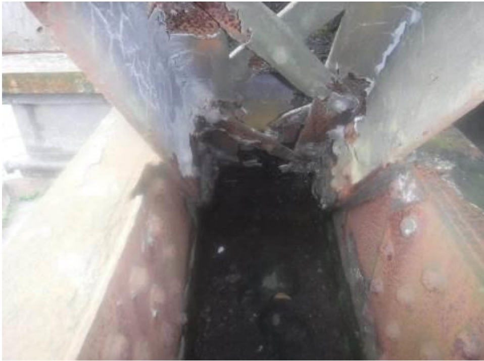
Photograph 125: Loss of section to diagonal bracing of north truss of span 4
