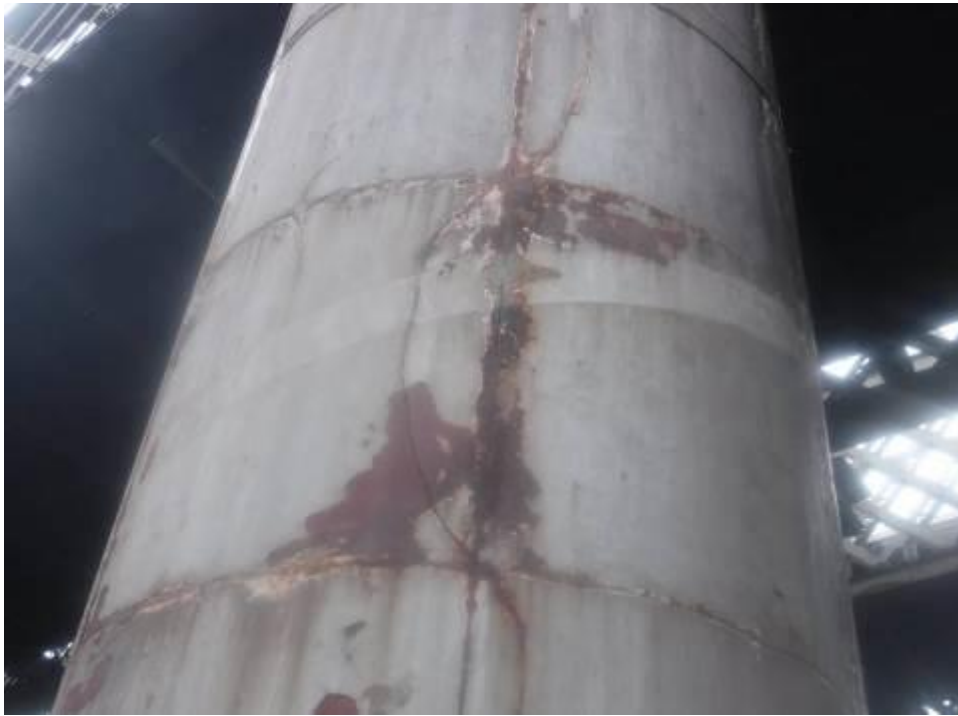
Photograph 57: Vertical fractures & loss of thickness to north column of pier 3
