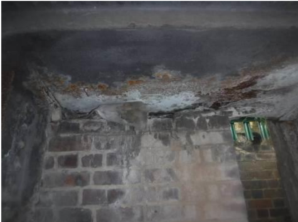
Photograph 227: Loss of thickness to deck & loose rust debris to ballast wall of soffit of span 8
