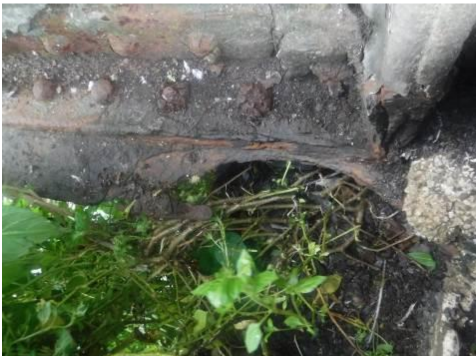
Photograph 138: Loss of section to bottom boom, bottom flange of north truss of span 5
