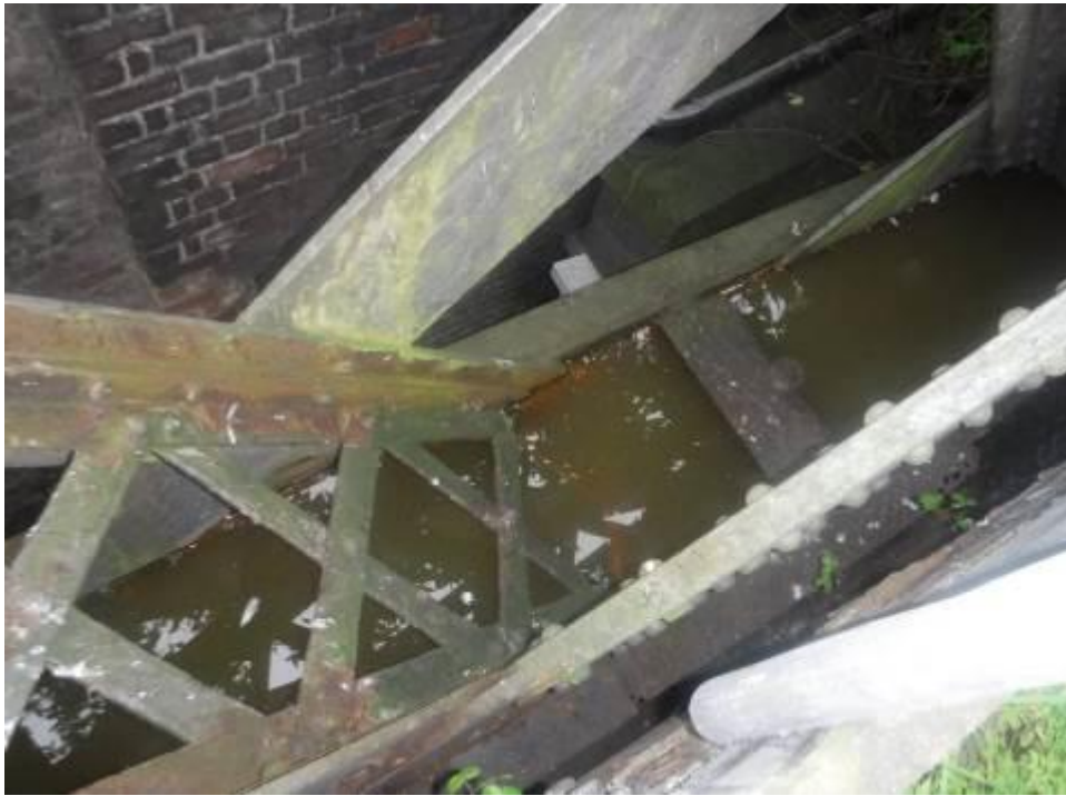
Photograph 149: Typical flooding to bottom boom of south truss of span 6
