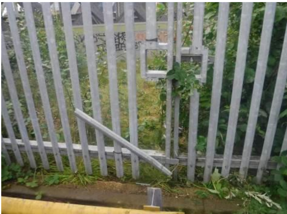
Photograph 238: Loose vertical strut to palisade fencing to east end of top of deck
