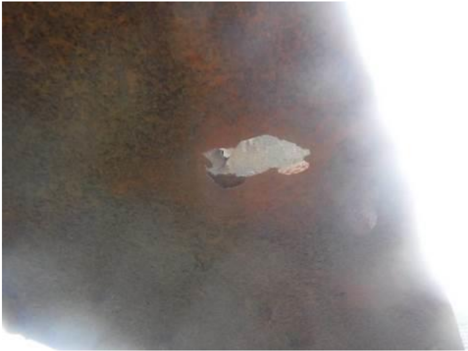
Photograph 177: Loss of section to upper transverse steelwork T21
