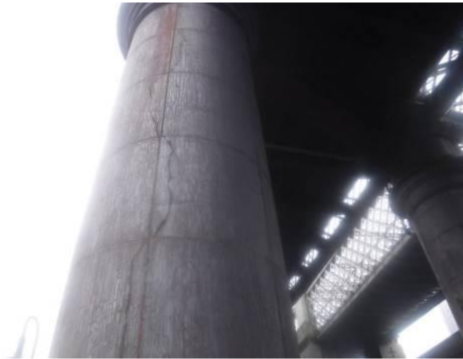
Photograph 69: Vertical fractures to north column of pier 4
