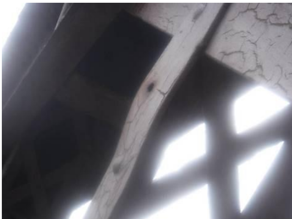
Photograph 127: Deformation & missing rivet to diagonal member of south truss of span 4
