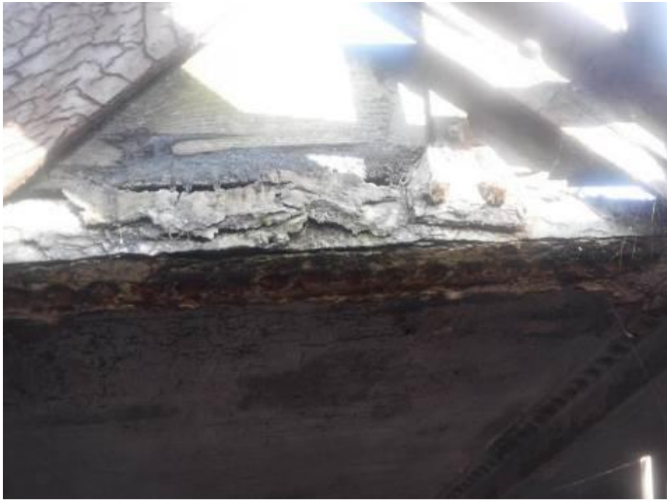
Photograph 217: Typical corrosion to deck edges of soffit of span 8
