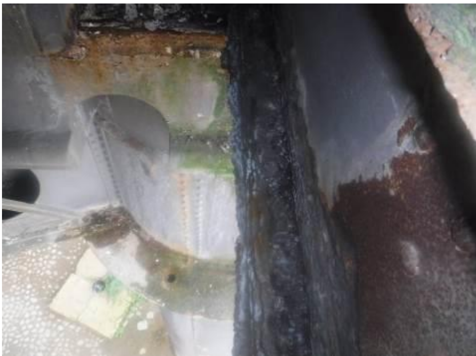
Photograph 126: Loss of section to bottom boom, bottom flange of north truss of span 4
