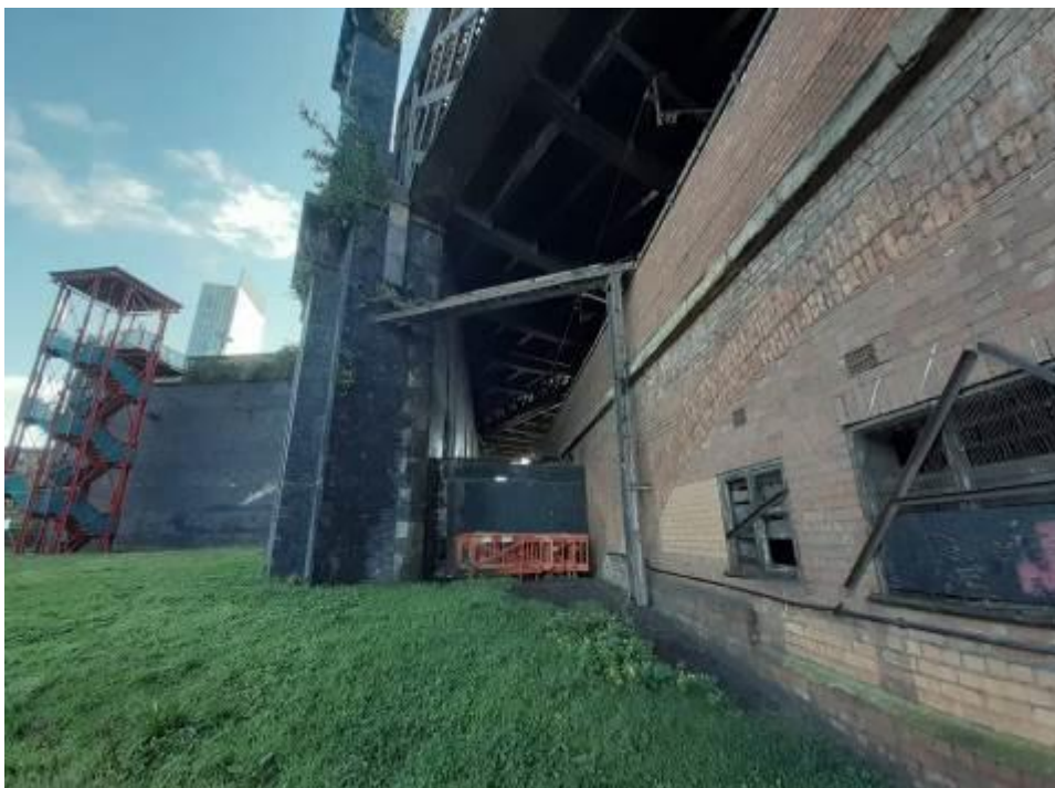
Photograph 18: Fencing blocking access to east abutment
