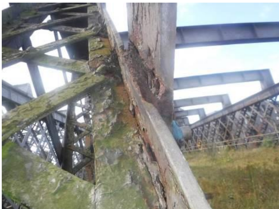
Photograph 143: Loss of thickness & rust jacking to diagonal member of south truss of span 5
