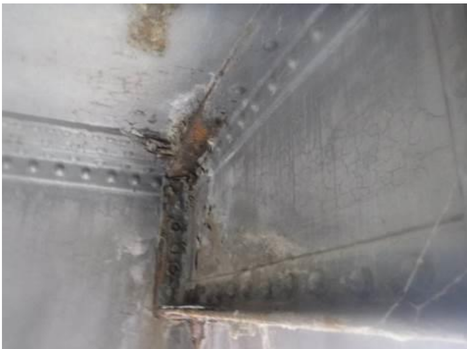
Photograph 226: Loss of thickness to MGI3 / T81 / deck of soffit of span 8
