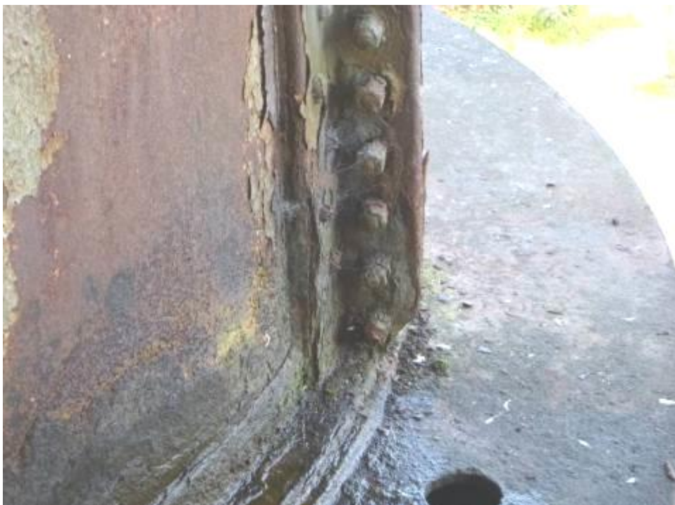
Photograph 58: Area of loss of thickness to stiffener of north column of pier 3
