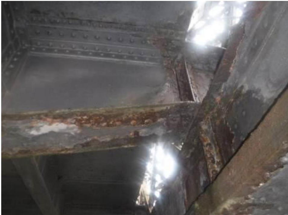
Photograph 207: Typical loss of thickness to T50 – T57 at MGE connections to soffit of span 6
