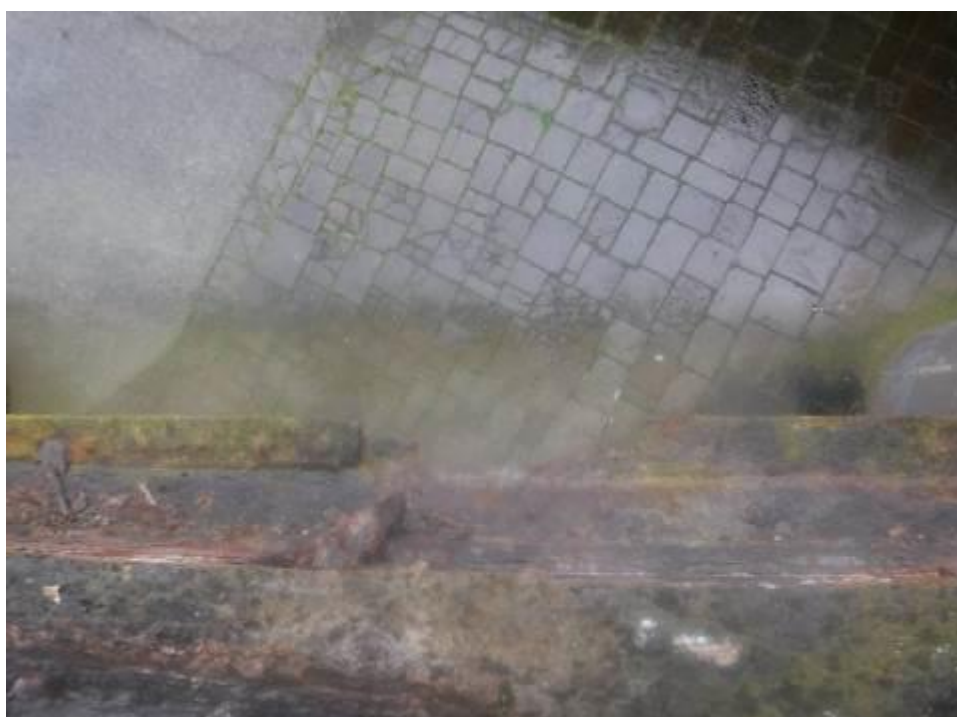
Photograph 102: Loss of section to bottom boom, bottom flange of north truss of span 2
