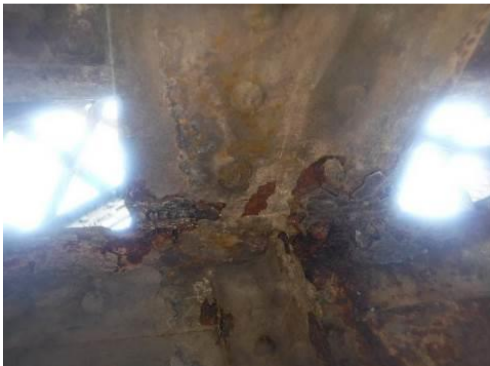
Photograph 221: Loss of section to T78 of soffit of span 8
