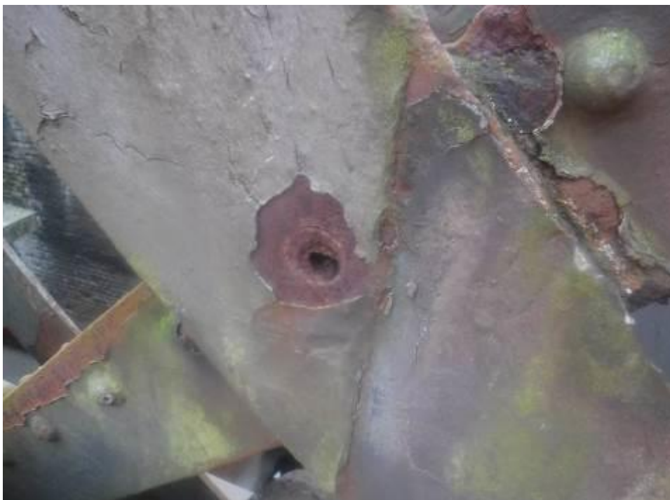
Photograph 108: Missing rivet to south truss of span 2
