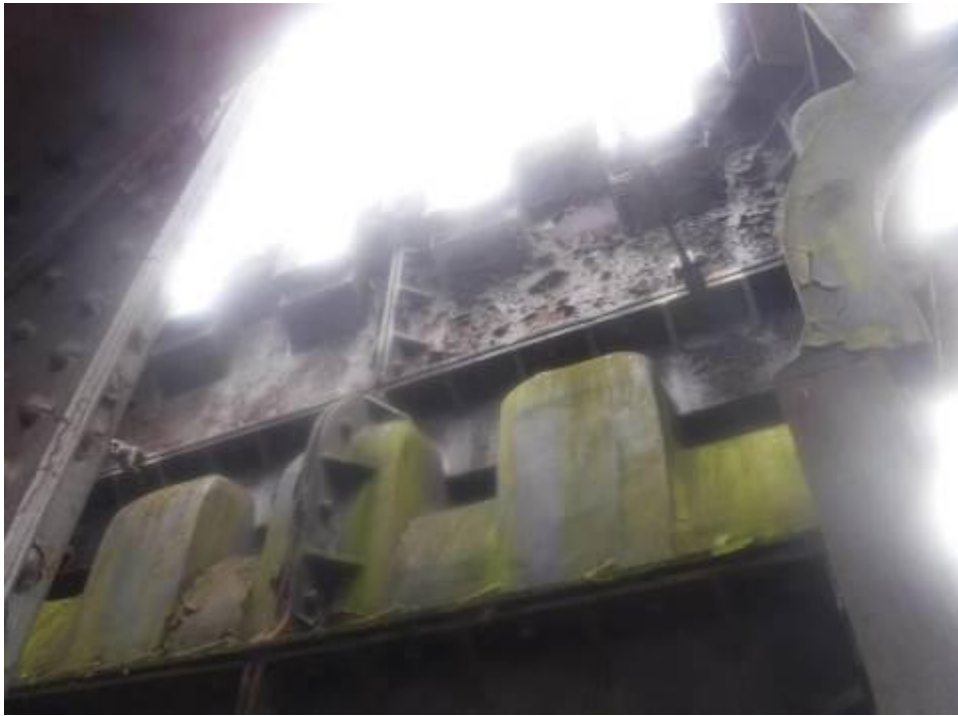
Photograph 91: Typical paint loss & surface corrosion to castle façades of piers
