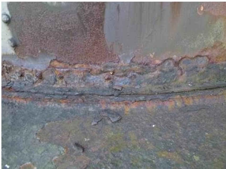
Photograph 39: Area of loss of thickness to north column of pier 1
