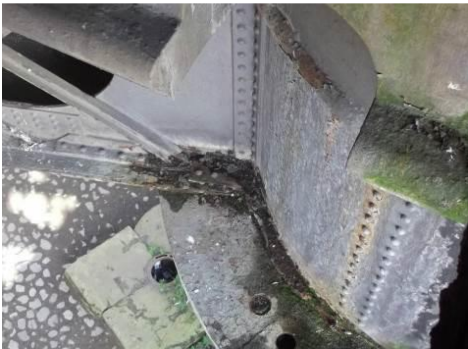
Photograph 64: Area of loss of thickness to interconnecting truss of pier 4
