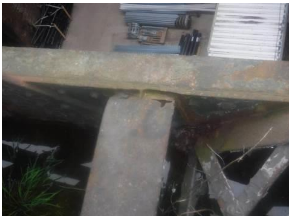
Photograph 172: Loss of section to bottom boom stiffener of south truss of span 8
