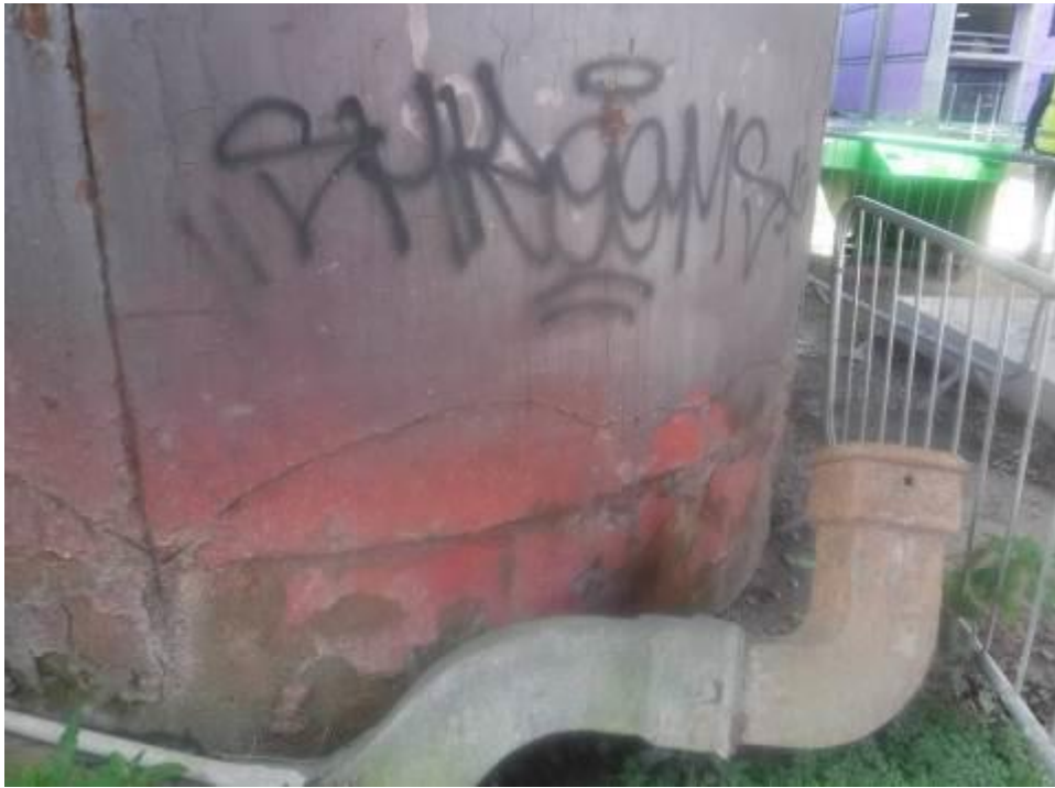
Photograph 87: Horizontal fracture to south column of pier 7
