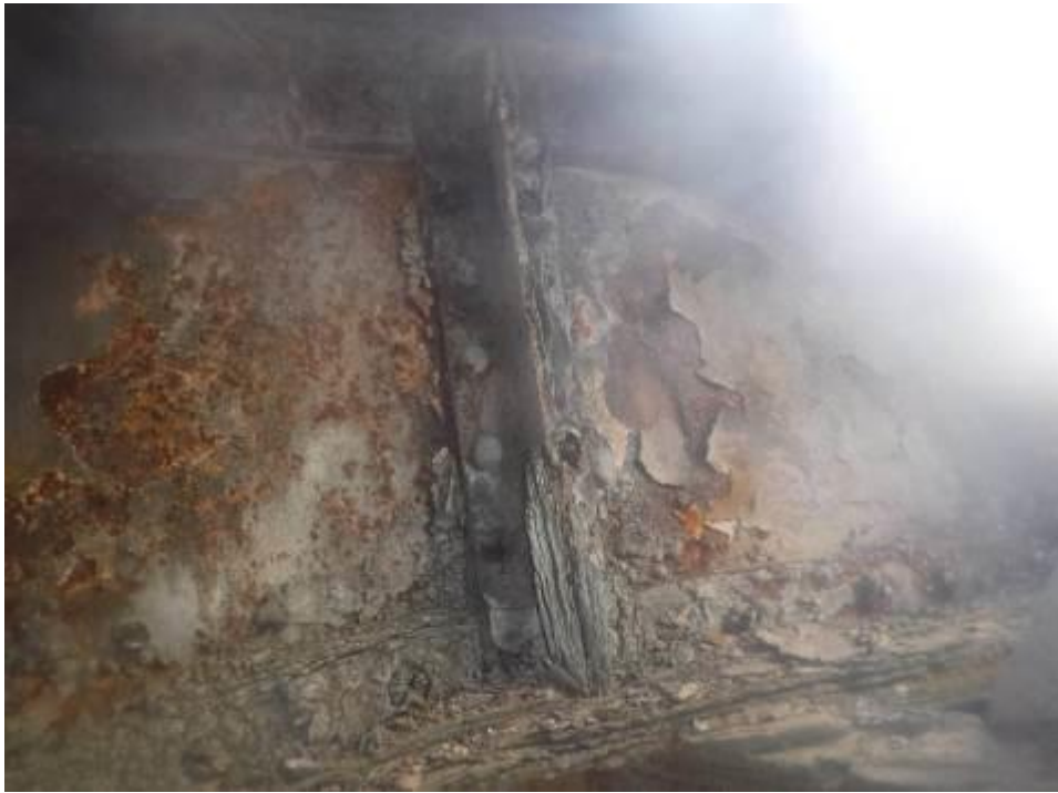
Photograph 225: Typical loss of thickness to T74 – 76 at connection with MGE1 of soffit of span 8
