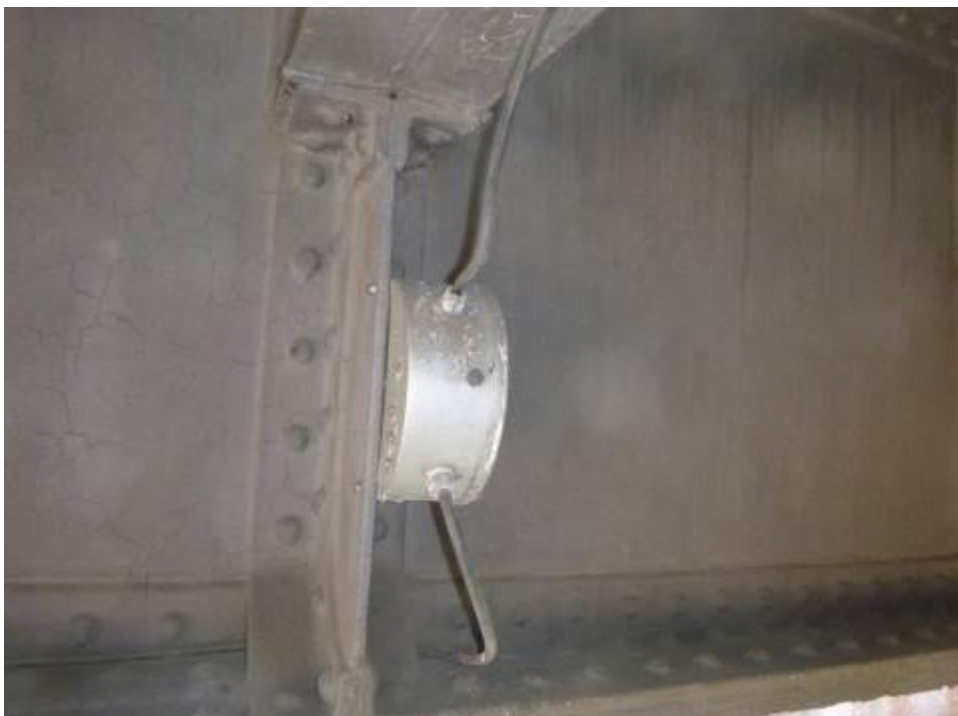
Photograph 186: Lighting junction box of soffit of span 3
