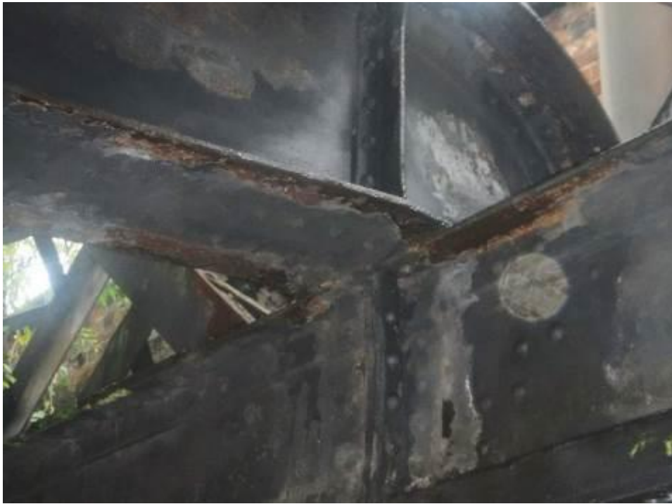
Photograph 209: Loss of thickness to T57 at MGE2 connection to soffit of span 6
