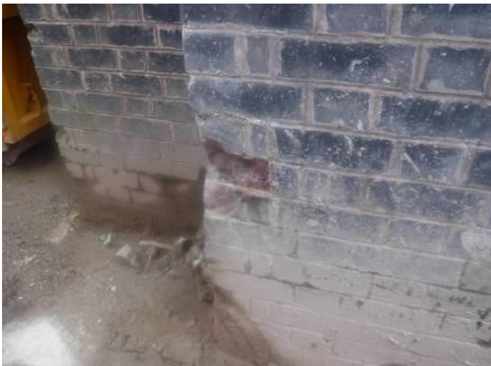
Photograph 34: Area of missing / spalled brickwork to west abutment
