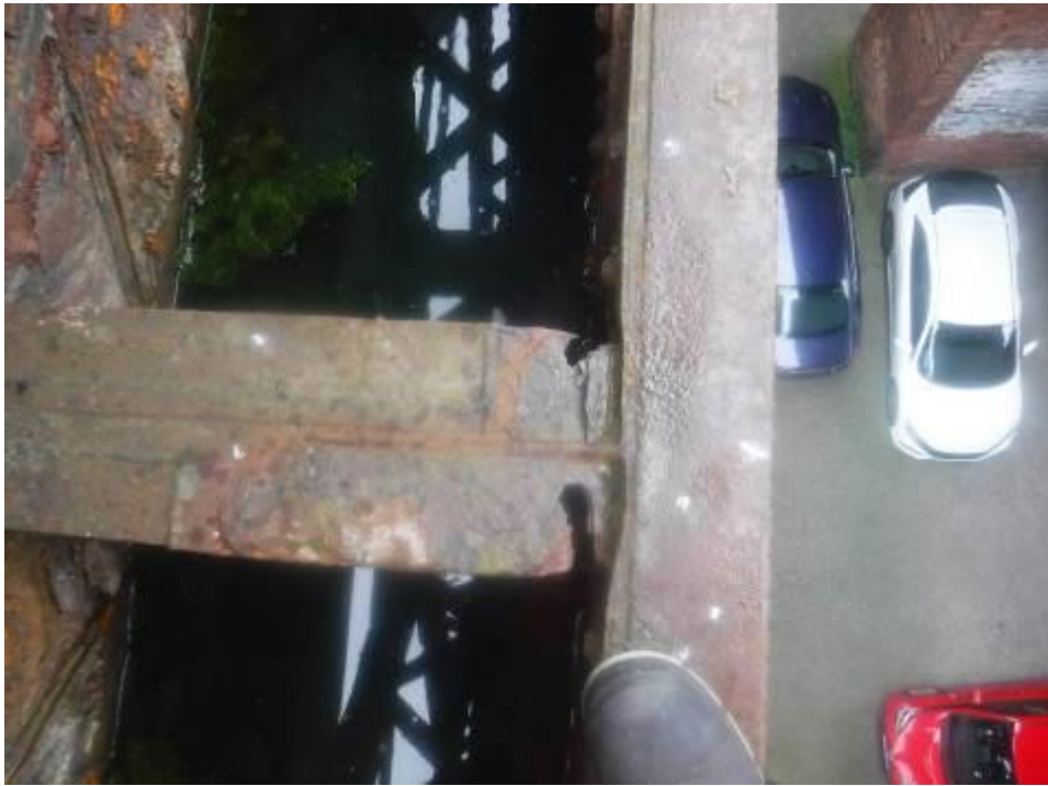
Photograph 113: Loss of section to bottom boom internal stiffener of south truss of span 2
