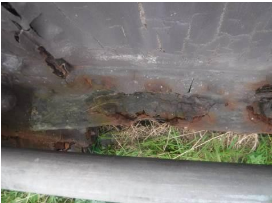
Photograph 168: Loss of thickness & section to lower web stiffener of south truss of span 8
