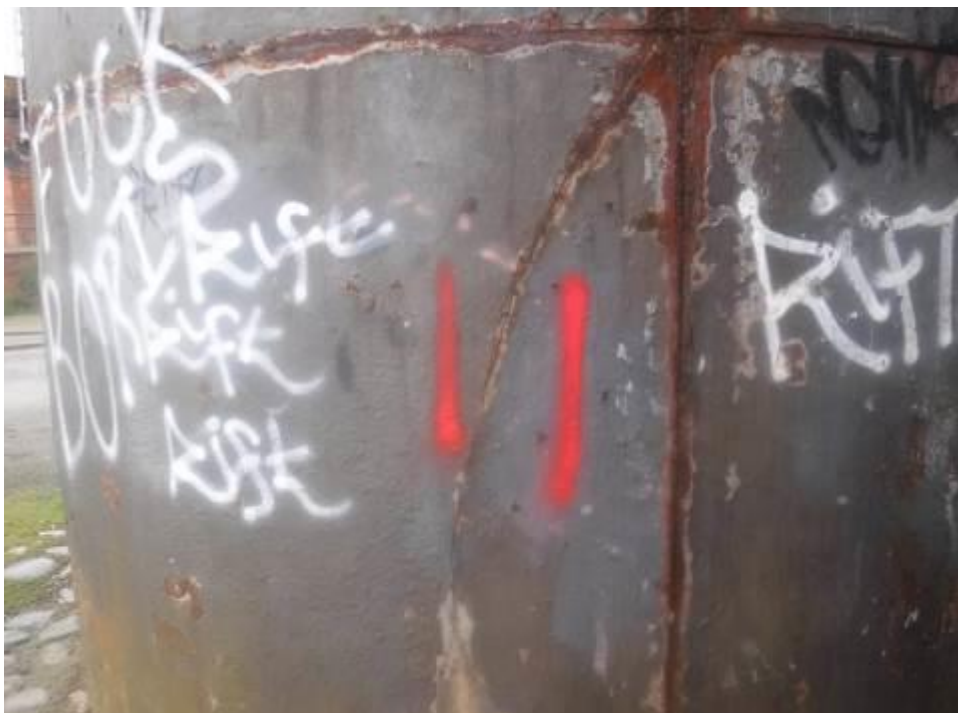
Photograph 54: Graffiti & diagonal fracture to north column of pier 3
