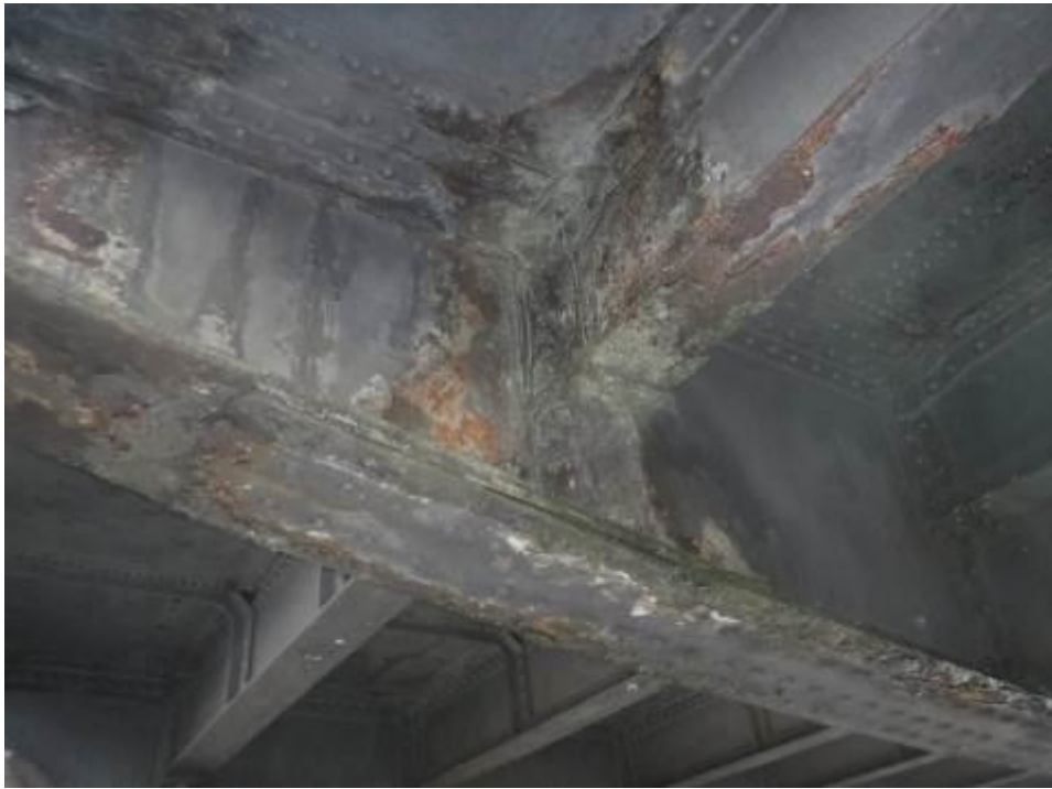
Photograph 203: Paint loss & surface corrosion to MGE1 & T45 connection to soffit of span 5
