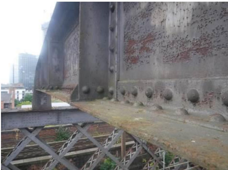
Photograph 174: Typical corrosion & pitting to webs of upper transverse steelworks
