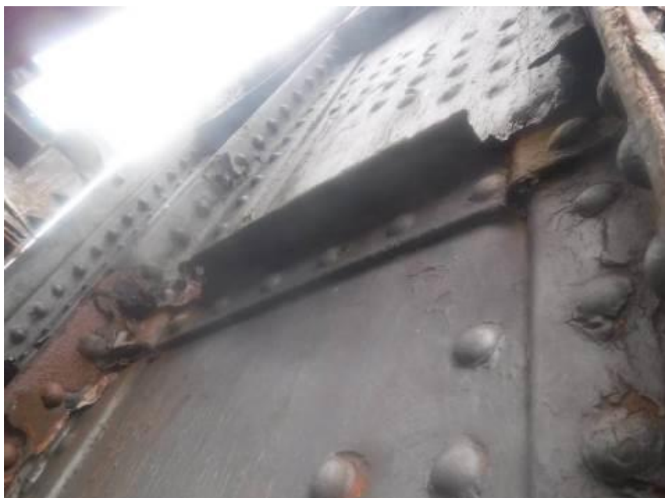
Photograph 153: Loss of section to end section upper horizontal stiffener of north truss of span 7
