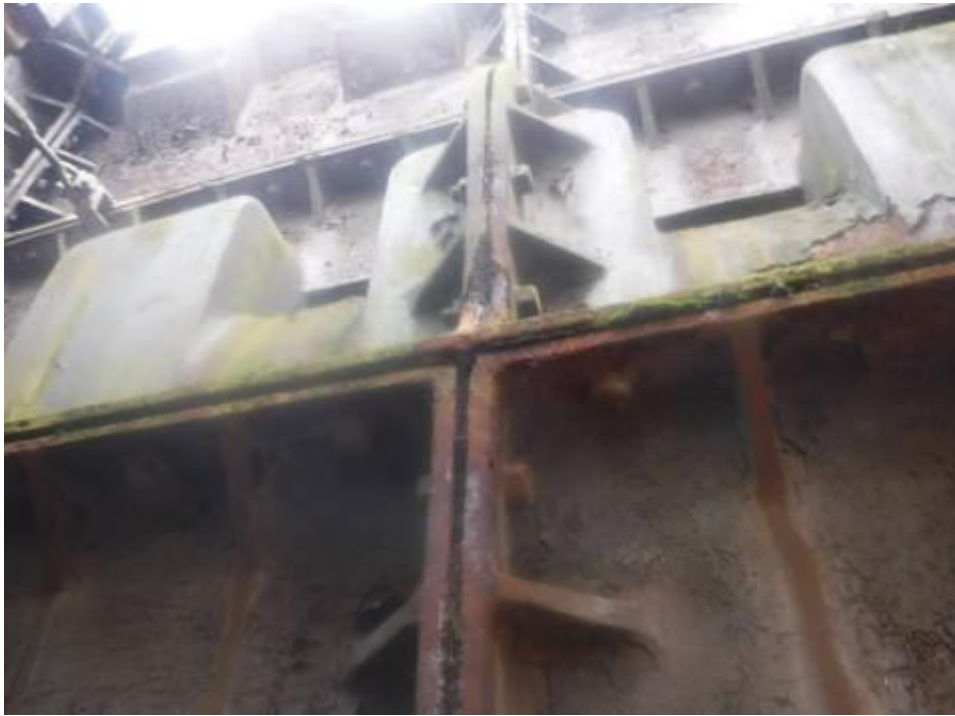
Photograph 93: Typical loss of thickness & rust jacking to panel joints of castle façades to piers
