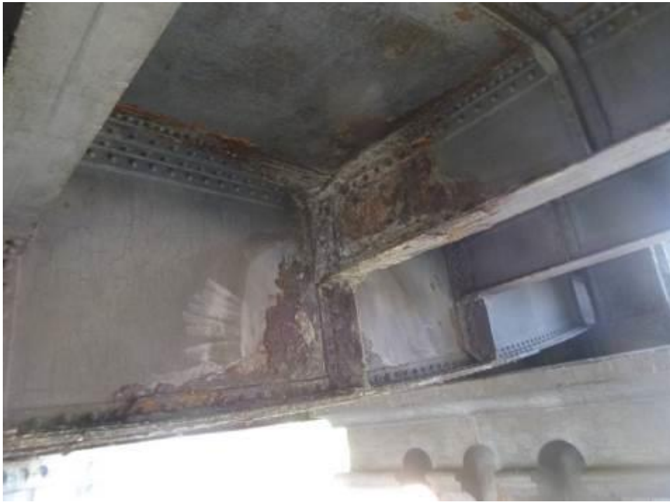
Photograph 199: Loss of thickness to T33 & section to MGI2 of soffit of span 4
