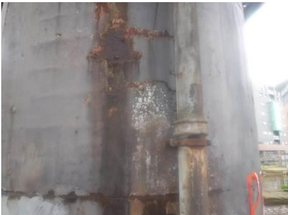
Photograph 74: Area of loss of thickness & vertical fracture to south column of pier 4
