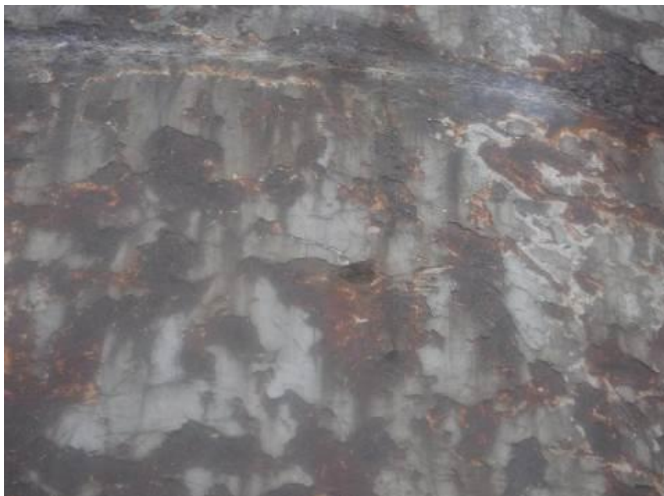
Photograph 47: Area of loss of thickness to north column of pier 2
