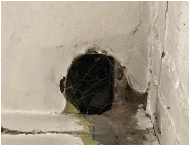
Figure 5 Photograph showing existing holes within ground floor slab
