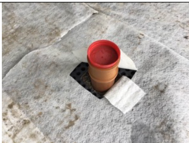
Venting cut around pipe penetration
