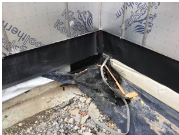
Damage and unsealed in corner
