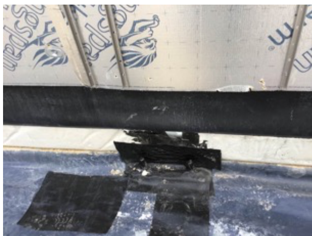
Stanchion seal using SAGM
