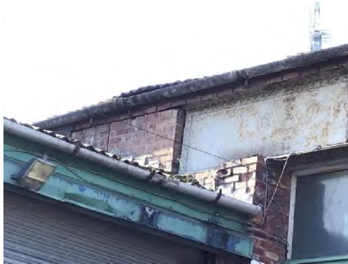
PLATE 14 SHOWING MOVEMENT CRACKS ON EXTERIOR WALLS
