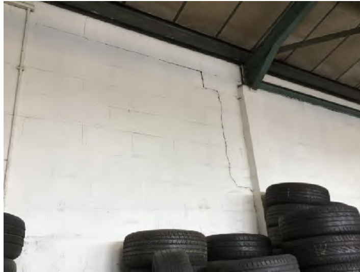
PLATE 5 SHOWING MOVEMENT CRACKS ON INTERIOR WALLS
