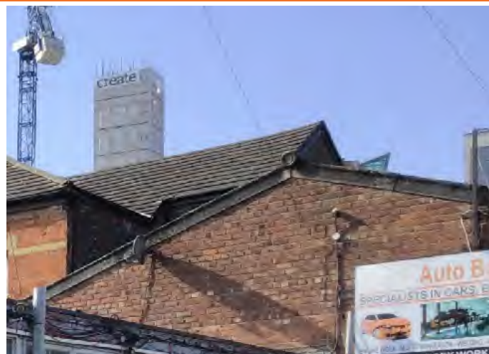
PLATE 11 SHOWING ASBESTOS SHEETING BARGE BOARD
