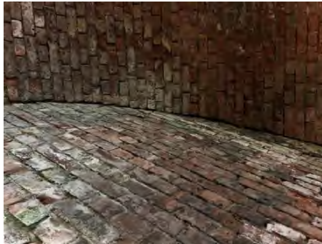
PLATE 21 SHOWING CREVICE IN BRICKWORK
