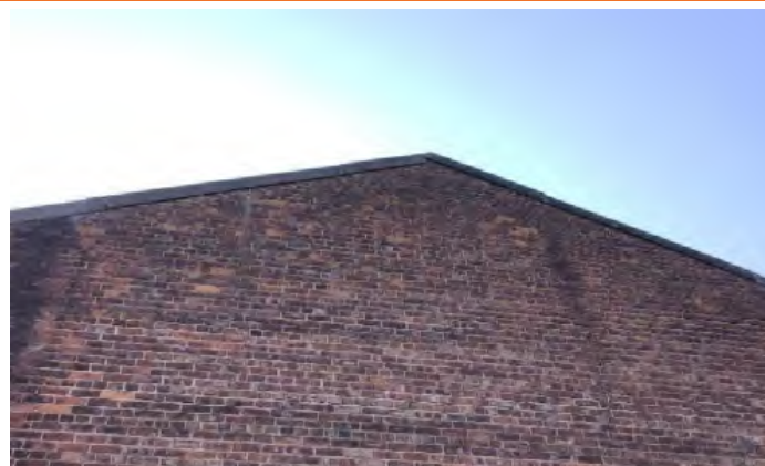
PLATE 13 SHOWING ASBESTOS SHEETING BARGE BOARD
