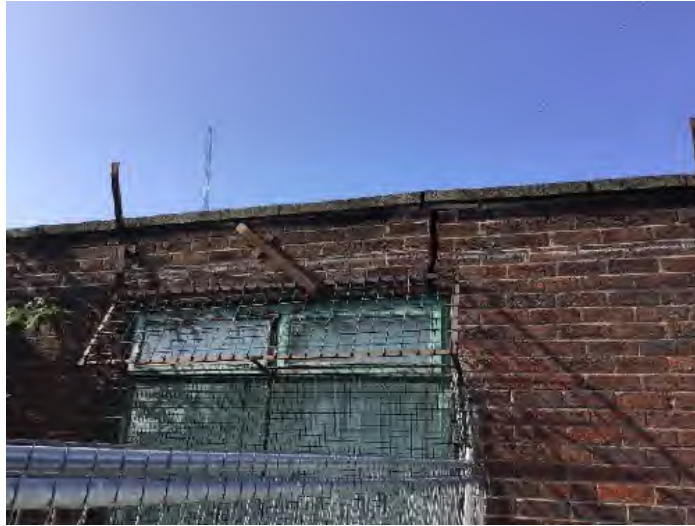
PLATE 7 SHOWING CREVICE AROUND WINDOW
