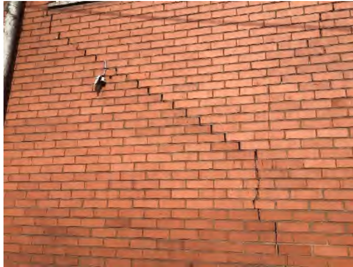
PLATE 3 SHOWING MOVEMENT CRACKS ON EXTERIOR WALLS
