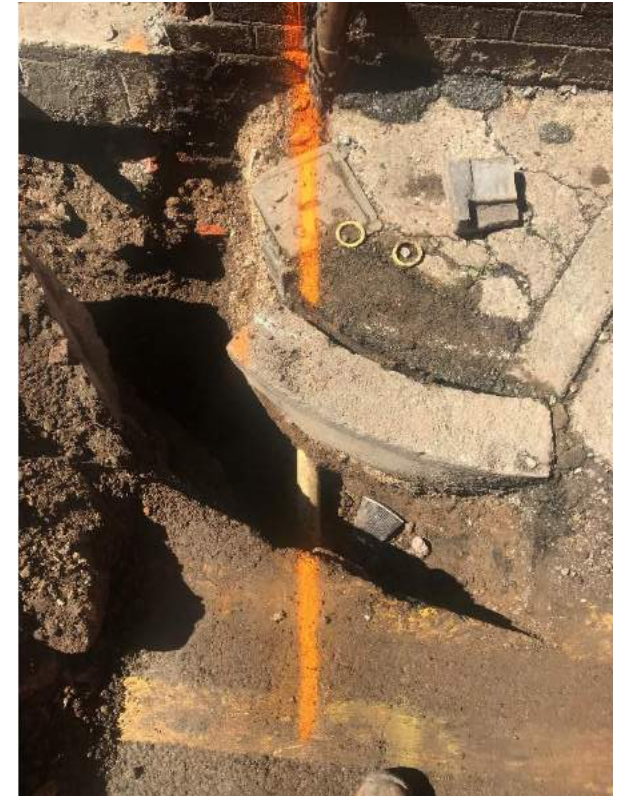
Curb to the north with gas pipe – facing West
