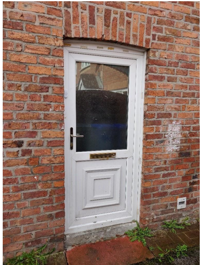
uPVC door to north elevation
