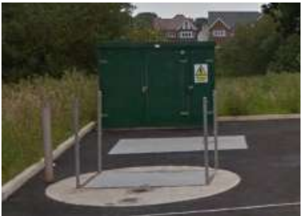
Similar existing pump station without fencing
