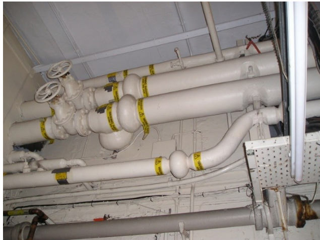
An example of thermal insulation in good condition installed to M&E services
