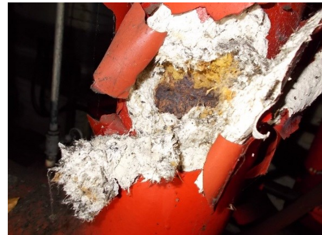
An example of thermal insulation in poor condition in situ
