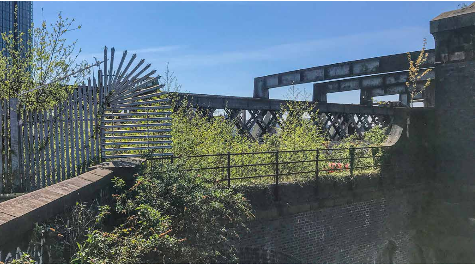
Photo of existing, inadequate guarding
