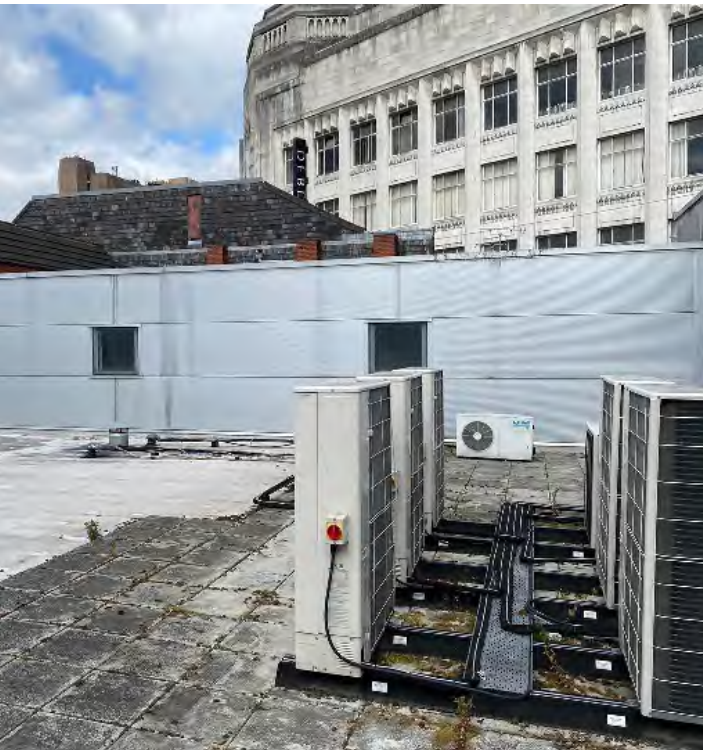
Rooftop plant area, with the Rylands Building behind
