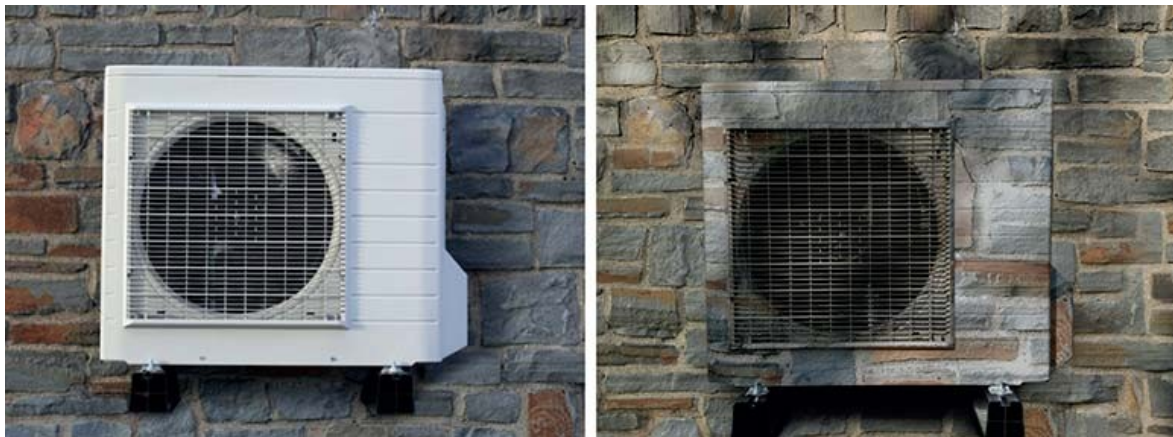
Example image of a vinyl wrap to external plant equipment.
