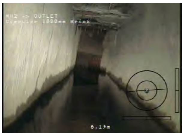
1, 00:04:53, 6.13 m Attached deposits, encrustation from 7 o'clock to 5 o'clock, 10% cross-sectional area loss
