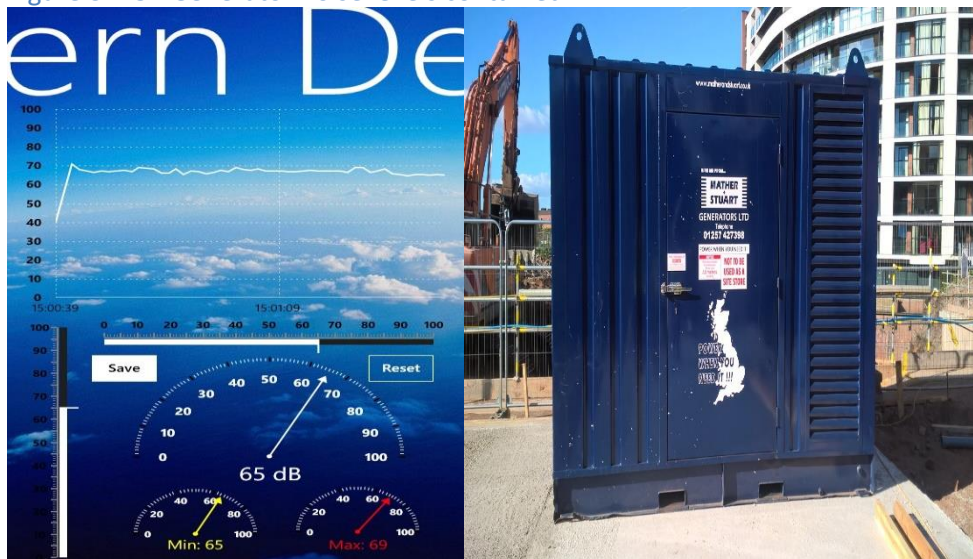
Figure 3.4.8 - Generator noise levels contained.
