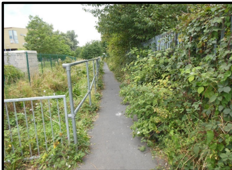
Photograph 3-12: Overgrowth observed along combined Cycle and Footway September 2021
