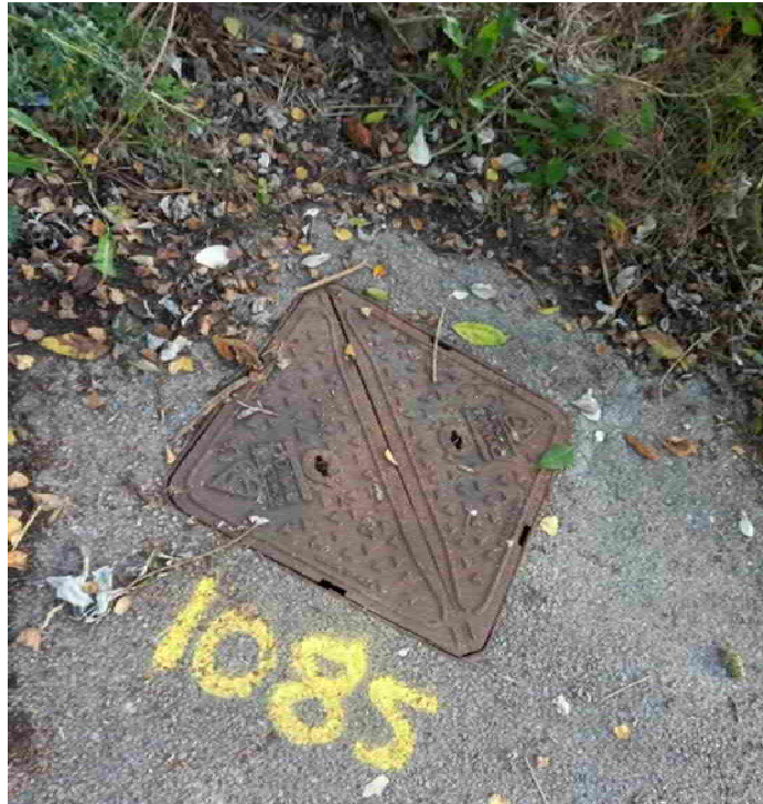
Photograph 3: View of one of the man holes located in the site.
