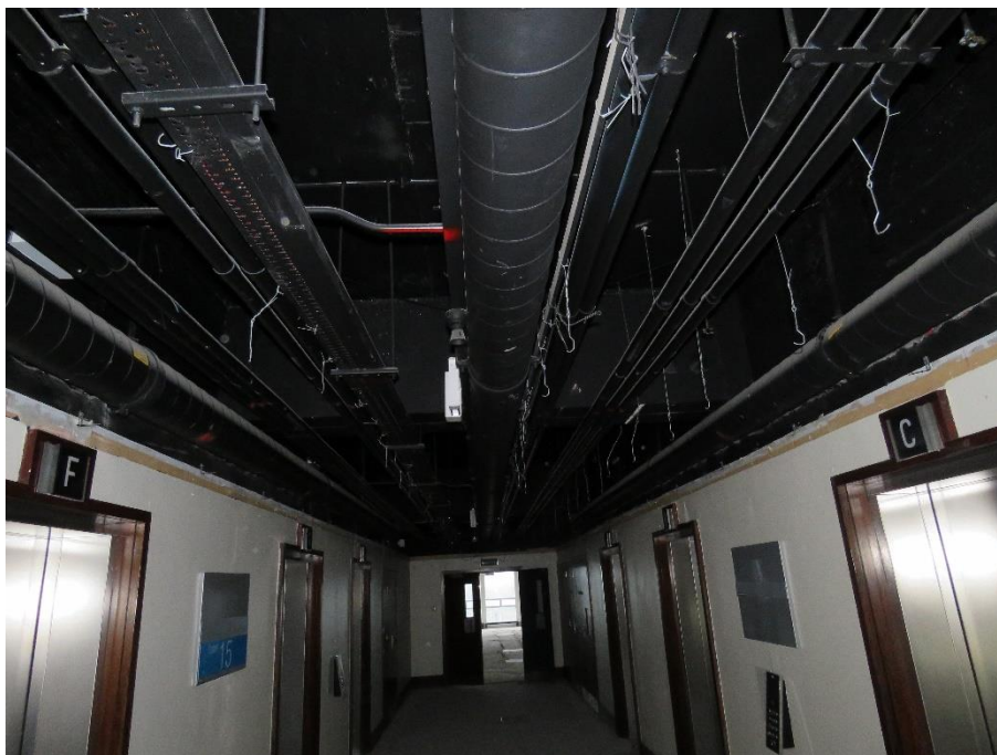
15.01 Looking along the lift lobby with now exposed services, unusually, the services have all been painted out black as you would find in a modern office development but have never been known to have been exposed.
