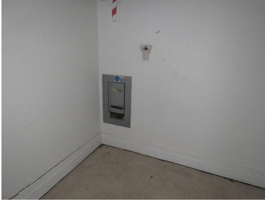
15.10 View of the Telelift outlet.
