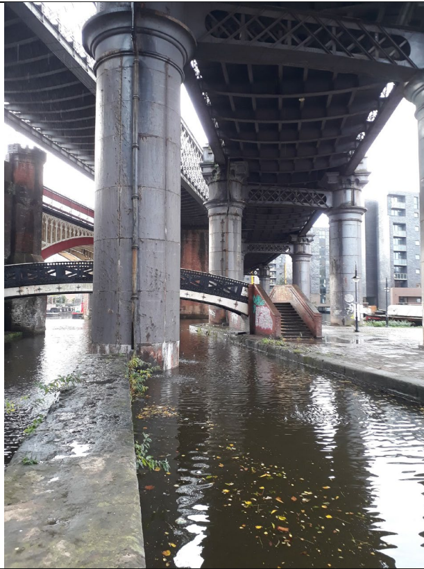
Photographic Plate No. 04: Post rainfall - noting water dropping from viaduct structure and at top of downspout
