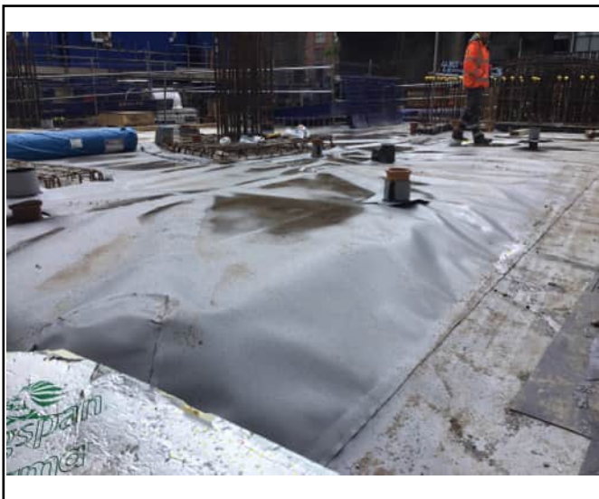
Overview of verified installation
