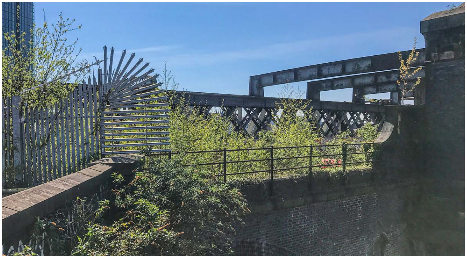
Photo of existing, inadequate guarding
