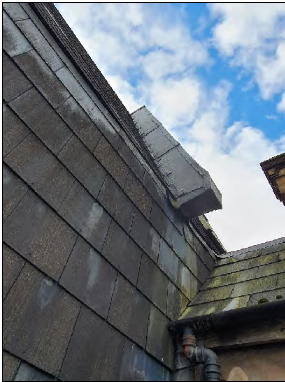
Photo 7 Another example of loosely fixed flashing creating PRF
