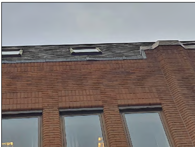
Photo 4 Eastern face showing small vertical mortar gaps above windows as well as raised lead flashing above top bricks
