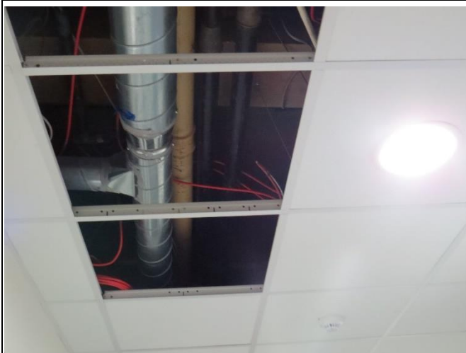
Services Above Suspended Ceiling
