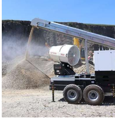
Fig.03 – Typical dust suppression equipment
