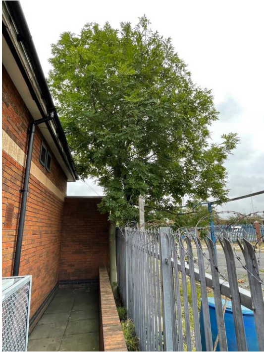
T1 Ash to the rear of the Sales Building impacting on the roof and gutter
