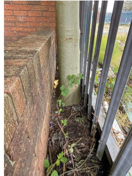
T1 Ash trunk already pressed against the wall and security fence
