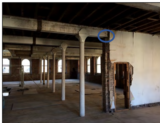
Detail 26: Truncated chamfer and stop detail (circled in blue) at second floor level confirming the brickwork partition to the right-hand side to be a later addition.
