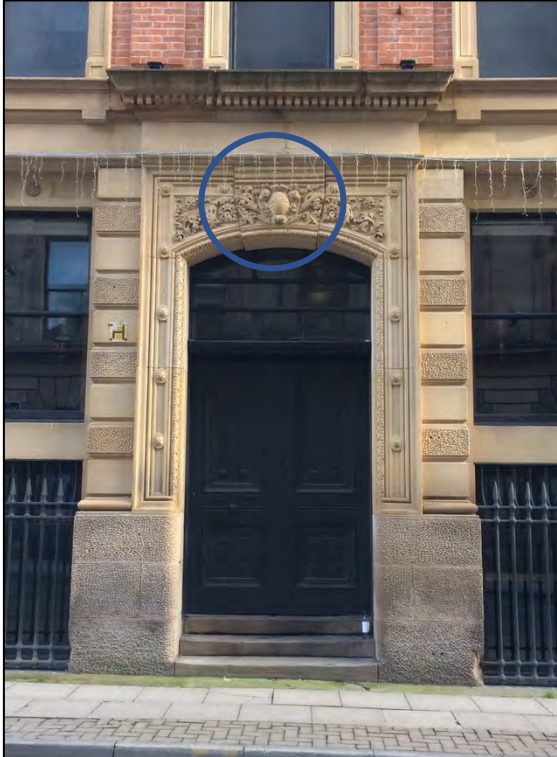
Detail 1: The oversized entrance door of c. 1896 to Southmill Street. This matches the original to Peter Street, itself subsequently lost in the 1963 alterations to the Peter Street elevation. The dropped keystone (circled in blue) is a typical Mannerist detail.
