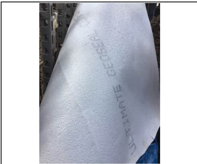
Visqueen Geoseal Ultimate used
