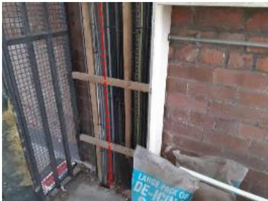
Picture showing cable route to loft space.
