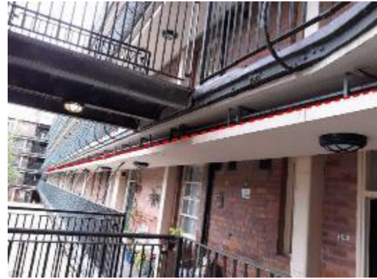
Picture showing typical cable run along tray work.
