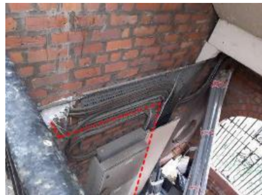
Picture showing cable route to loft space.
