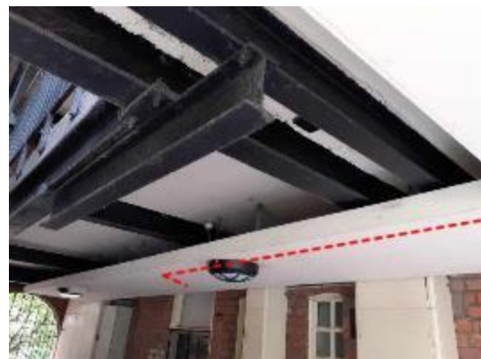
Picture showing connection for apartments.
