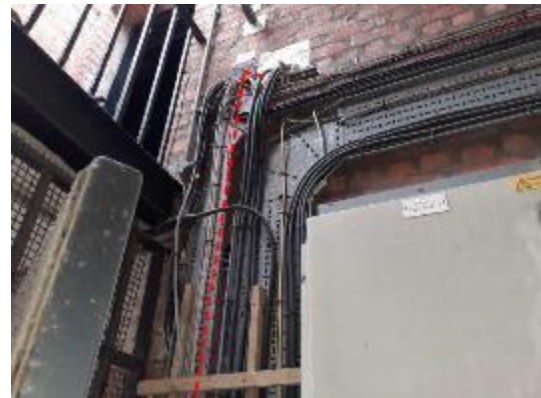
Picture showing cable route to loft space.
