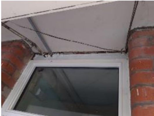
Picture showing fire seal above doors.
