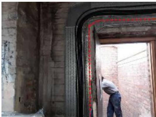
Picture showing cable route to loft space.
