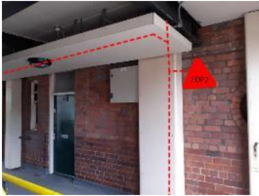
Picture showing cable route from FDP1.
