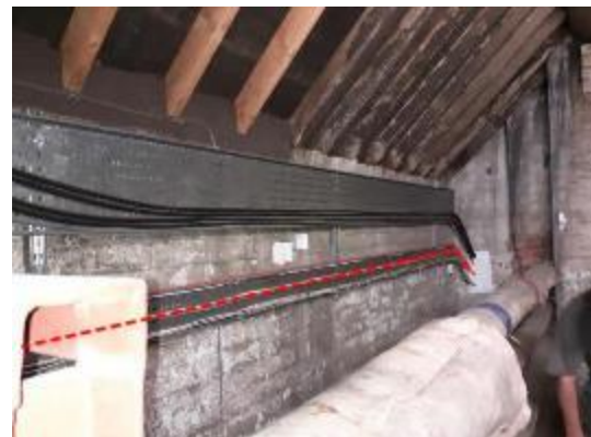
Picture showing cable route to loft space.
