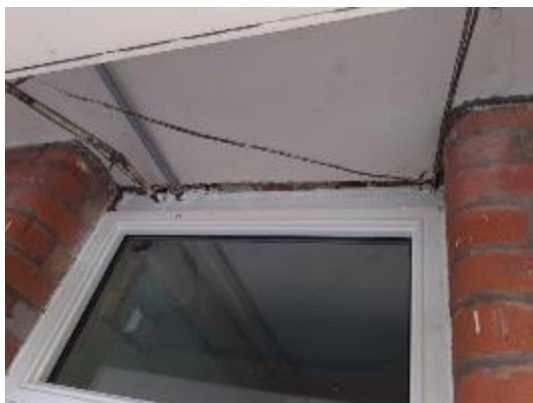
Picture showing fire seal above doors.
