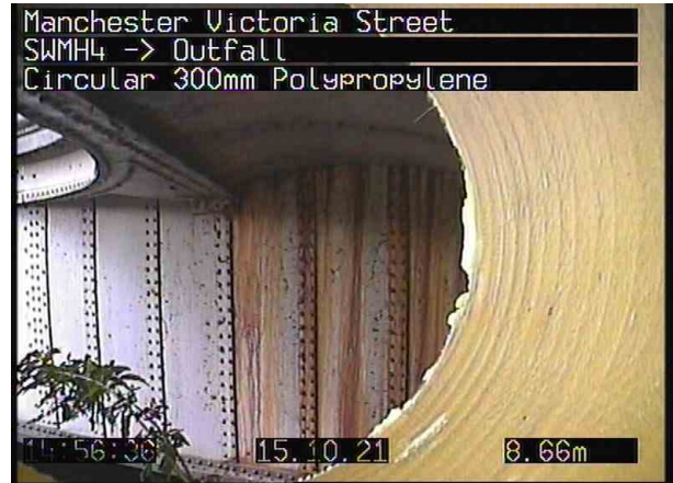
SWMH4X_4fe15750-e136-467e-83f6-88fe7f023eca_20211019_153850_128.jpg, 00:02:27, 8.66 m Point repair, localised lining from 12 o'clock to 12 o'clock, end of patch
