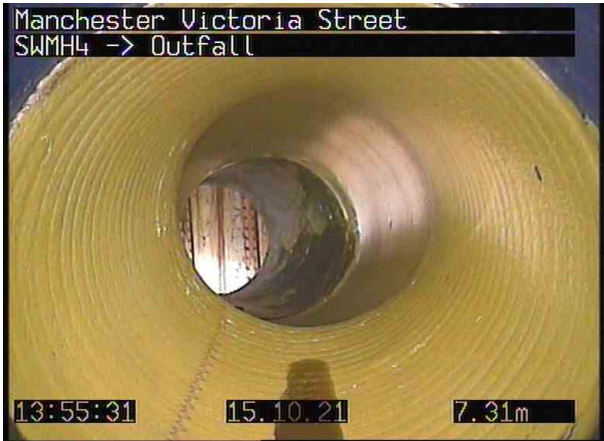
SWMH4X_1efb133e-cbb1-49ba-8a6b-ce4472694a3b_20211019_153845_315.jpg, 00:00:40, 7.36 m Point repair, localised lining from 12 o'clock to 12 o'clock, Start Of Patch
