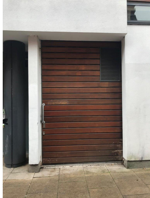
Figure 4: Existing ventilation louvres on William Fairburn Way.
