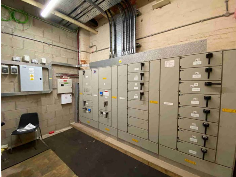
15: Main electrical switchgear
