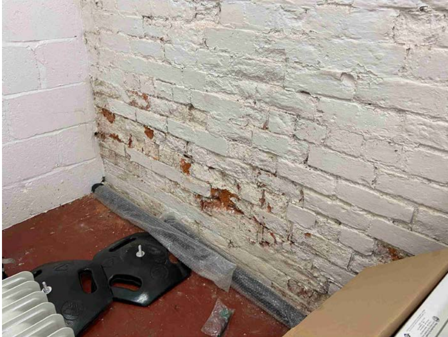
35: Typical water ingress to internal basement walls
