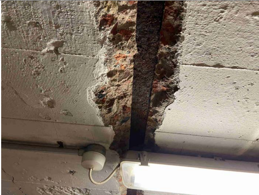
21: Historic corrosion to embedded steelwork to roof plant room
