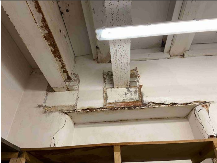
37: Typical water ingress at basement at high level Peter Street elevation
