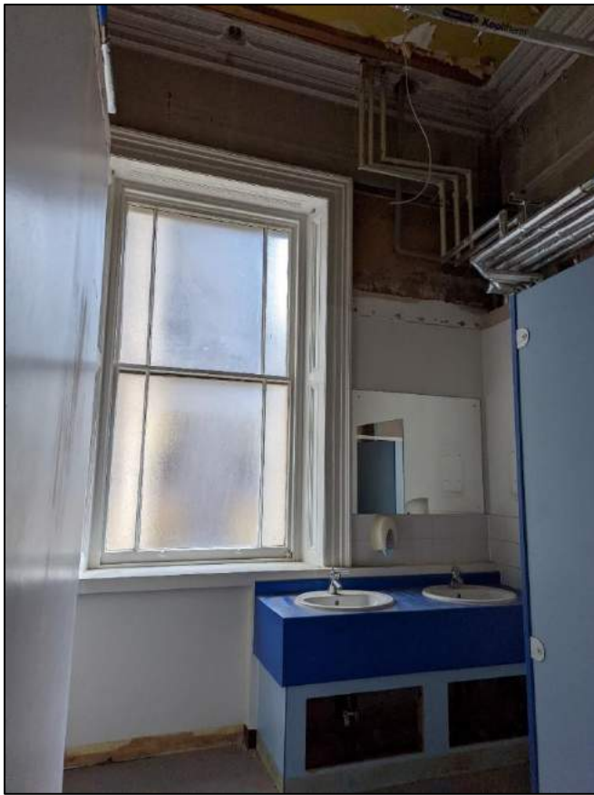
Plate 74: WC off corridor above showing cornice
