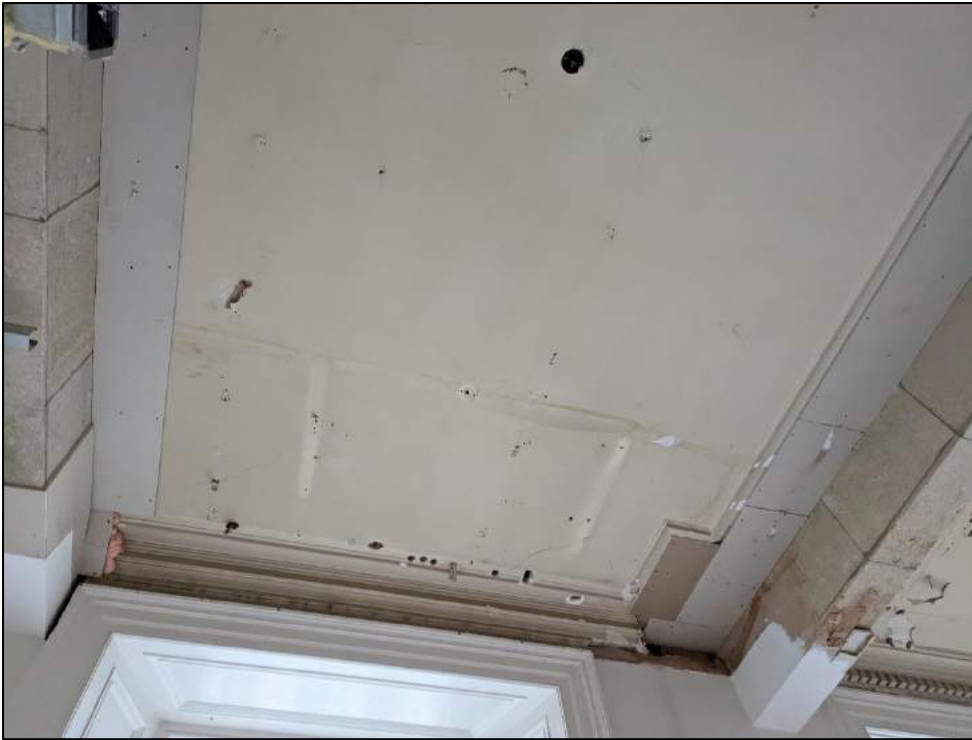
Plate 66: Detail of damaged cornice
