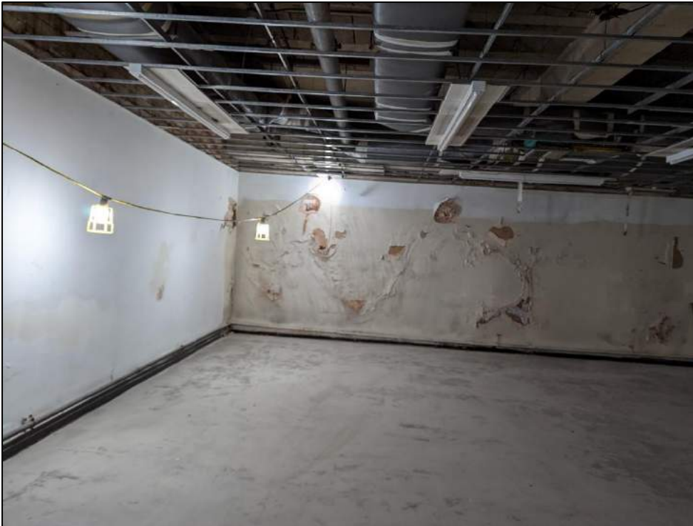
Plate 112: As above showing decaying plasterwork
