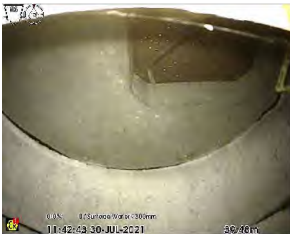
MH01 US LINE A_39-48m_114243.jpg, 00:04:21, 39.48 m Finish node type, manhole, reference number: LINE A, MH02
