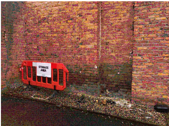
5. Staining to brickwork. Brickwork to be cleaned with a steam cleaner. Brickwork to be repointed if necessary. Mortar to match existing.
