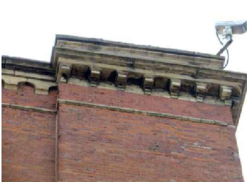
1. Damaged edge to string course. Stone repair required.
