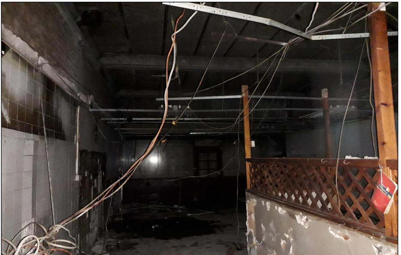
View of Café Unit 20 – Internally it is in a very dilapidated condition.
