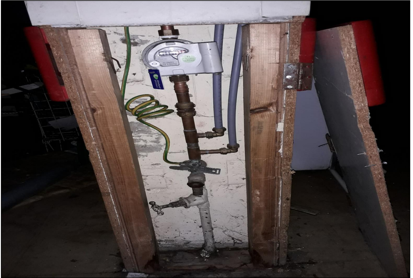
View of rising C.W. Supply and water meter within loading bay area to Unit 18.
