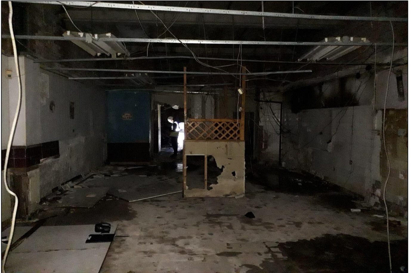
View of Café Unit 20 – Internally it is in a very dilapidated condition.
