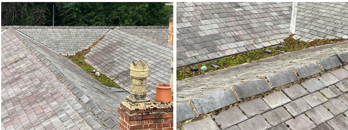
Condition of the hidden valley gutter August 2021 – Note the moss and debris retaining water run off and obstructing central outlet.
