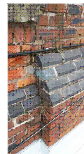
8 Vegetation growth in mortar joints requiring removal
