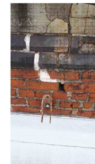
5 Deterioration to front parapet requires repointing
