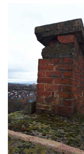
10 Southern corner showing missing brickwork to outer leaf. Missing bricks to be replaced.
