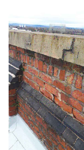
13 Weathered brickwork to rear elevation, record photo
