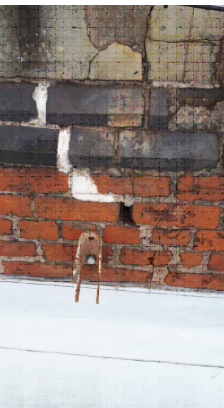
5 Deterioration to front parapet requires repointing
