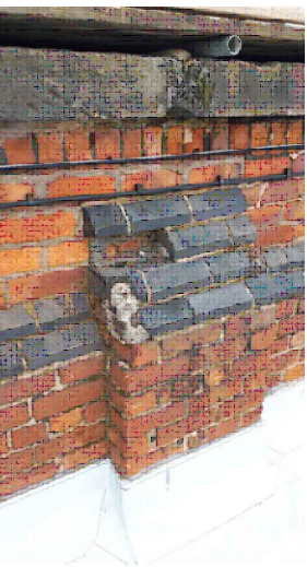
6 Missing cant brick requires replacement
