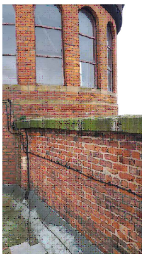
9 Steel restraint straps and cracking brickwork on northern corner requires replacement brickwork and repointing
