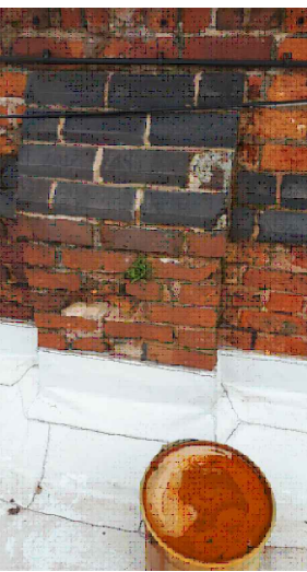
7 Spalling mortar to front parapet requiring repointing and vegetation growth requiring removal
