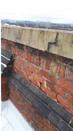
13 Weathered brickwork to rear elevation, record photo
