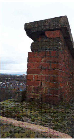
10 Southern corner showing missing brickwork to outer leaf. Missing bricks to be replaced.
