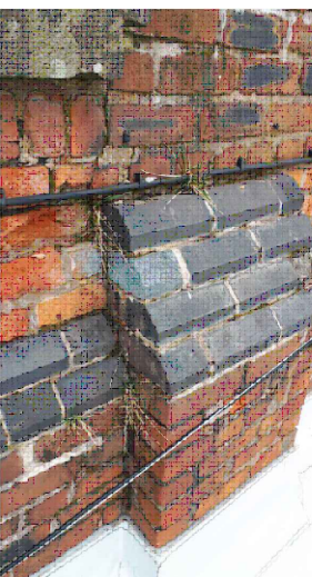
8 Vegetation growth in mortar joints requiring removal
