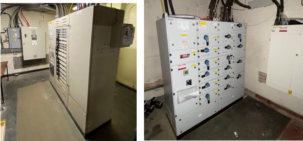
Figure 3.3: Spring Gardens Main LV Switchboard (left) and Mosley Street LV Switchboard (right)
