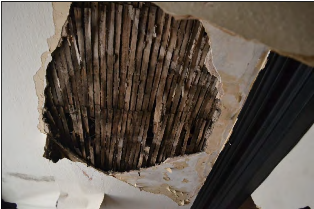
Photograph 116: Detailed view of structural damage to ground floor ceiling
