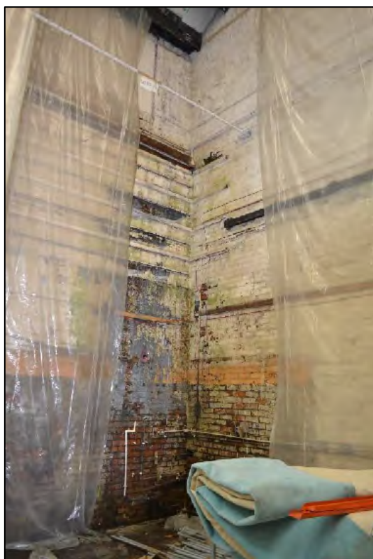
Photograph 73: General view of corner between C2 and C1 showing water damage
