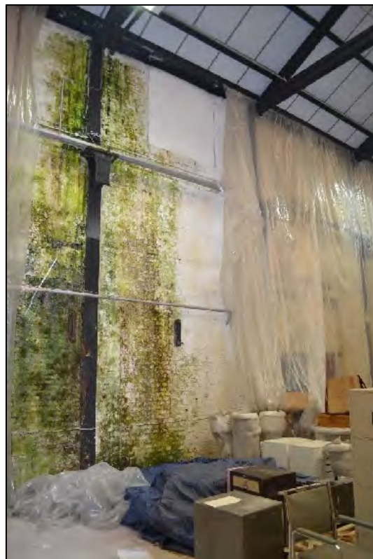
Photograph 68: Detailed view of eastern wall of C2 showing water damage around cast iron column
