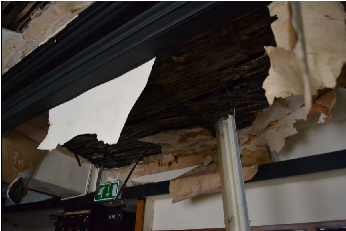
Photograph 117: Detailed view of structural damage to ground floor ceiling
