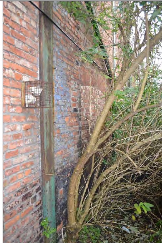
Photograph 26: Detailed view of one of the bricked-up and overgrown former apertures along the north-eastern elevation
