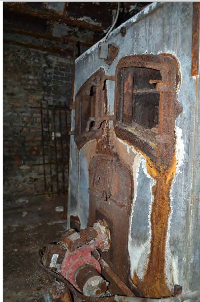
Photograph 102: View of the boiler within D3
