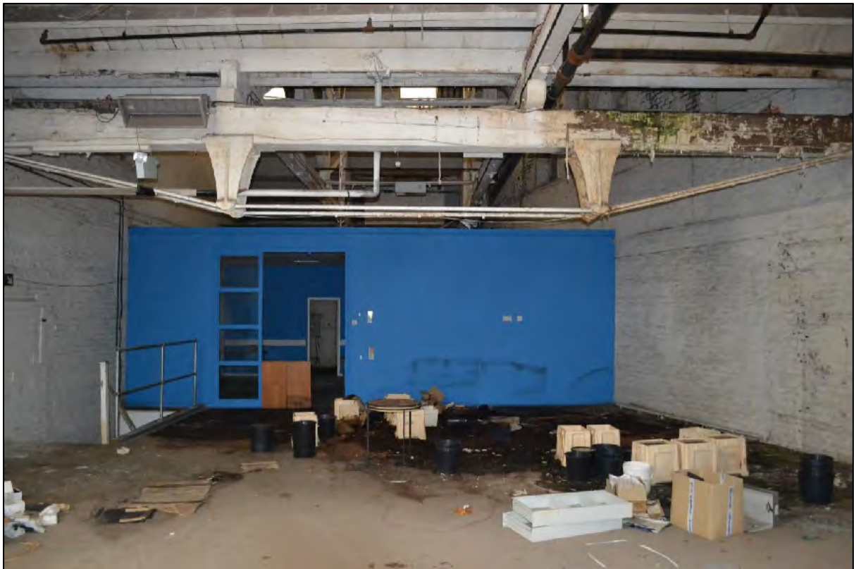
Photograph 63: View north-east from first floor doorway between Structures A and B. Note water damage to floor
