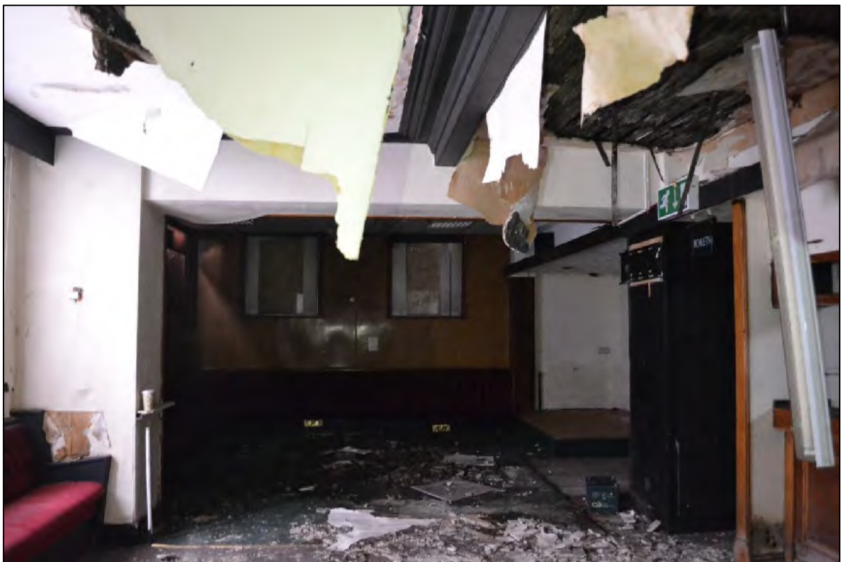
Photograph 114: View north within ground floor of Public House showing structural damage
