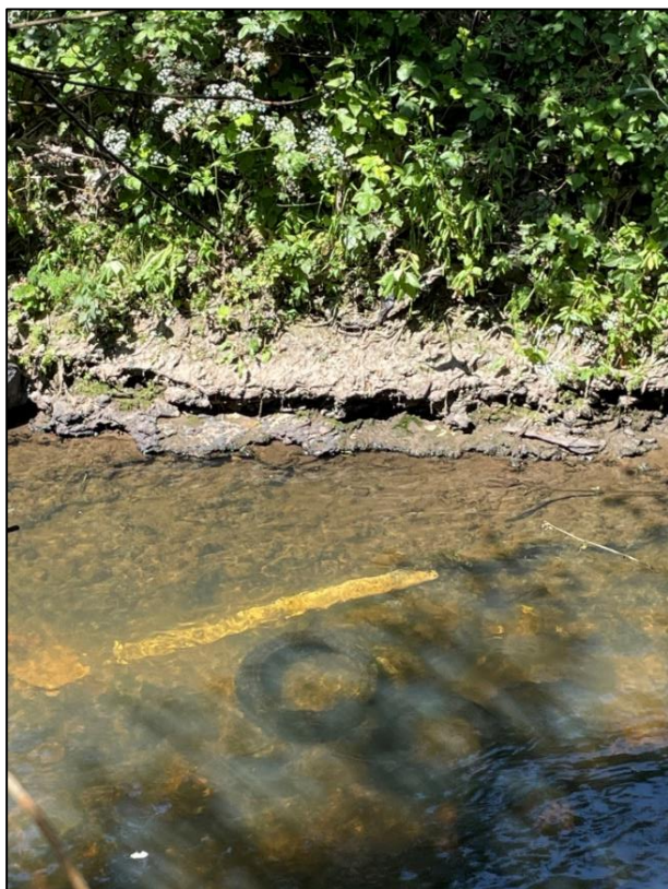
Figure 17: Across-channel view of Reach 4 showing erosion of berm on right bank side.
