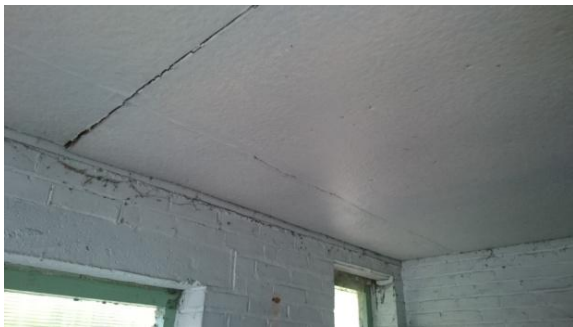
Photograph 3 Gap in ceiling panel of garage
