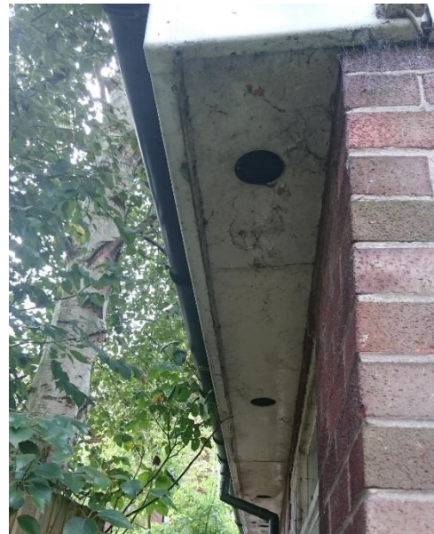
Photograph 6 Showing series of large holes within the plastic and asbestos soffit box on the western side of the house.
