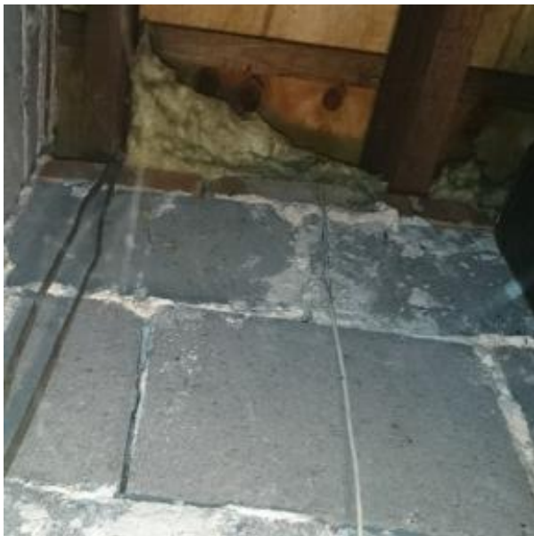
Photograph 5 Inside small loft void showing the unlined roof and exposure of cavity wall insulation.
