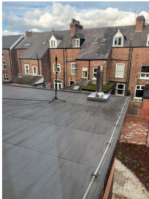
Figure 7 - location of boiler flue.
