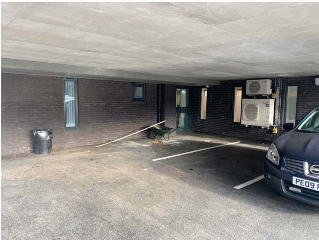
Figure 6 - A/C condenser location relative to Flat 4 window.
