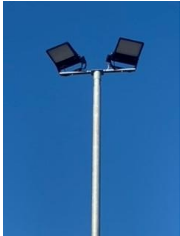
Double Lighting Column
