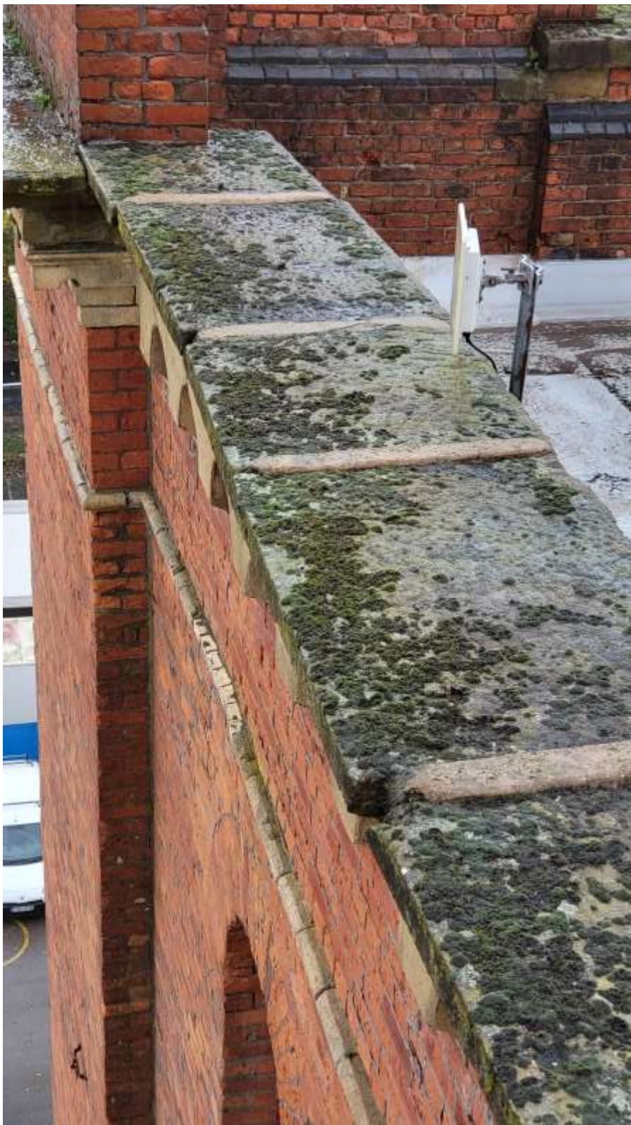
1: North West Elevation: Damage to edge of coping stone
