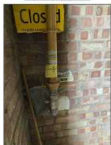
GAS ISOLATION POINT
