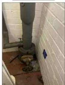
MAINS COLD WATER ISOLATION POINT
