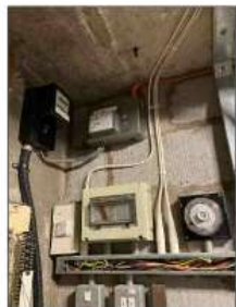
MAINS ISOLATION POINT
