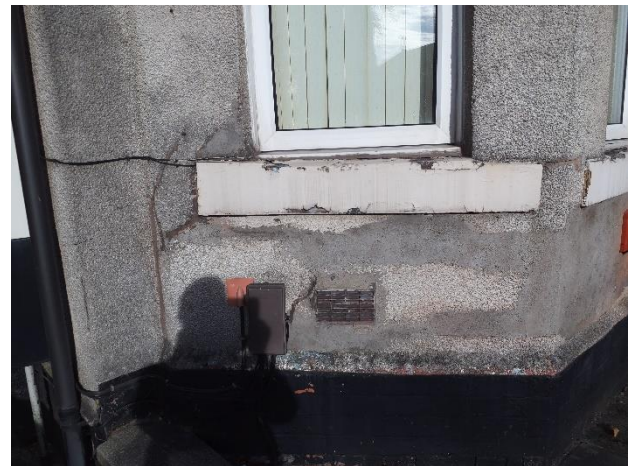
Figure 04: General condition of defective render
