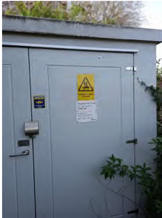
Photo 15: Electricity sub station located to the south west of Site D.
