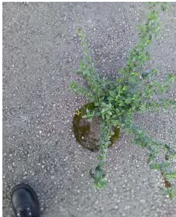
Photo 8: Asphalt surface and previous borehole location with vegetation growing in crack, within Site D.
