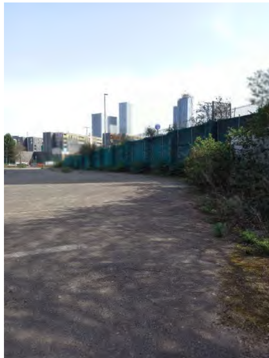
Photo 16: Brick Retaining wall running adjacent to the Regent Road Bridge, covered with netting due to reasonably poor quality of the brick surface.
