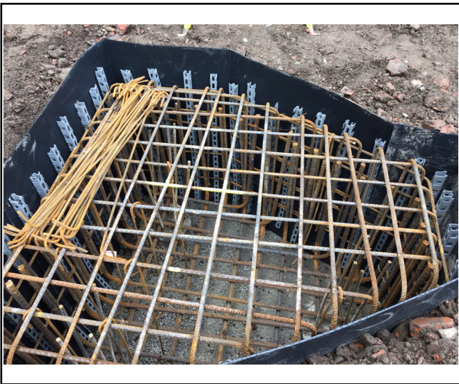
One of the pile caps did not need
