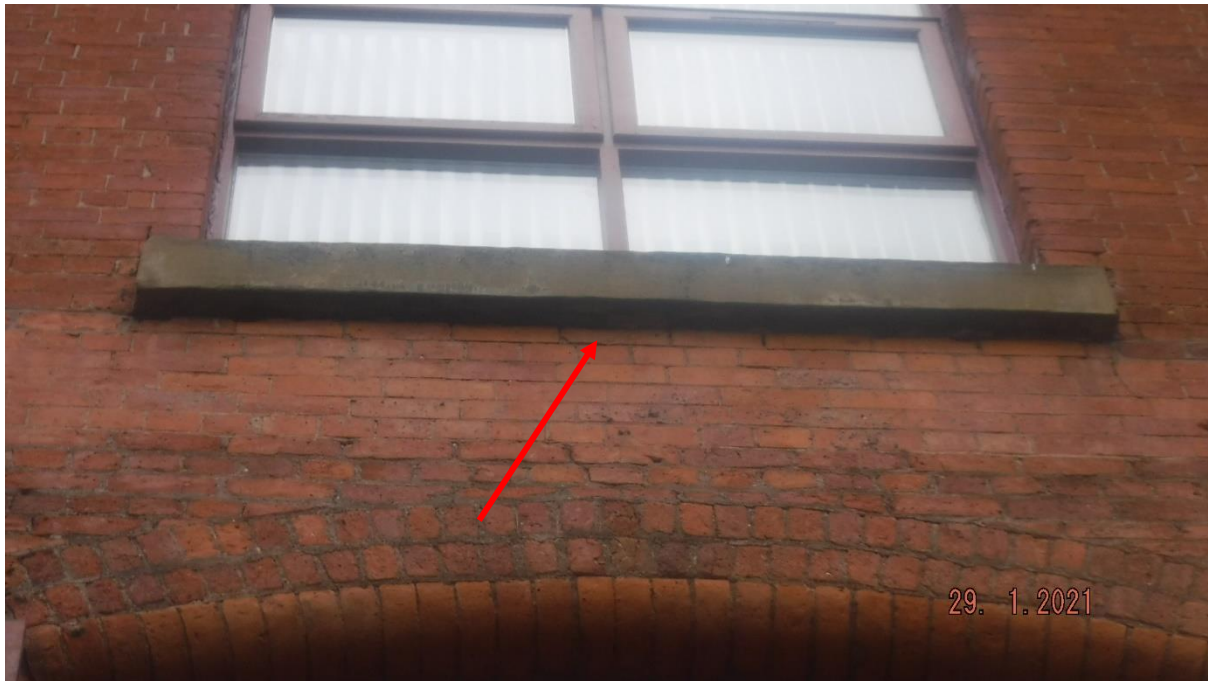
Photo 5. Location of Roost 2 on the south-western aspect of Victoria Mill, beneath a window lintel.
