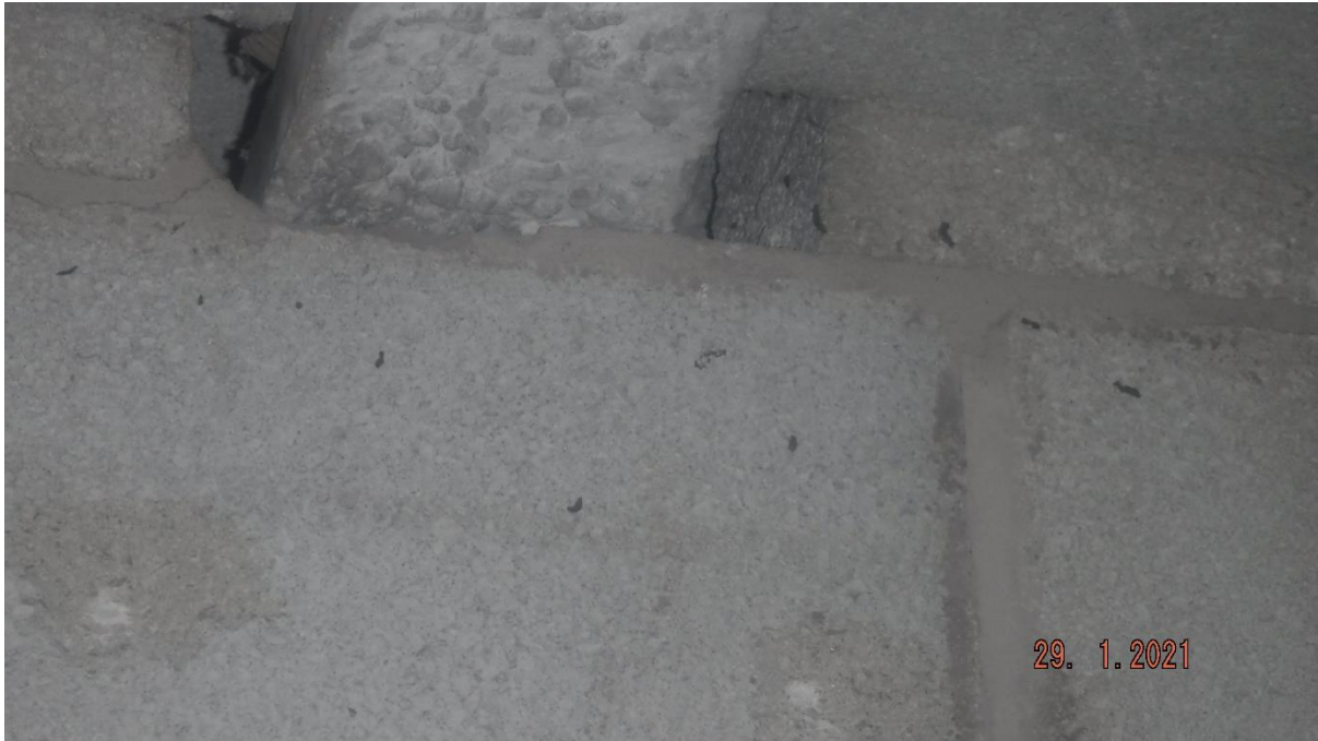
Photo 9. Scattered droppings present at the top of a breezeblock wall, consistent with the location of droppings during the hibernation surveys in 2016/2017.
