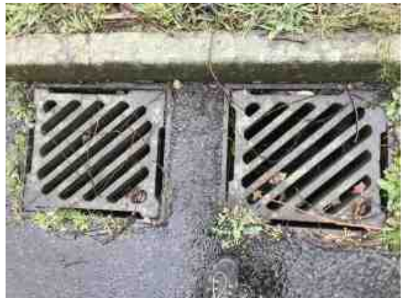
Photograph 5 (P5) Gullies present within the south of the site.
